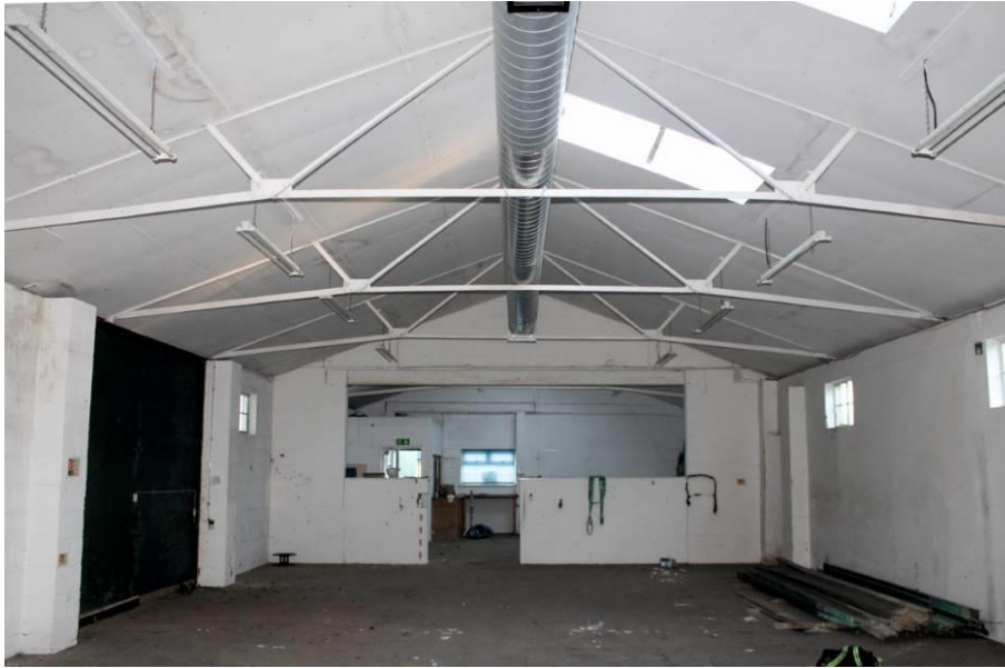
Plate 19: Building C, room C1 showing roof structure and partition. Looking south east.
