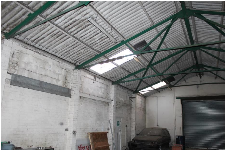
Plate 12: Building A, showing blocked windows and RSJ in roof structure. Looking west
