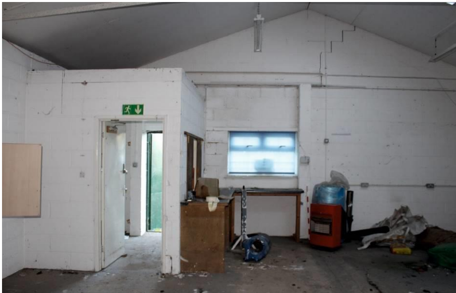
Plate 22: Building C, room C1 showing partition C5 and blocked entrance. Looking south east.
