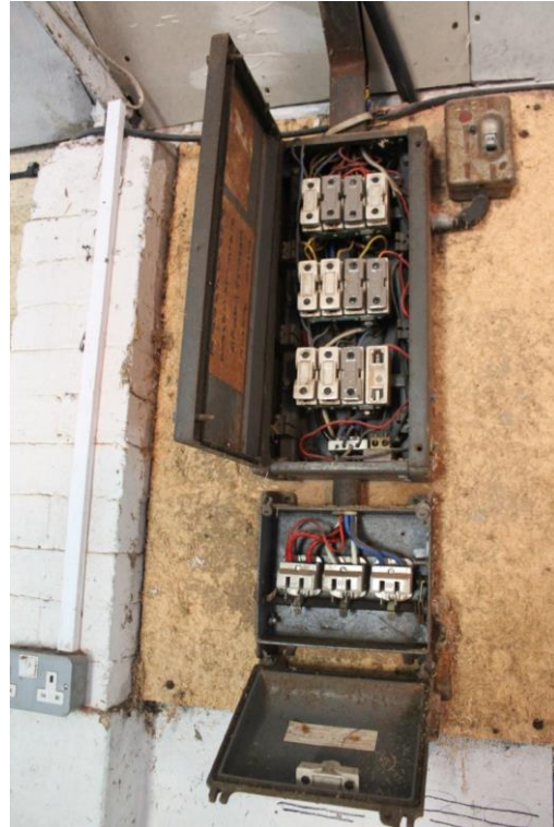
Plate 27: Room G1; northern wall with historic fuse box and switches. Looking north
