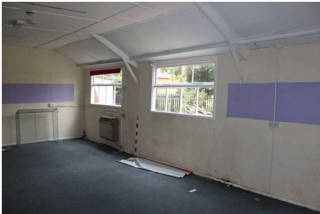
Plate 18: Room 17, showing windows and leaning wall. Looking south west.
