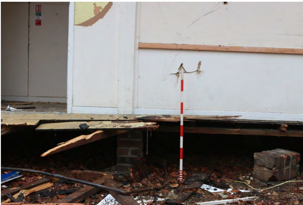
Plate 7: Mid-demolition, showing brick pad and supporting beam under eastern block. Looking east.
