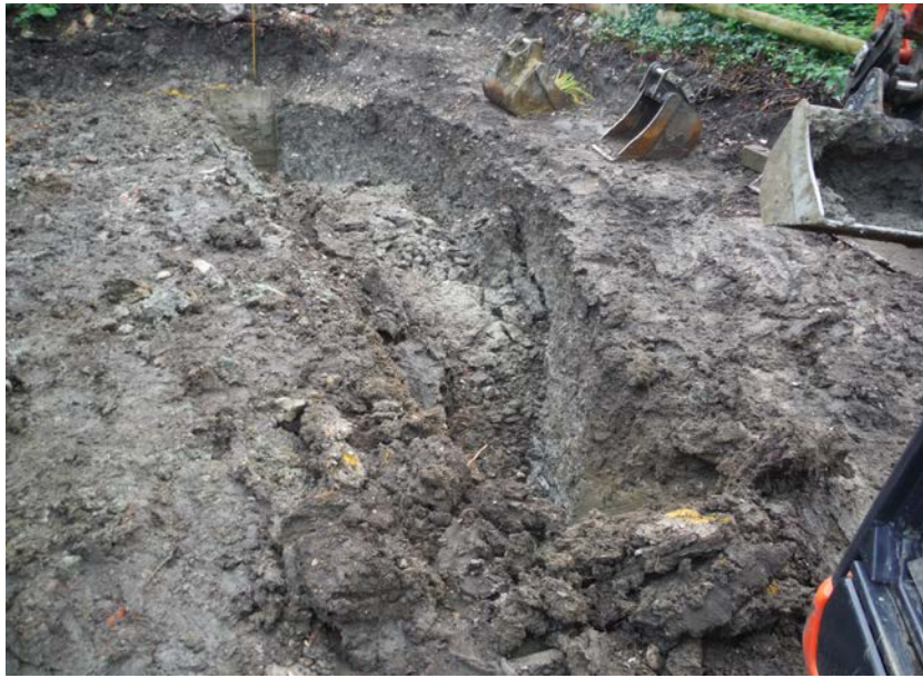
Plate 1: Collapse of south/south-west footing. Looking south-east.
