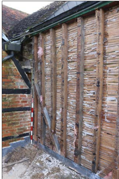
Plate 26. Framework of the north east wall, showing junction with the earlier structure
