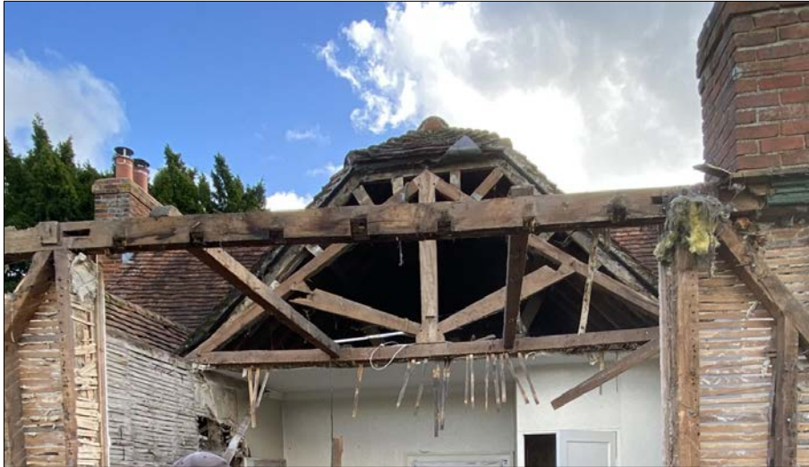
Plate 33. King post truss inserted within the gable of the earlier building's half-hipped roof
