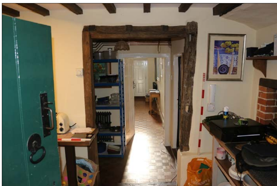
Plate 12. South eastern wall of Room G1; the scale bar is resting on the plinth
