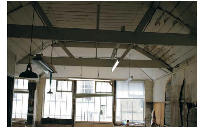
Plate 8. The roof space of No. 32 showing the tie beams and Queen Beam supports (cross-section G)
