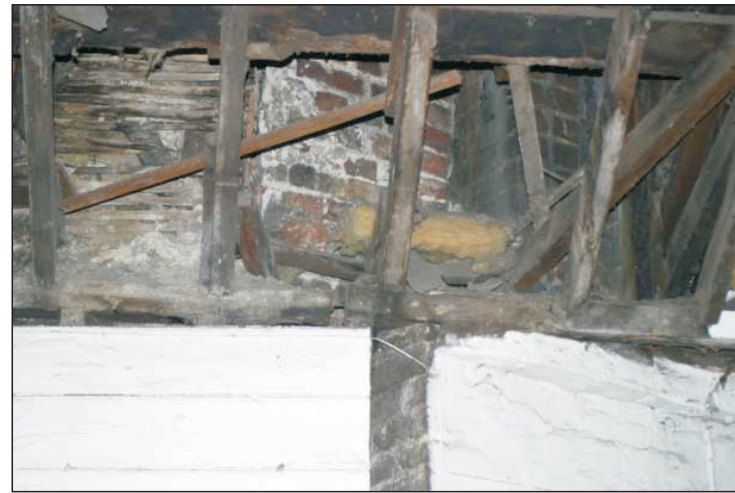
Plate 6. The lathe covered wall and brickwork of No. 32& 34 St Michael's Street evident in the roof space of No. 32 (wall C)
