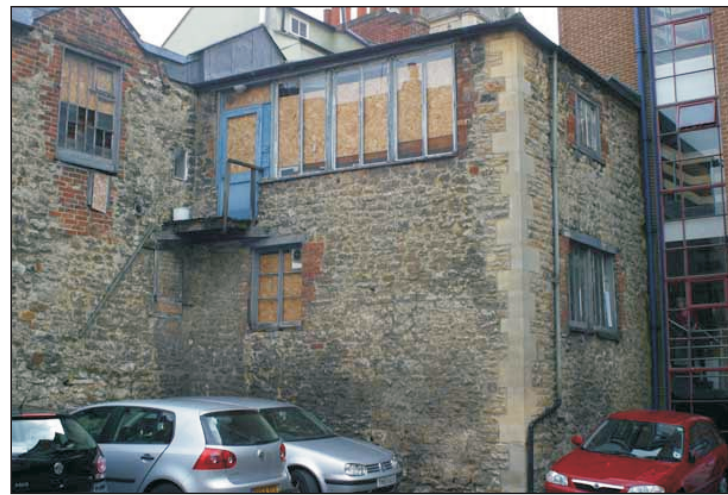
Plate 2. General view of Bastion 2 rear of 32 St Michael's Street (walls A & B)
