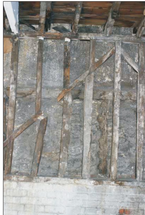
Plate 4. The west wall of No. 32 St Michael's Street showing the wooden frame to support boarding at No. 32's wall and also the timber frame wall onto which it is built of No. 34 (wall C)
