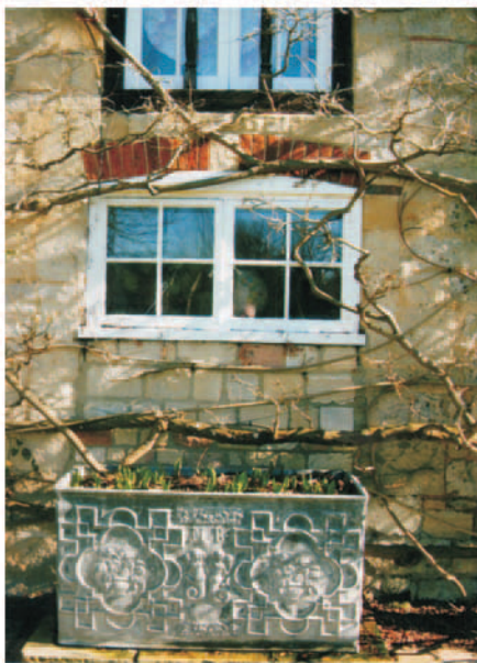
13. Blocked door with hayloft doorway above. Note two straight joints below window and blocking behind lead cistern
