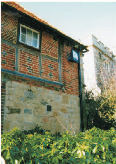
4. North end of east wall. Note fine ashlar stone blocks in lower part of wall.
