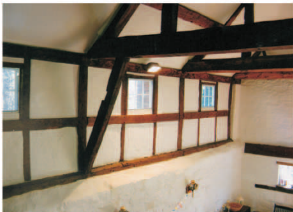
27. East wall from inside. Note thick masonry wall. Also tie beam with brace supporting it.
