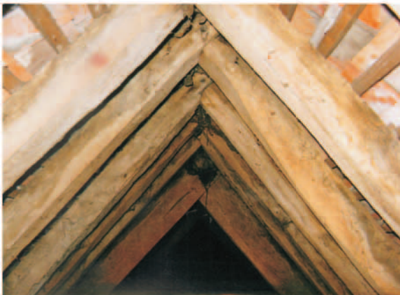
31. Common rafters at apex of roof. Note halving and pegging and absence of ridge piece.
