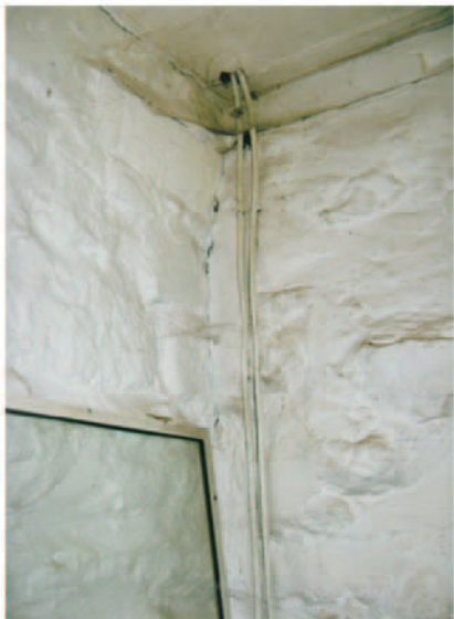
41. Detail of lateral wall (on right), east wall on left. Note crack.
