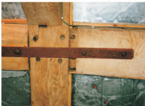
34. Iron strap nailed across principal rafter and purlins which are pulling away
