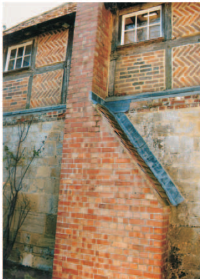
5. Chimney added to east front. Note Fletton bricks. Also ashlar masonry of lower part of east wall
