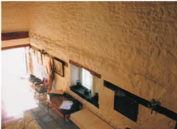
25. Inside of west wall showing where the wall has been raised. Note timber bonds.
