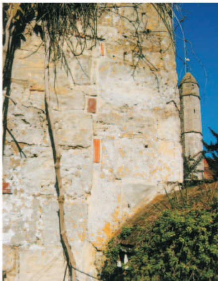
8. End of east wall. Note straight joint indicating that building went further to south
