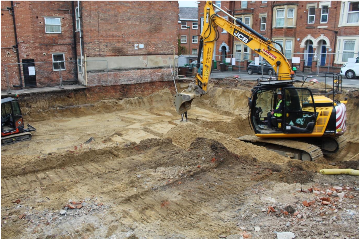
Plate 1. Overview of site during the machine stripping of the overburden. Facing north.
