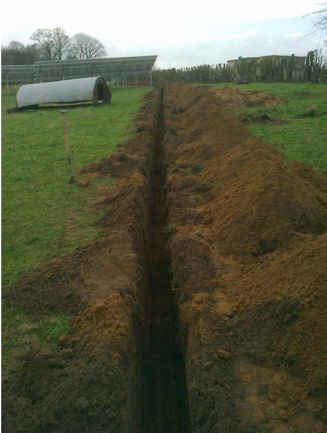
Plate 1: Looking south along cable trench towards solar photovoltaic array
