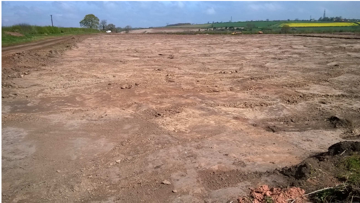
Plate 2: Stripped surface, area to the south of Golden Hill Lane, looking north
