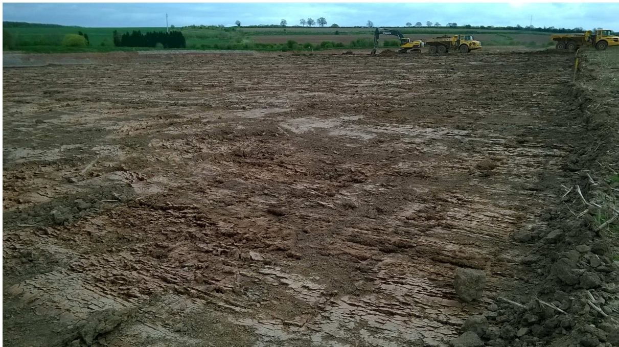
Plate 3: The area to the north of Golden Hill Lane, looking south, during completion of topsoil stripping, 22 April 2015
