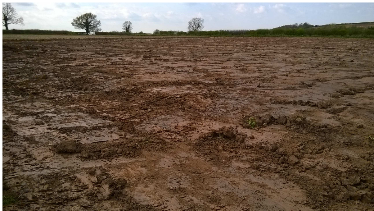
Plate 4: The stripped surface of the area to the north of Golden Hill Lane, looking north-west, 22 April 2015
