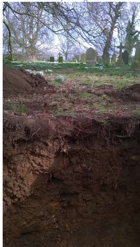
27: Part of west-facing side of 1.10m-deep pit for the soakaway, looking east
