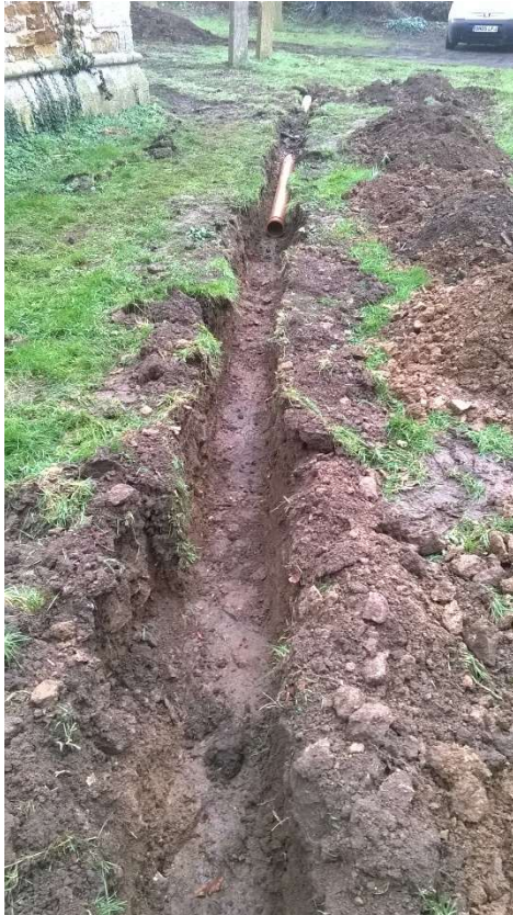
24: Pipe partially laid for main drain across west end of church, looking south-east
