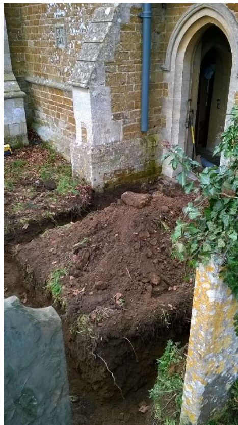
9: Trench for drain from gully below downpipe from organ chamber gutter, looking north-west
