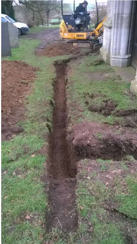
13: The trench for the main drain passing south of the porch, looking west
