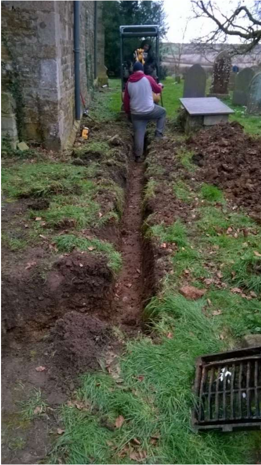
10: The trench for the main drain along the north side of the chancel and nave, looking west
