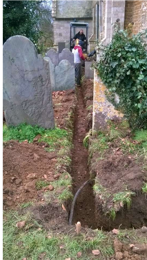
8: Trench for main drain along the side of the aisle, looking west
