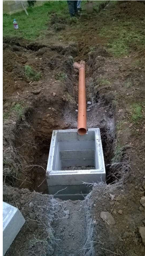
25: Partly installed concrete-lining of manhole for the silt collection chamber, to north-west of the tower, looking south-east
