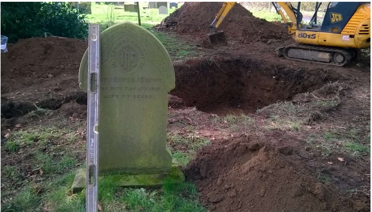
29: North-west facing view of the pit for the soakaway pit, showing its location behind the headstone for the grave of John Edward Brown, died 11th May 1919, and in relation to the slope down to the driveway. The more recent graves in the eastern part of the churchyard are visible in the background beyond the driveway
