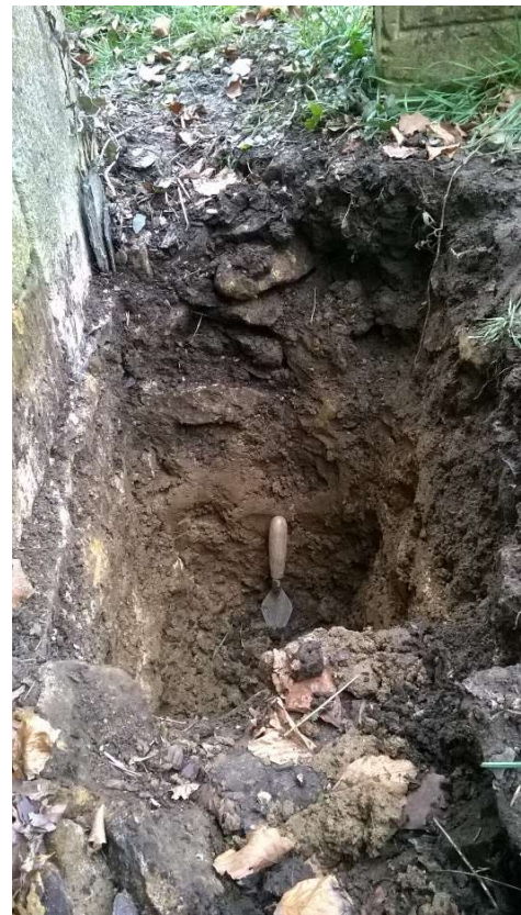
6: Hand-dug pit to take the trap below the corner of the vestry, looking east
