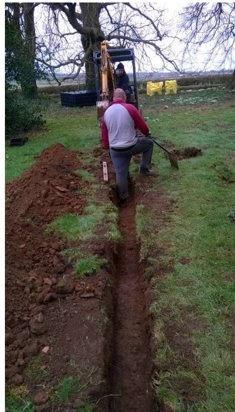
16: The trench for the drain leading to the silt collection chamber and soakaway, looking north
