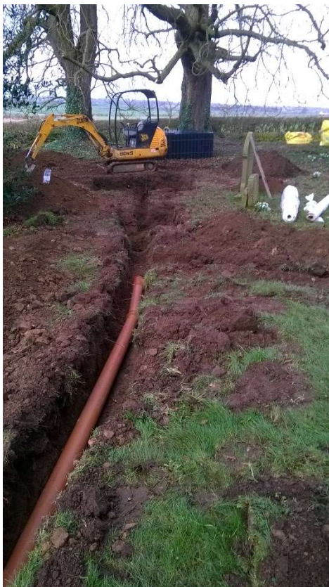
26: View of the trench to the junction of the south and north drains and the excavated pit for the silt collection chamber and main soakaway beyond
