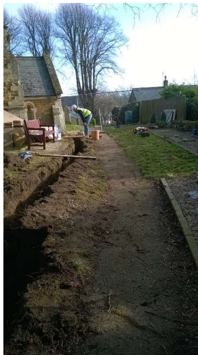
33: The drain to the south-west soakaway running along the north side of the path, looking east
