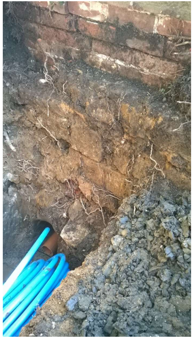
40: Another view of the back of the churchyard wall, showing how the brickwork was added to the front of the earlier stonework, looking north-east
