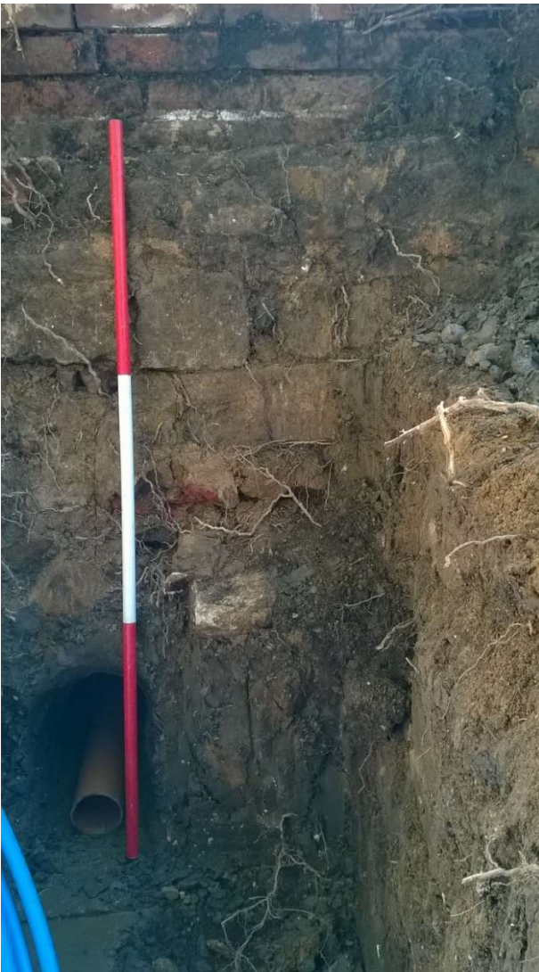
39: The back of the churchyard retaining wall, as seen in the pit to bring the waterpipe onto the site from the main on Main Street (scale = 1500mm)
