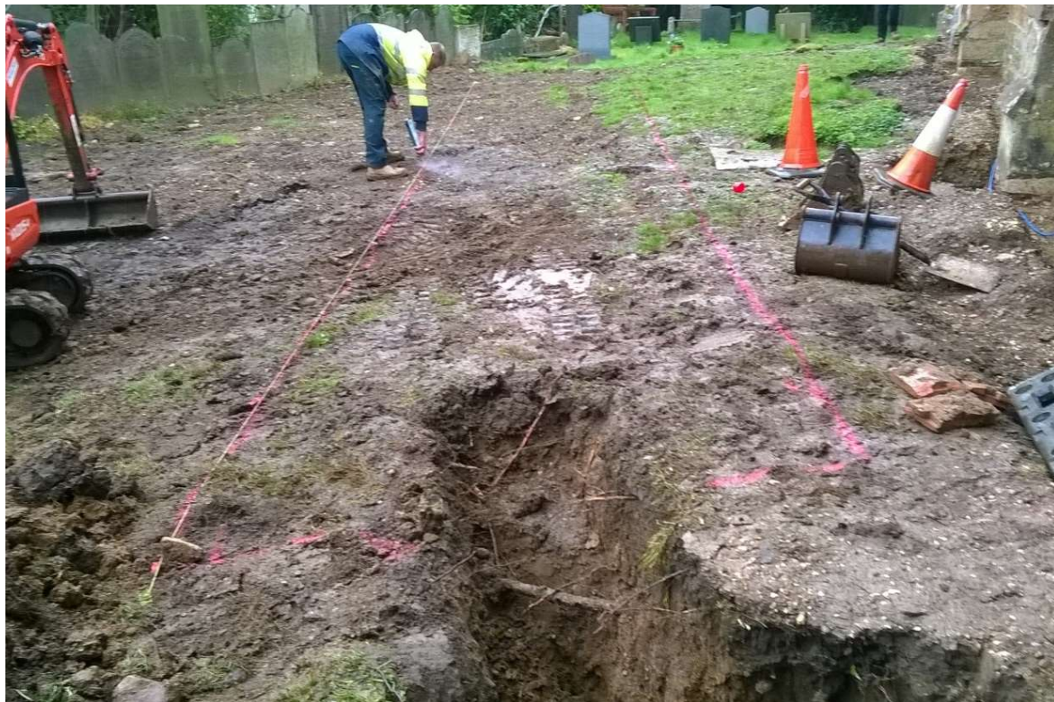
20: Marking out the extent of the trench arch drain, showing its location in the churchyard and the where the electricity cable to the end of the nave crosses at its west end, looking east
