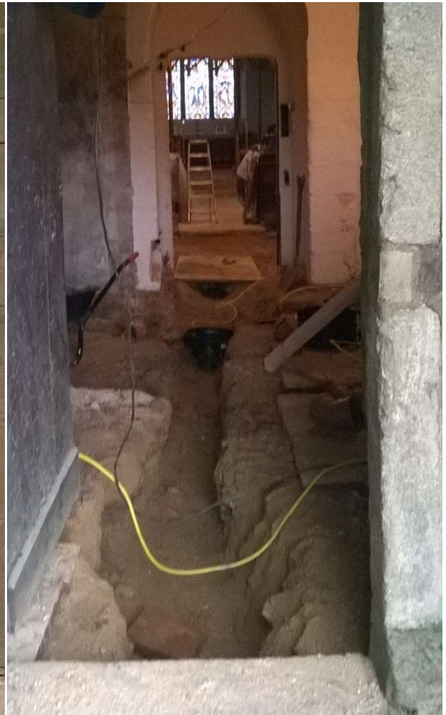
47: View of the tower through the west door, showing excavated service trenches
