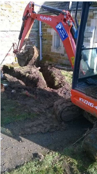
32: Trenches of drains from north-west corners of porch and aisle, looking north-east
