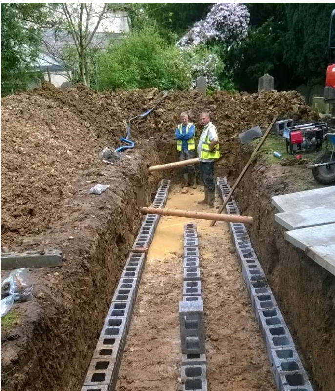
28: Installation of the trench arch drain. The three rows of hollow concrete blocks support a double row of paving slabs leaving a 200mm cavity into which the waste water drains discharge
