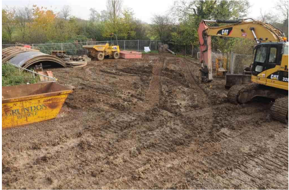
Plate 1: General view of humus tank area after topsoil strip. Camera facing southeast
