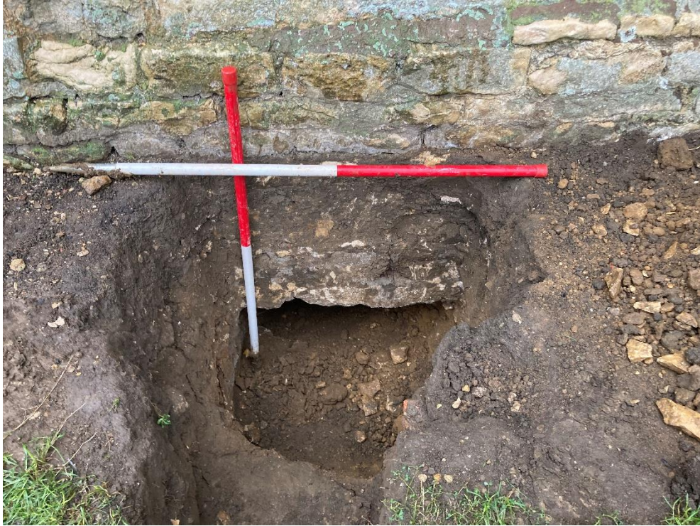
Photograph 5: West wall of north aisle - hole excavated for west pipe, facing east.
