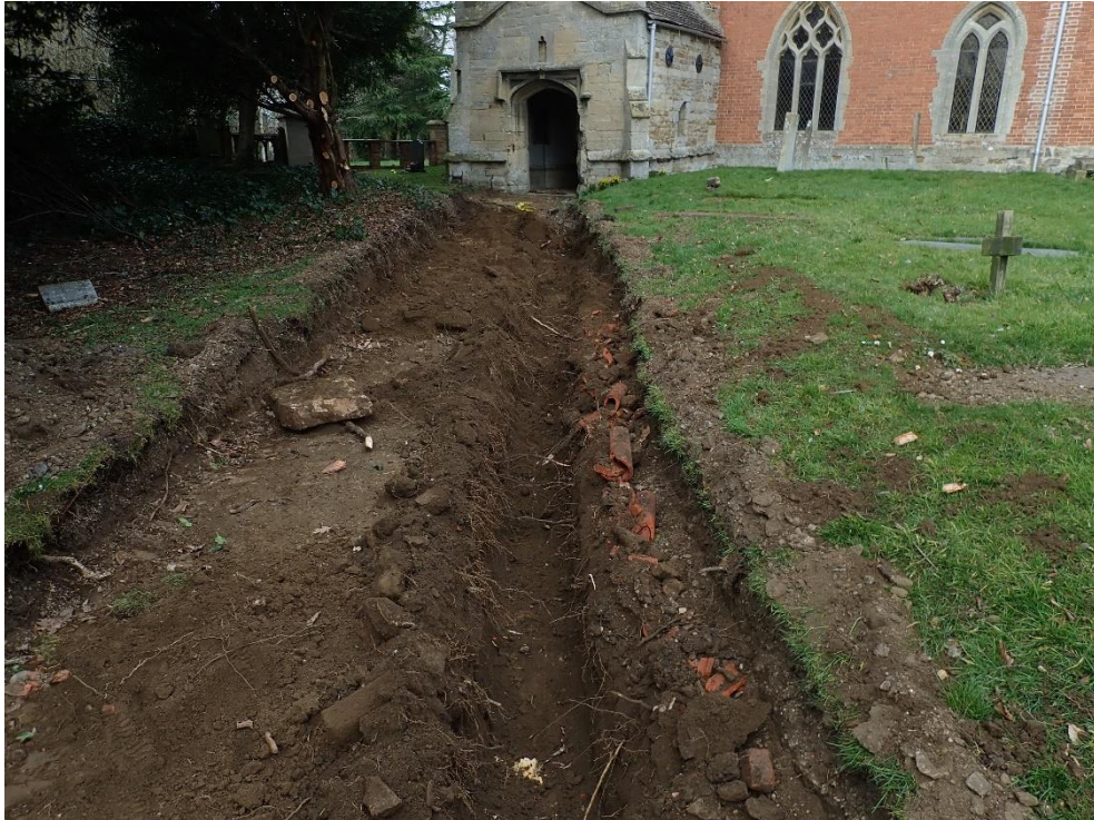
Photograph 8: Stripping of the conduit to the north of the church, facing south
