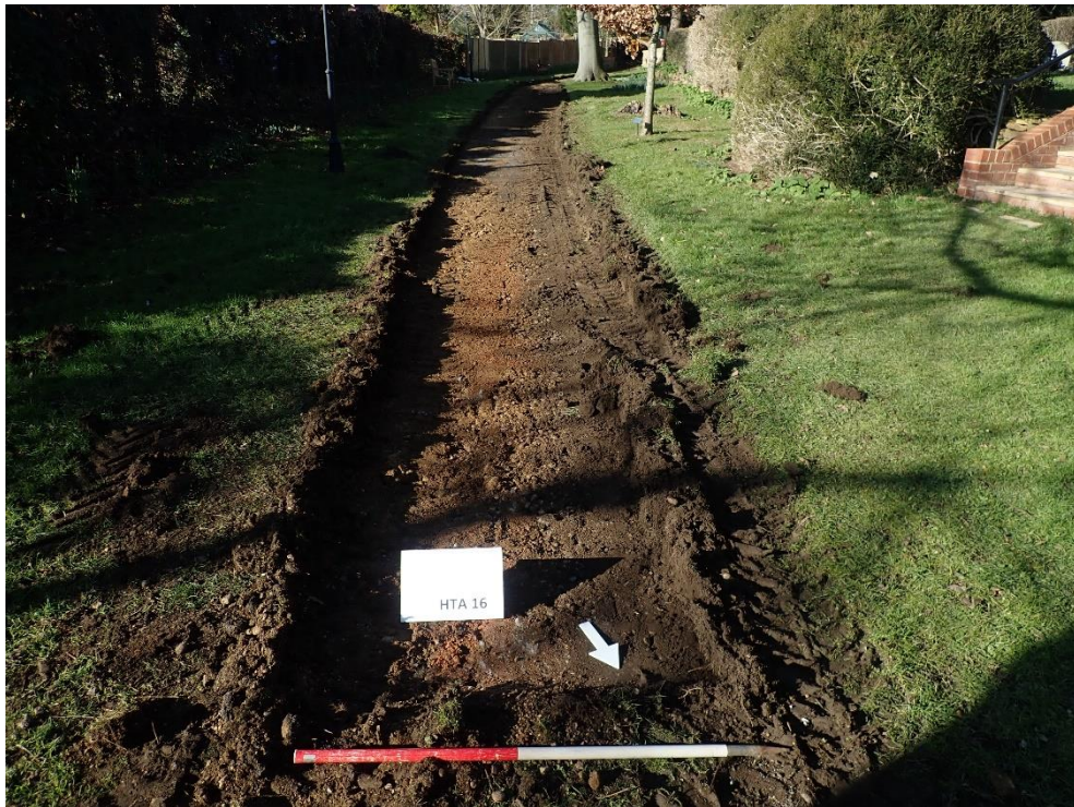
Photograph 6: Stripping of the pathway to the southwest of the main access, facing southwest
