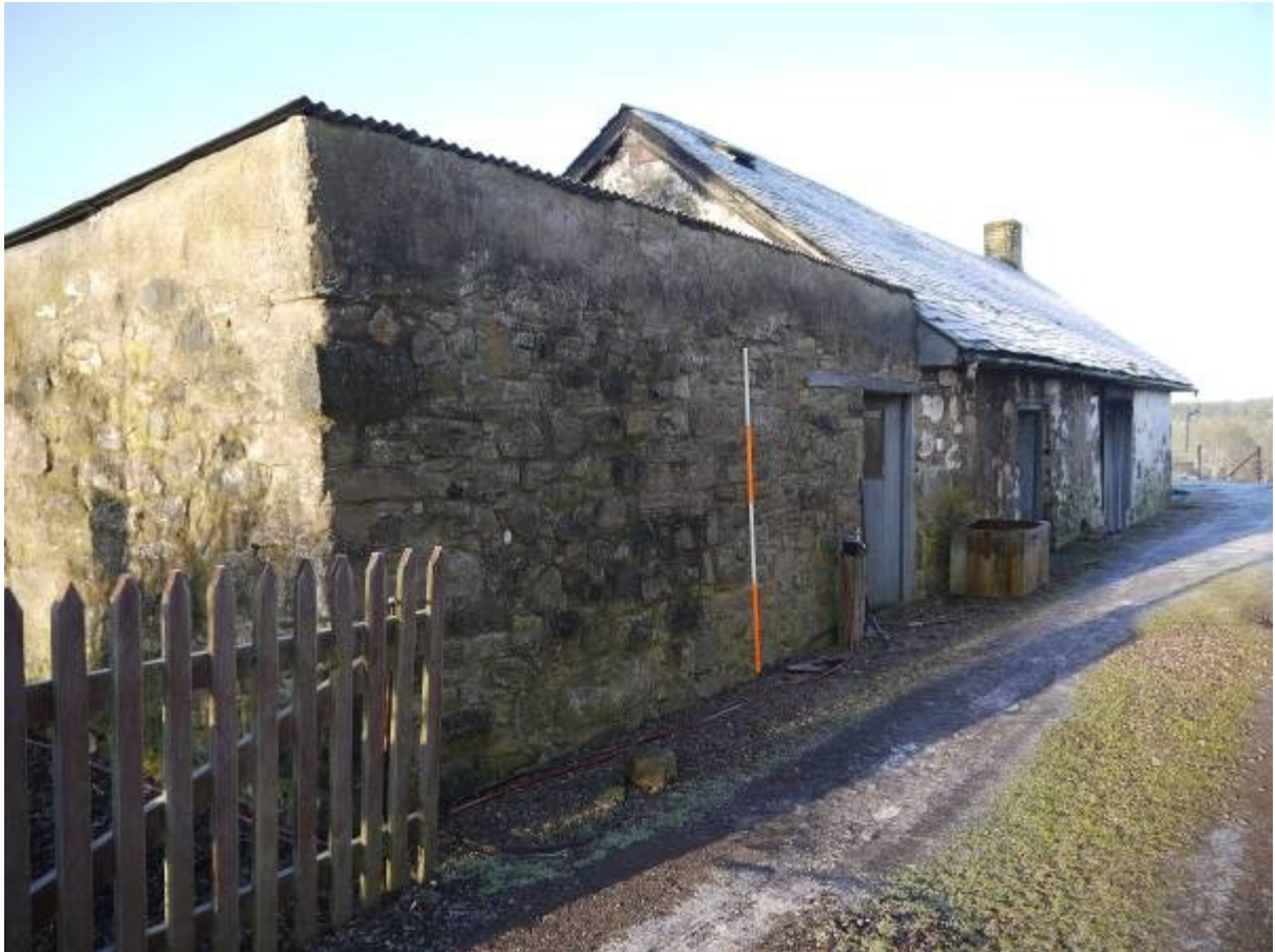
Illustration 8 Northern elevation of Eastern extension (A) showing blocked window (behind scale) and doorway with long wooden lintel
