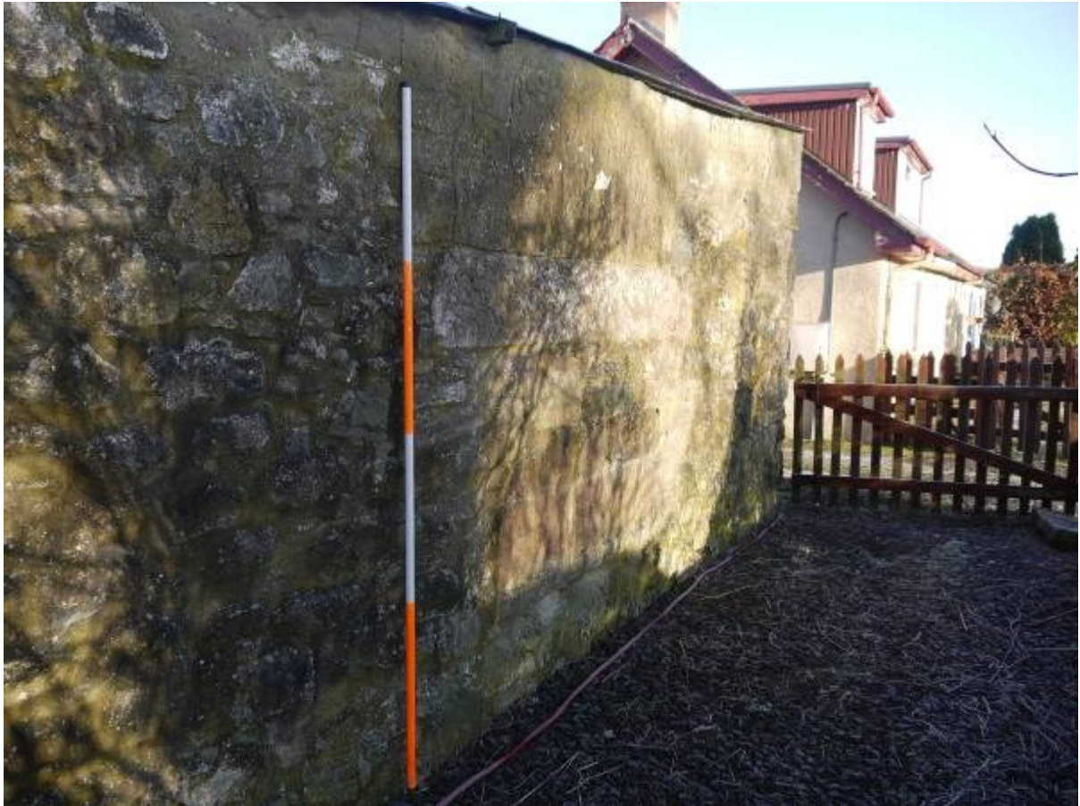
Illustration 6 Eastern elevation of extension (A) showing blocked window/access point with stone lintel to right of scale
