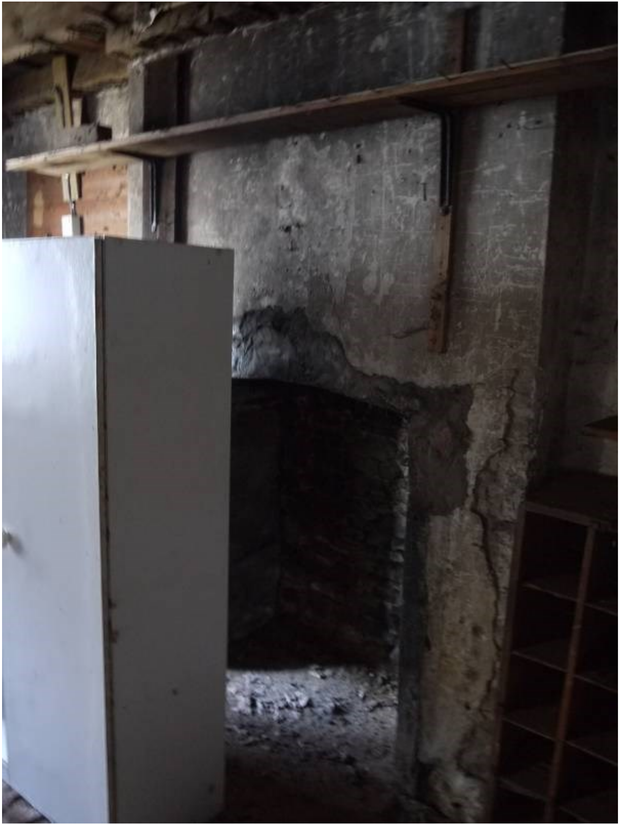
Illustration 20 Flue and chimney base at Western end of western room (C) in main Smithy building
