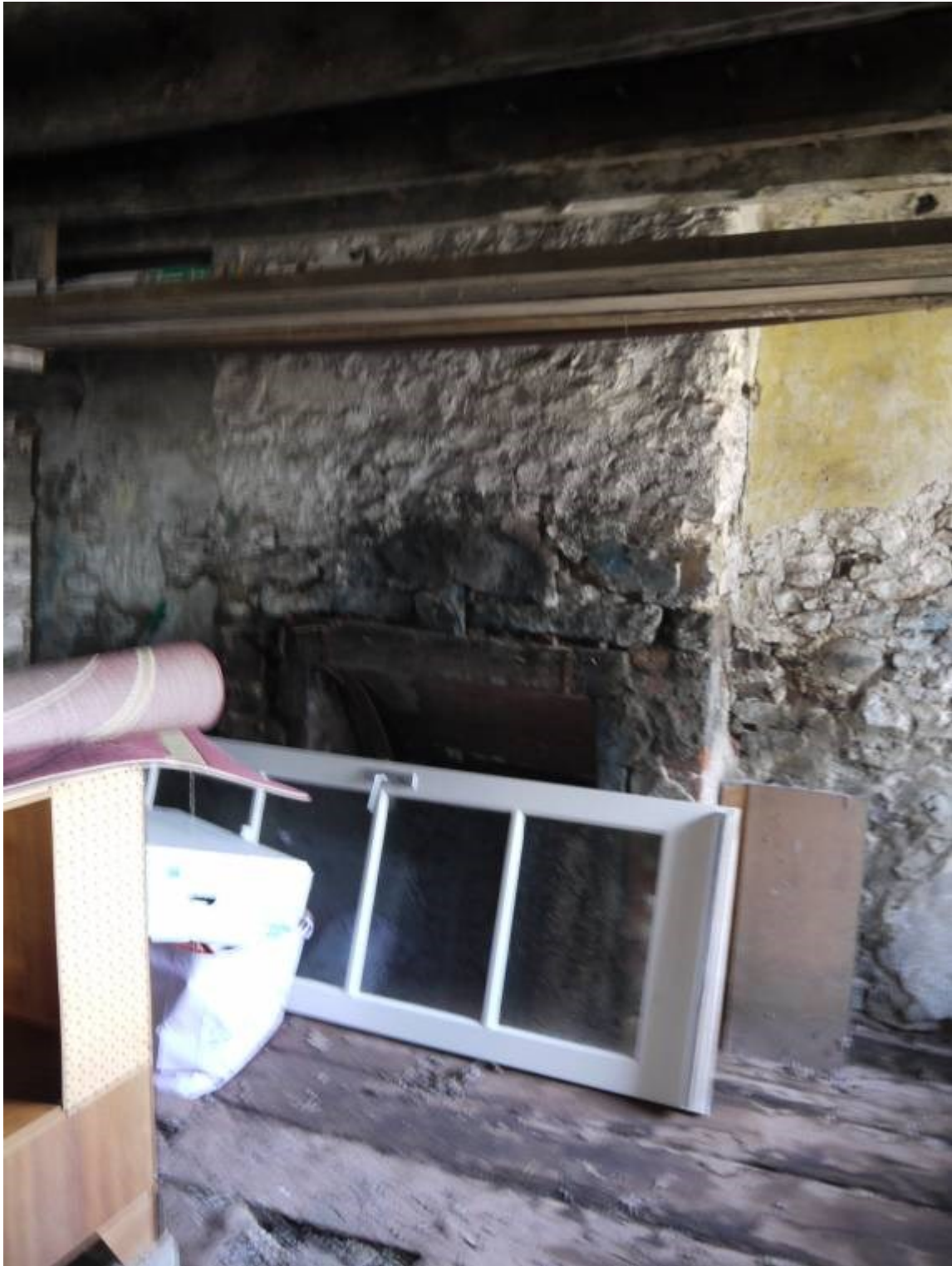
Illustration 21 Flue and chimney base in Eastern elevation of Western room (C) of main Smithy building
