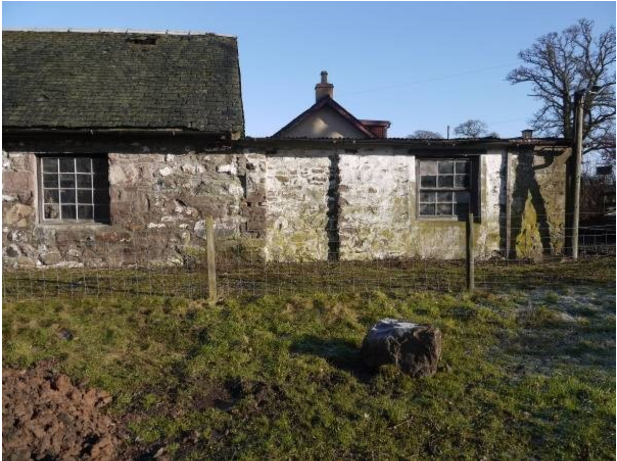
Illustration 7 Southern elevation of Eastern extension (A) showing single window and blocked doorway
