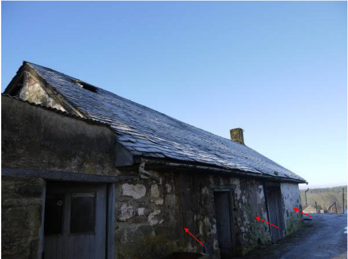
Illustration 11 Northern elevation of main Smithy building (B and C) (red arrows indicate position of blocked slit windows)
