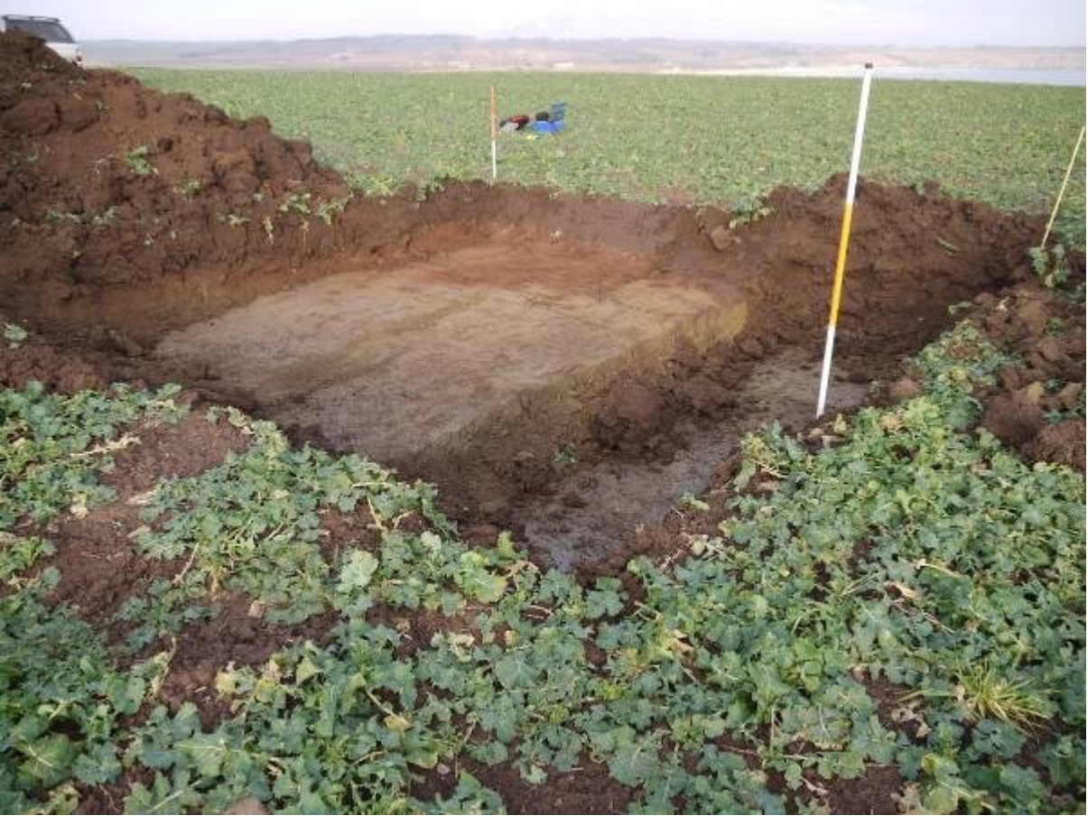
Illus 9 Stripped area for Turbine 2 looking North West showing surface of natural clay
