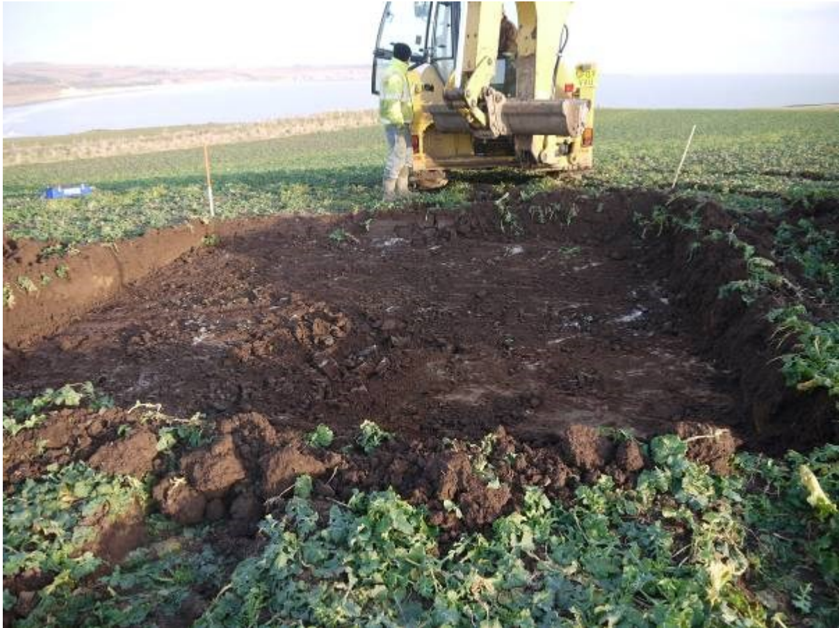
Illus 6 Stripped area for turbine 1 looking North East following removal of plough soil onto natural rock surface
