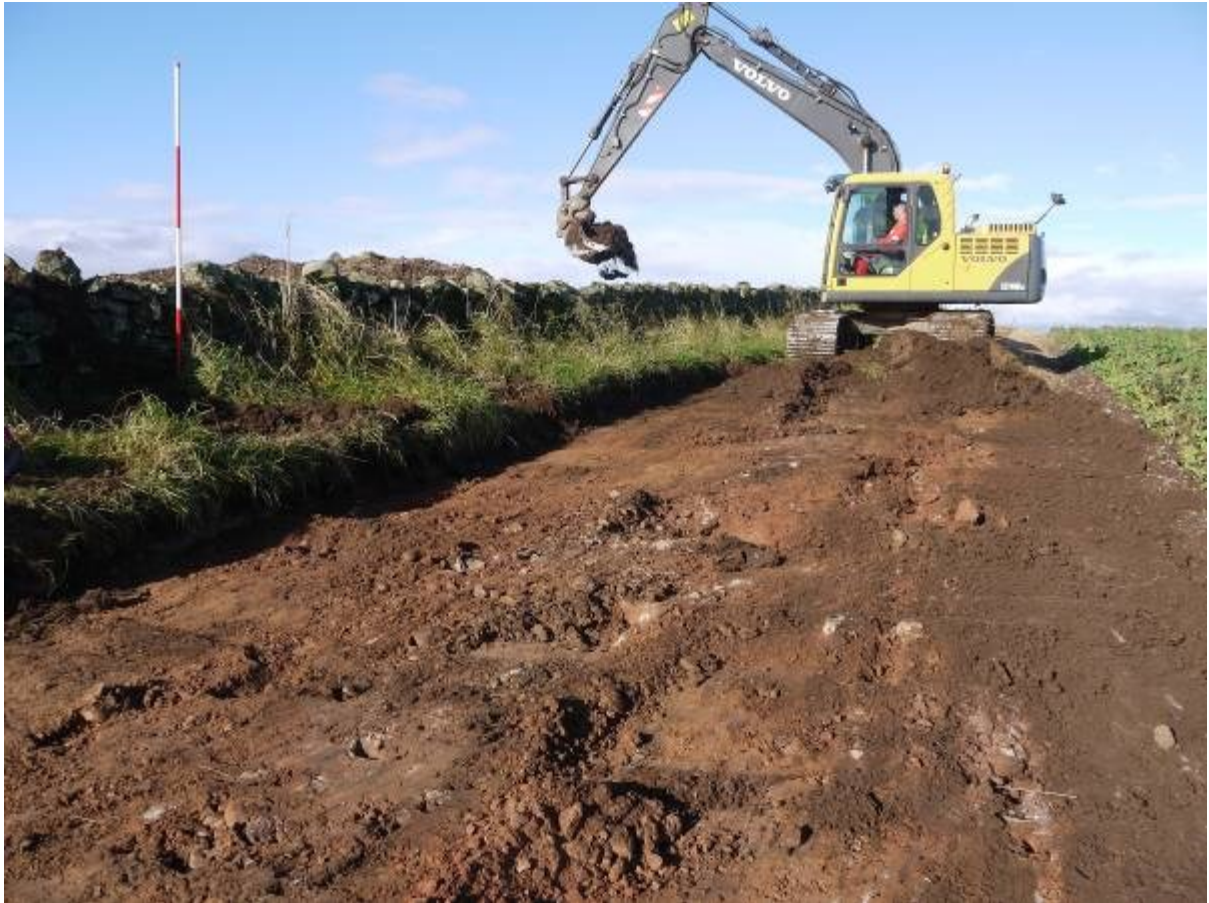
Illus 33 Access track to turbine 7 showing natural ground surface looking North West
