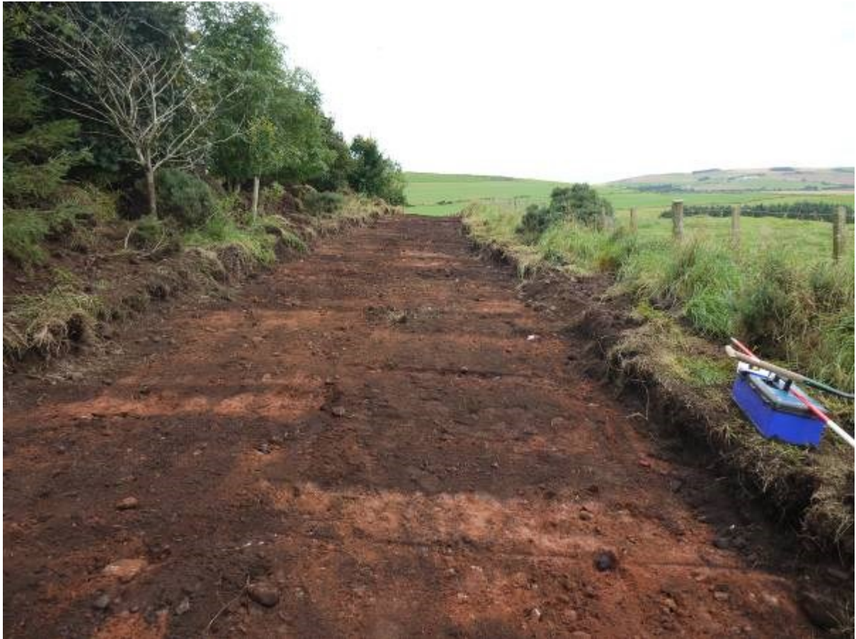
Illus 7 Final stretch of stripped access track to wind turbine 3 looking South East
