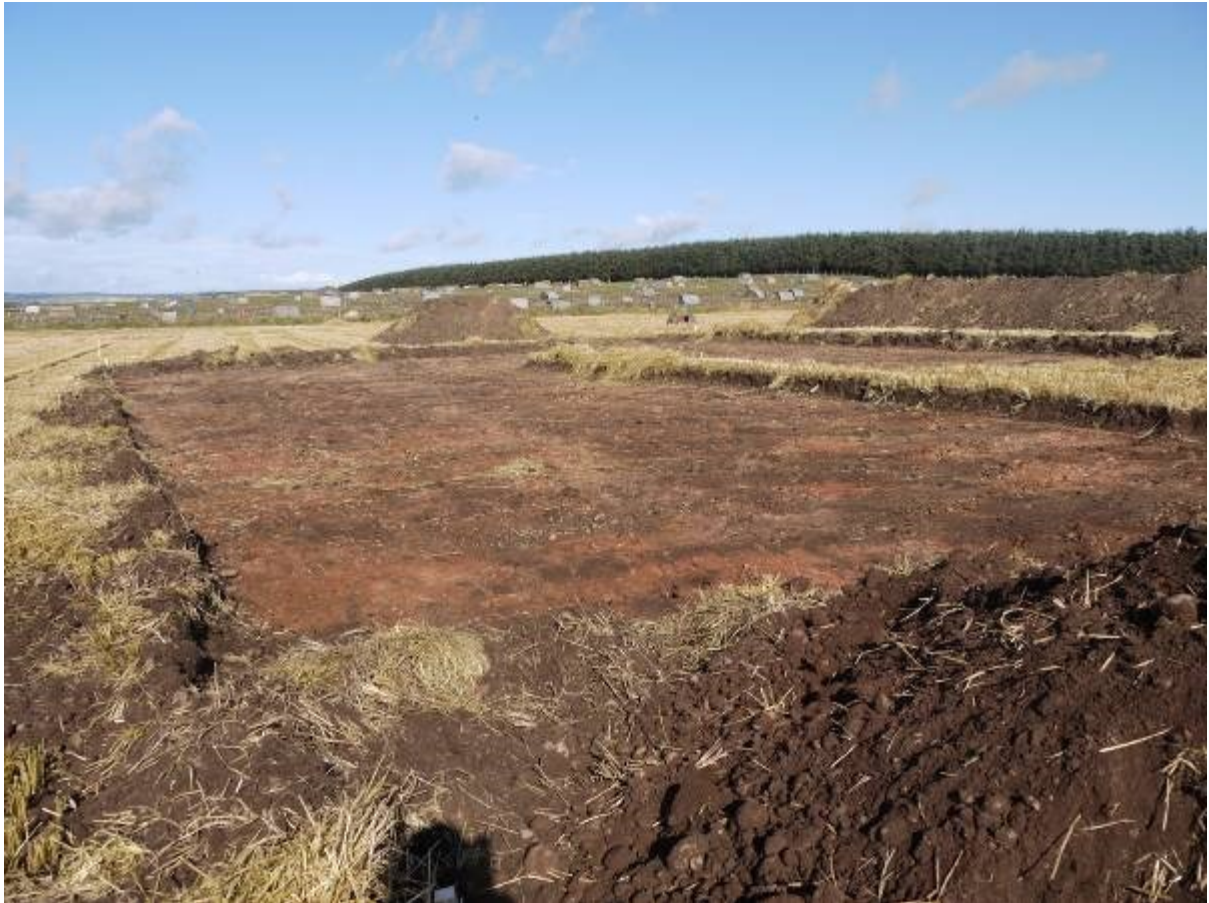
Illus 9 Area stripped for crane pad for wind turbine 6 showing natural ground surface visible below plough soil looking North West
