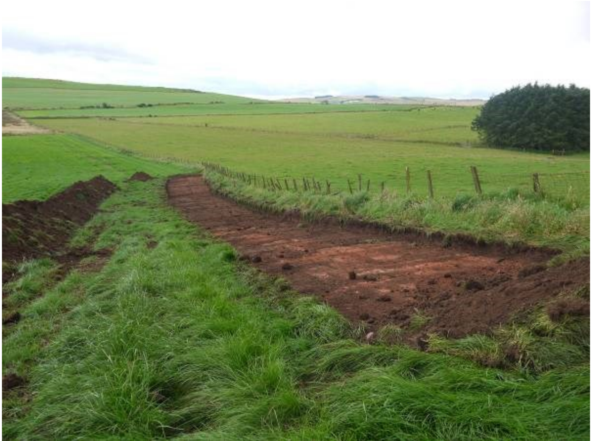
Illus 5 Access track to wind turbine 3 stripped to top of hill looking South East
