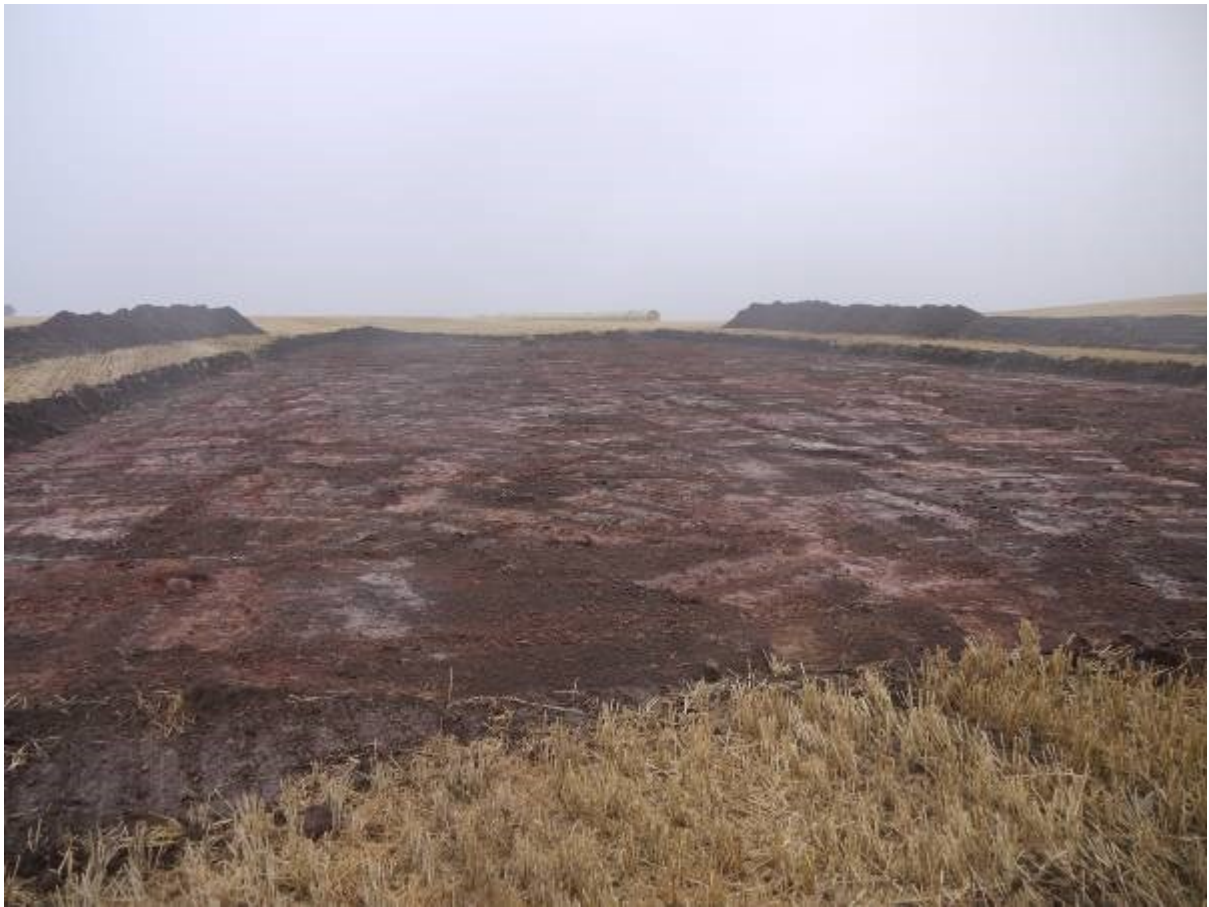
Illus 16 Stripped crane pad for turbine 8 showing natural ground surface looking South
