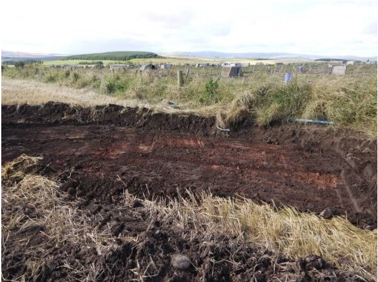
Illus 12 stripped access track for wind turbine 6 at junction with existing farm track showing natural ground surface looking South West
