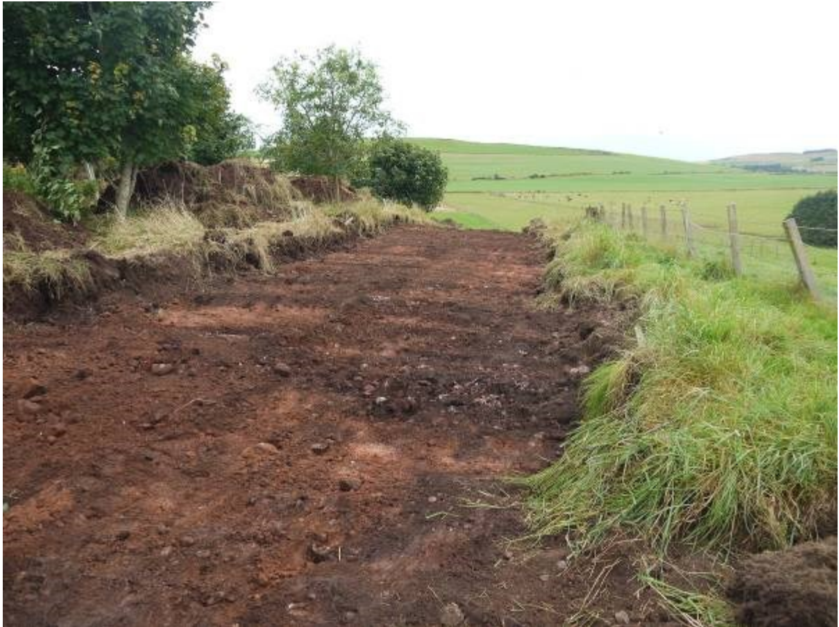
Illus 6 Access track to wind turbine 3 stripped adjacent to forestry plantation looking South East
