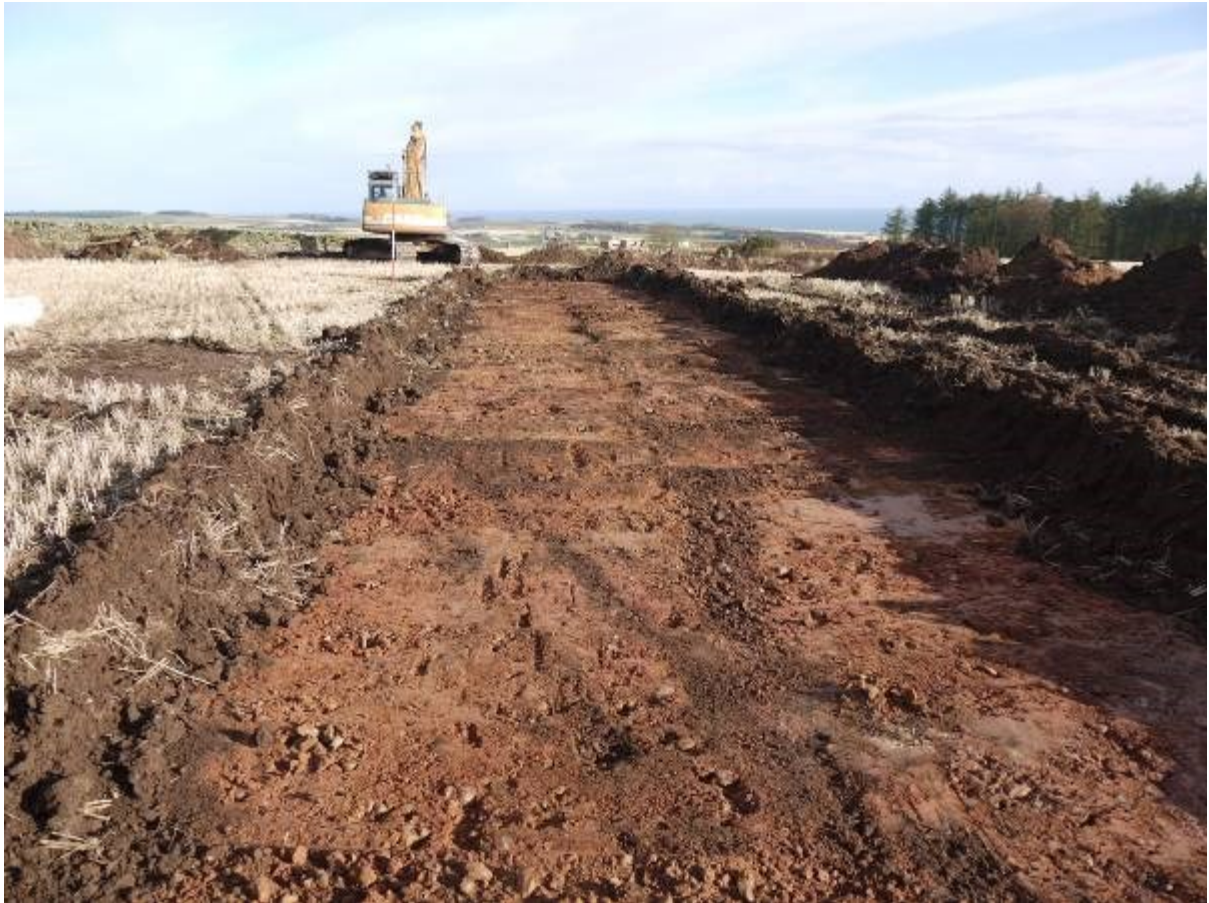
Illus 25 Replacement access track for wind turbine 8 showing natural ground surface with plough scars looking North
