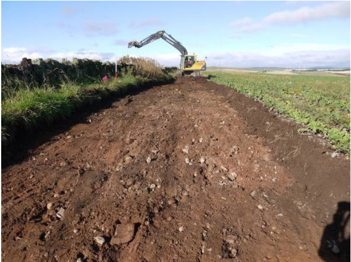
Illus 34 Access track to turbine 7 showing previous road metalling on natural ground surface looking North West
