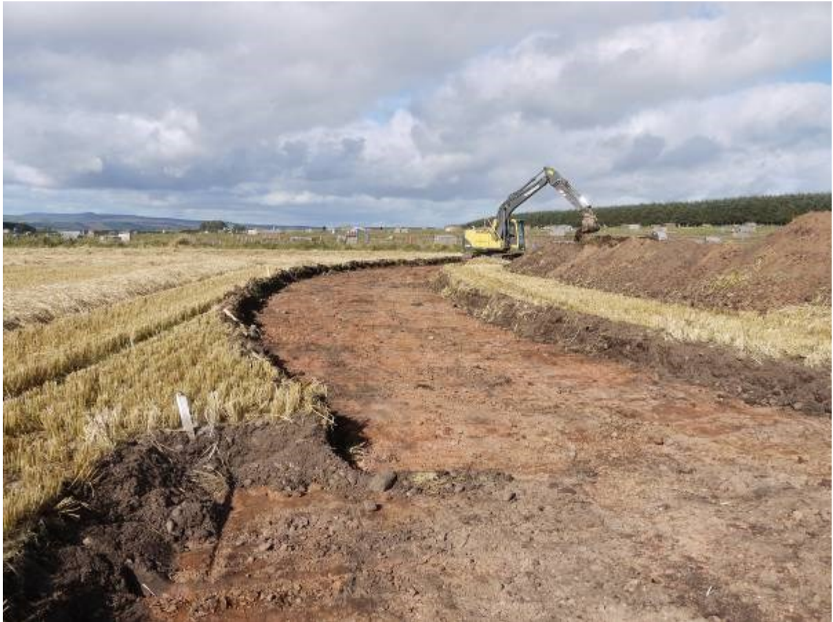
Illus 11 Access track for wind turbine 6 showing natural ground surface looking North West
