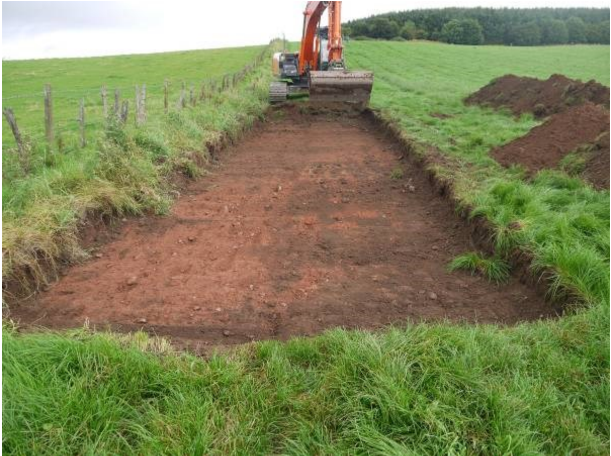
Illus 4 Access track to wind turbine 3 being excavated looking North West showing natural ground surface visible below ploughsoil
