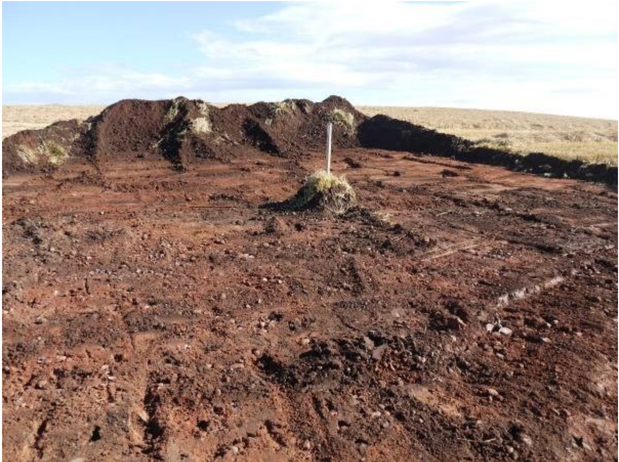
Illus 10 Base for wind turbine 6 stripped showing natural ground surface looking North
