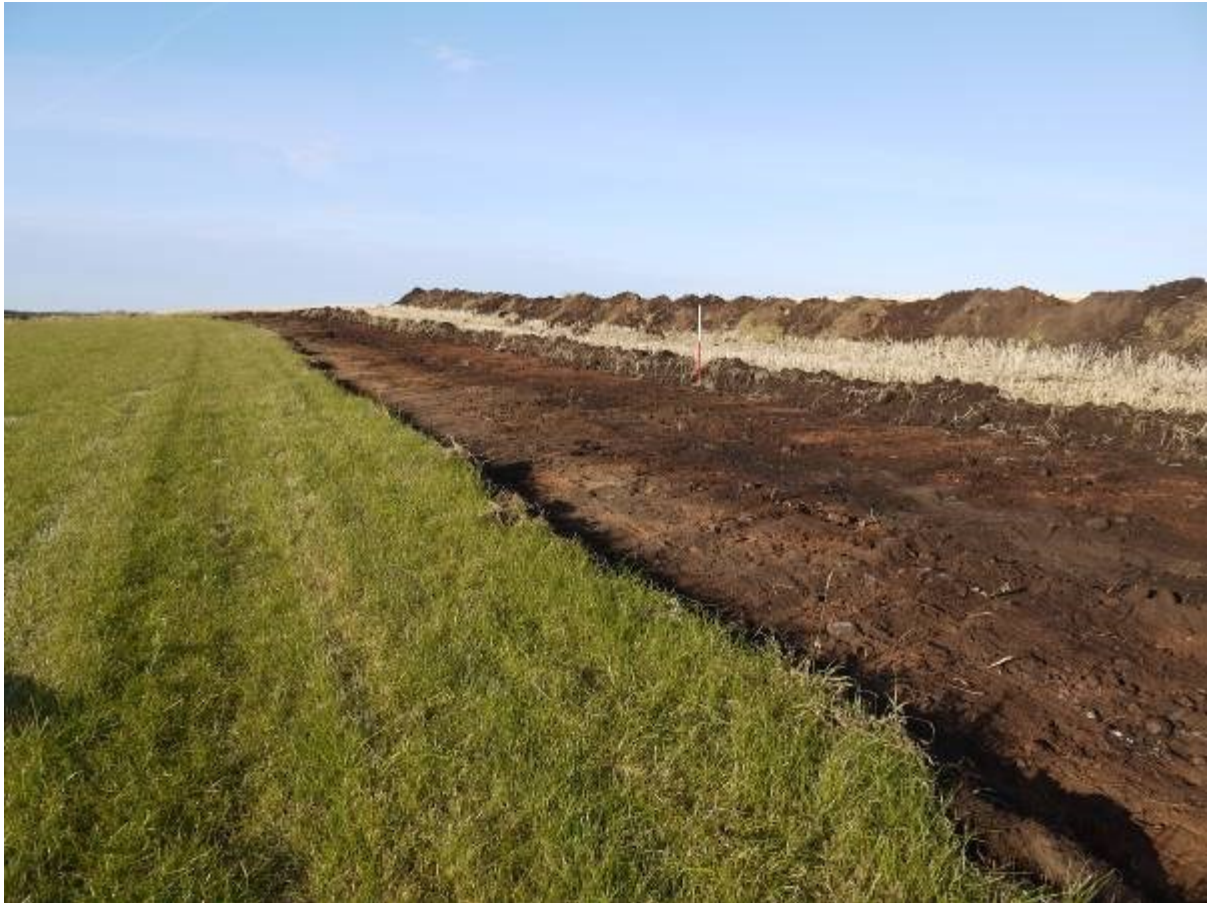
Illus 14 Stripped access track to wind turbines 8 and 9 showing former field boundary visible as linear black stain looking South West
