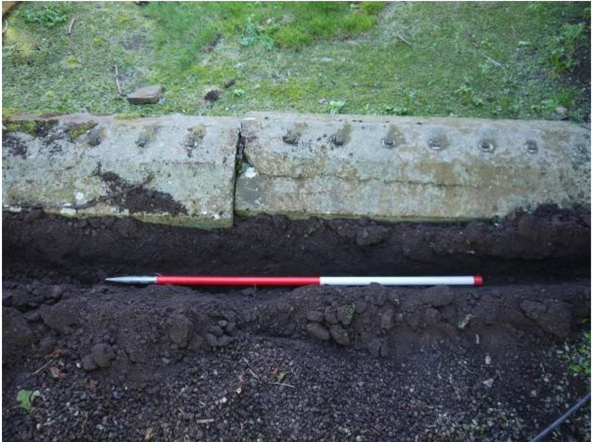
Illus 9 Excavated trench for cable for bulkhead light looking North (C on illus 3)
