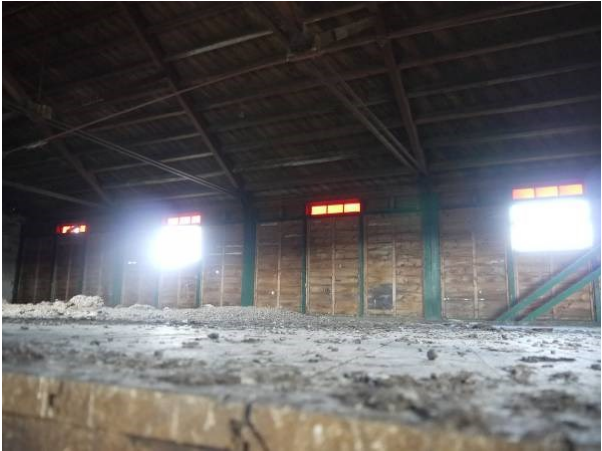
Illustration 22 northern side of top floor of Building A showing four of red leaded glass louvers
