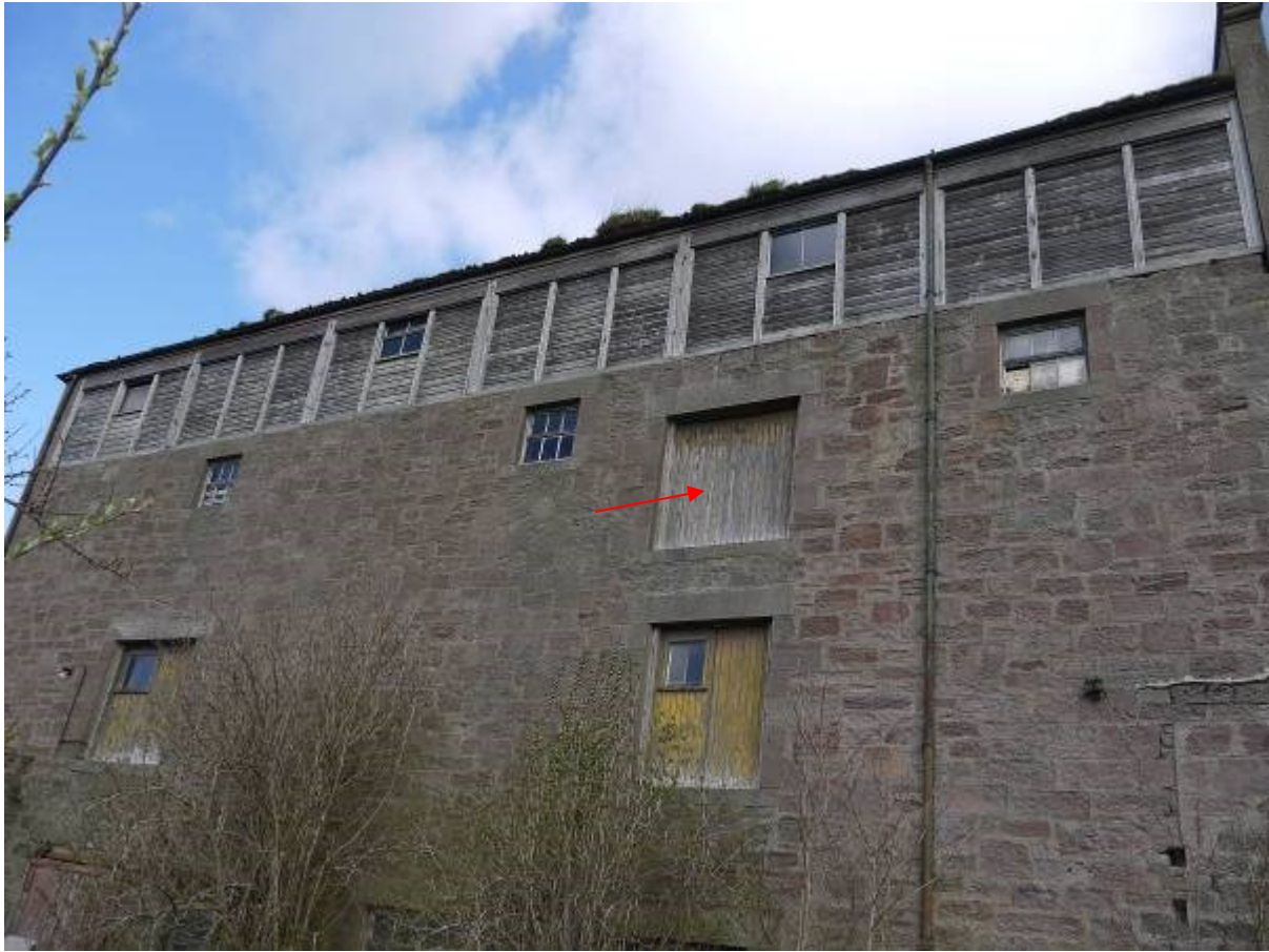
Illustration 11 southern elevation of Building A, red arrow indicates door in front of chute on first floor (see Illus 18)
