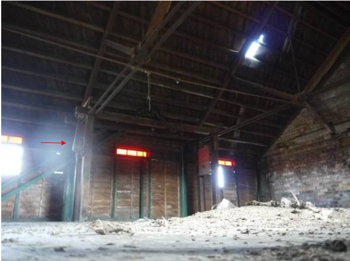
Illustration 23 eastern end of top floor of Building A showing remaining red leaded glass louvers and fire extinguisher at red arrow
