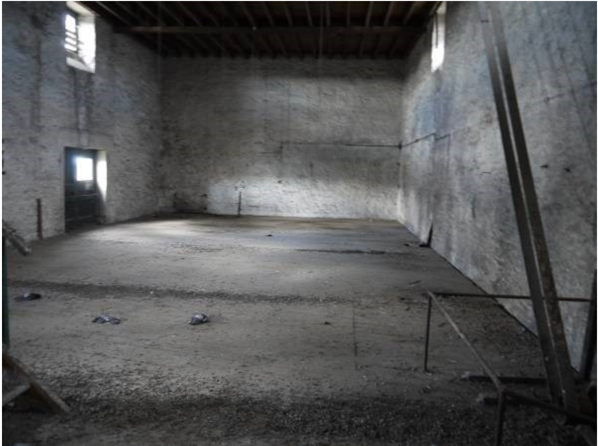
Illustration 19 western end of first floor of Building A electric motor and belt visible to right
