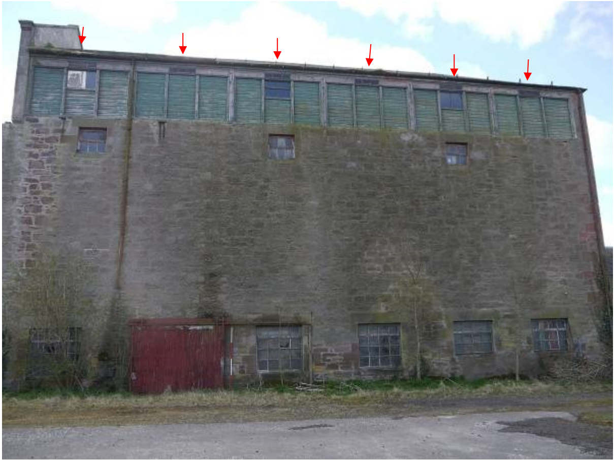
Illustration 9 northern elevation of Building A (louvers at top floor level marked with red arrows)
