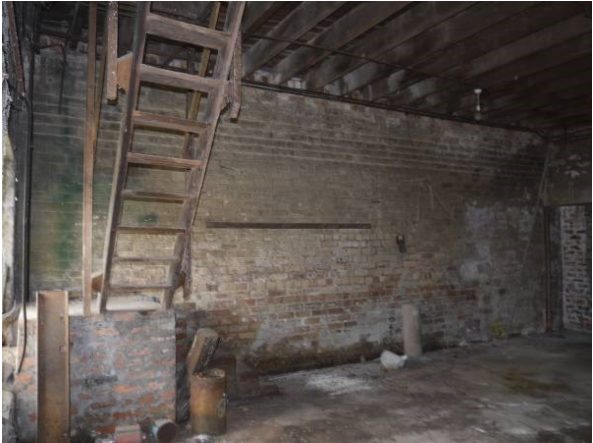
Illustration 13 Ground floor of Building A accessible from north side showing wooden stair to first floor
