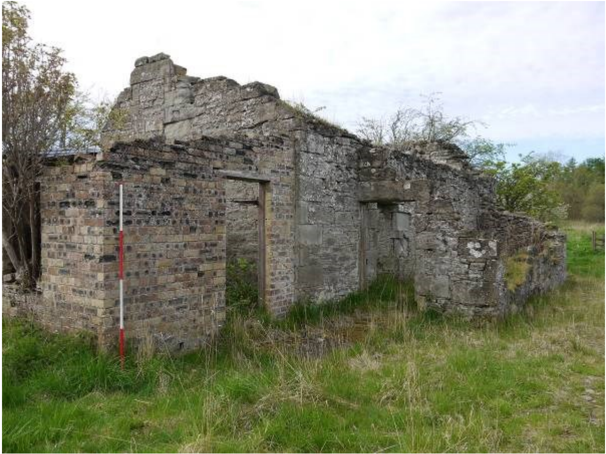
Illustration 7 Eastern end of Northern elevation of Building A showing brick extension and front porch looking west
