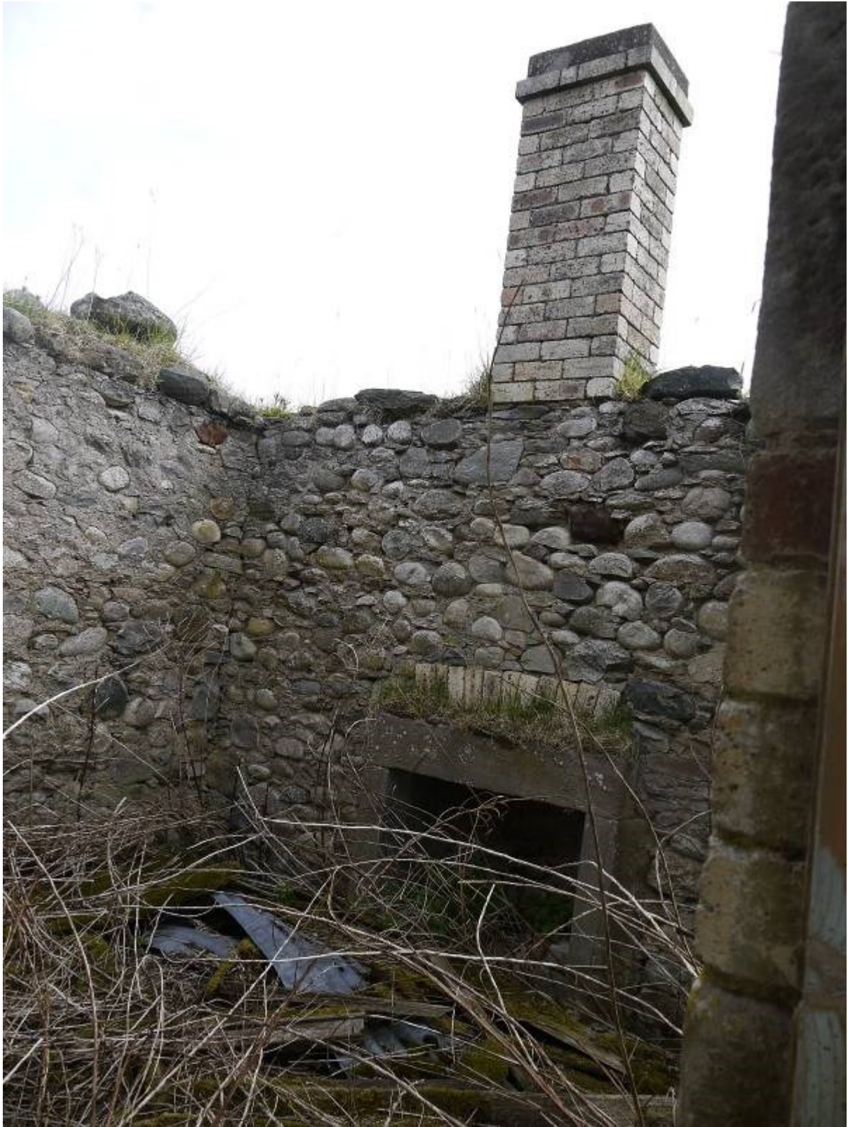
Illustration 33 Interior of room at southern end of Building E showing fireplace and associated brick chimney looking north east
