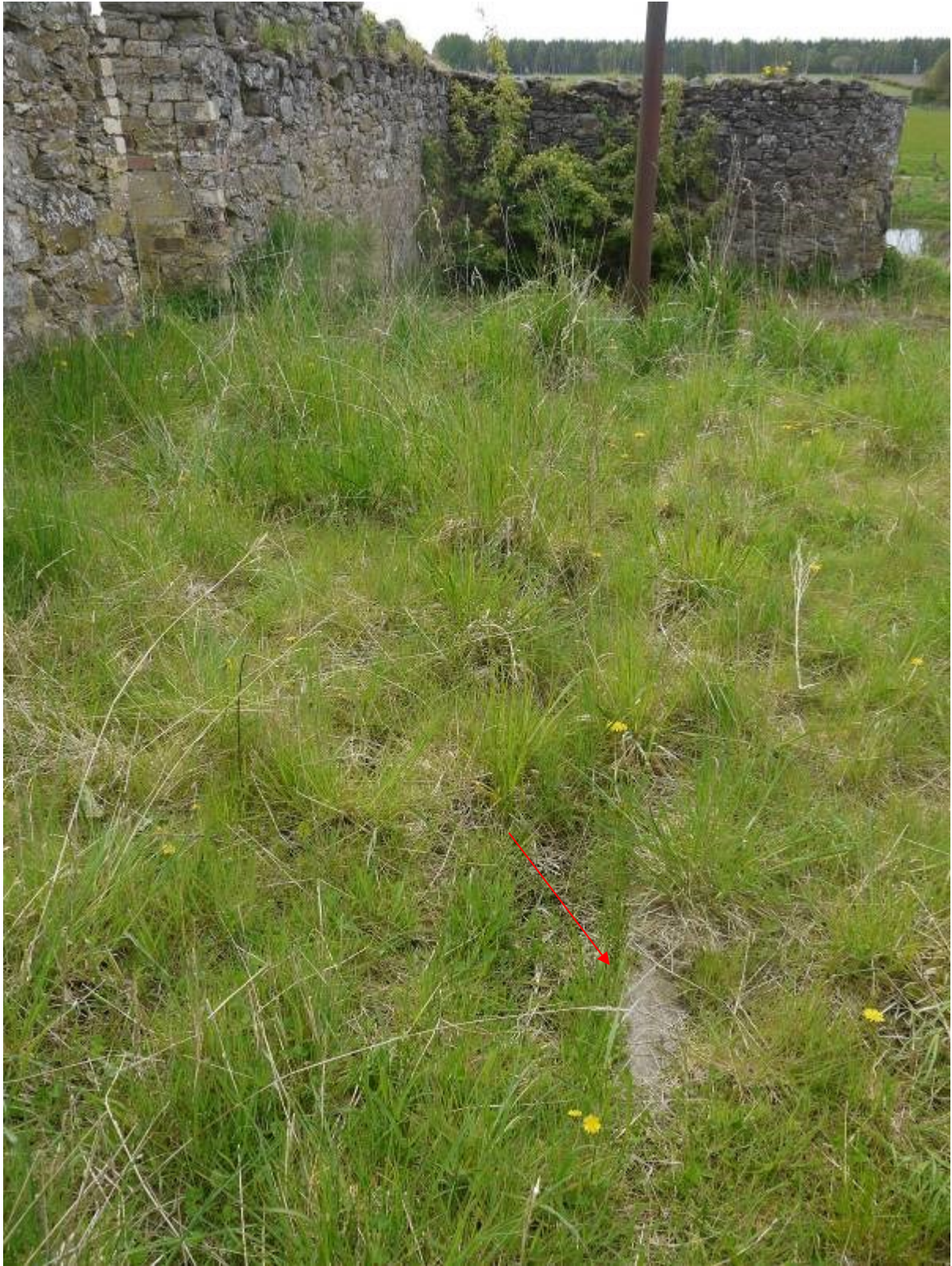
Illustration 26 Drain in floor at eastern end of Building C (red arrow), surviving cast iron roof support visible in back ground
