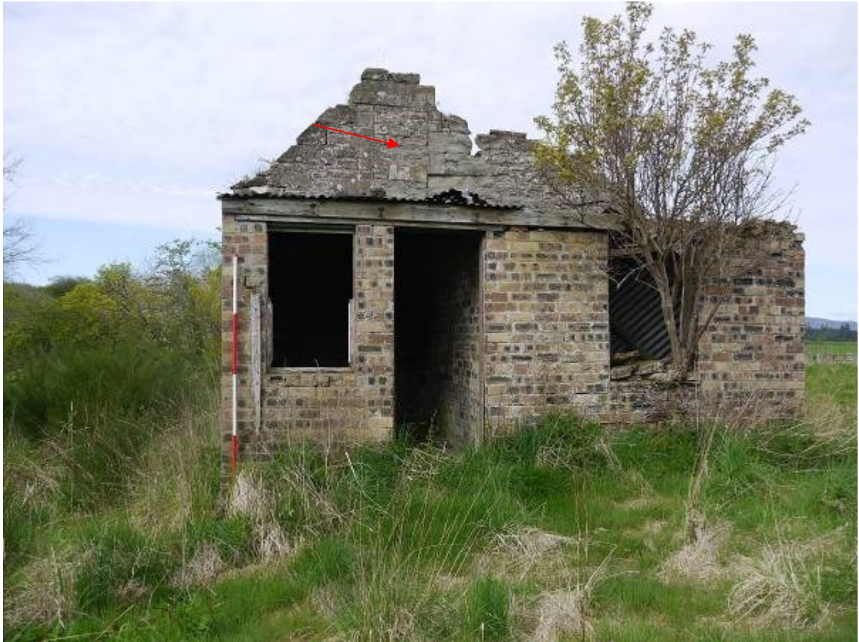
Illustration 11 Eastern elevation of Building A showing brick extension, blocked window in farmhouse wall marked with red arrow
