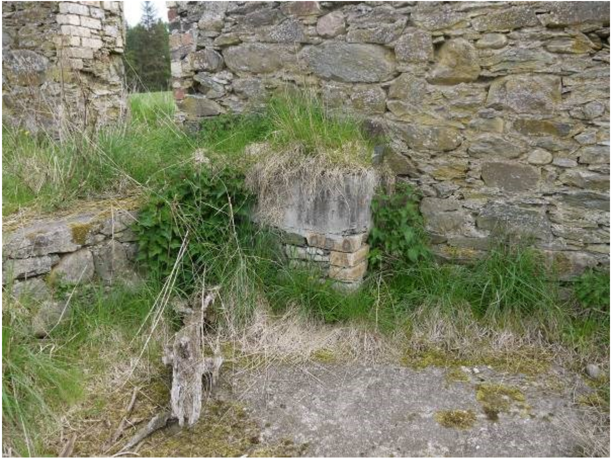
Illustration 29 Water tank at north eastern end of Building D
