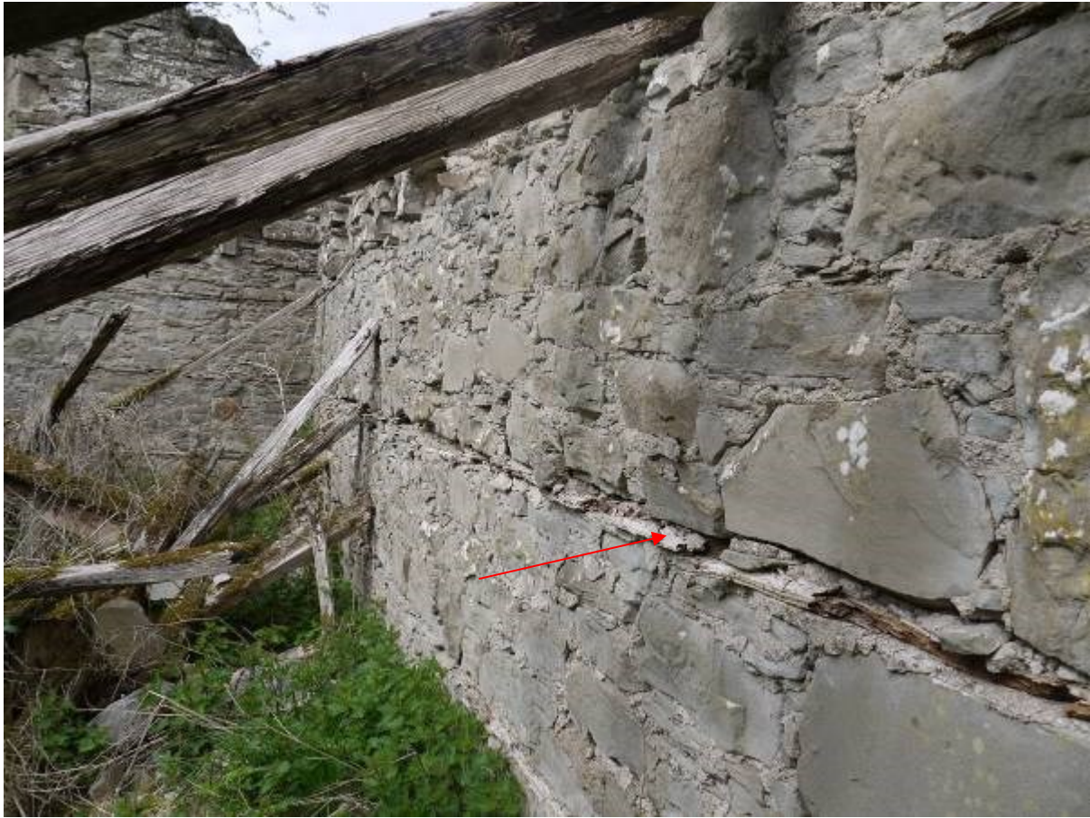
Illustration 15 Internal southern elevation of Building A showing plank built into wall (red arrow)
