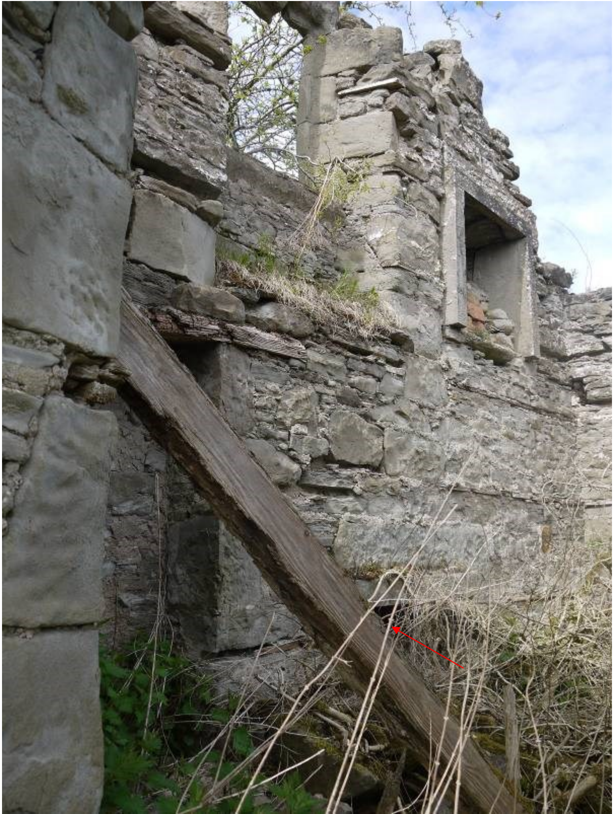
Illustration 14 Internal eastern elevation of Building A showing fireplace and window on first floor level, red arrow indicates ground floor fireplace
