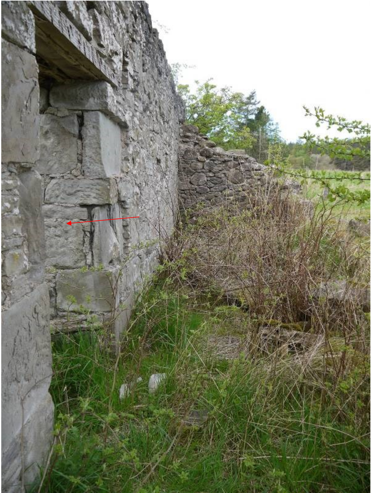
Illustration 8 interior of 'porch' of Building A looking west, doorway into house marked with red arrow
