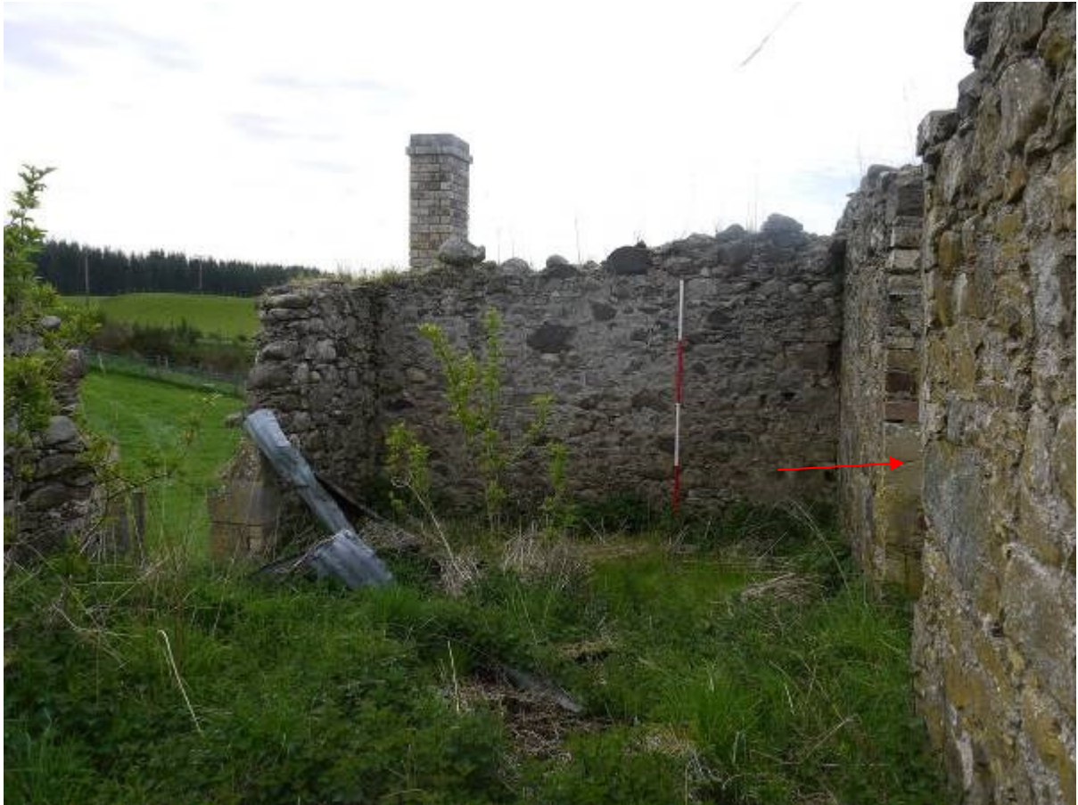
Illustration 34 Southern half of other room in Building E looking south, doorway into Building C marked by red arrow
