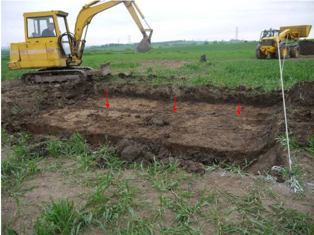
Illustration 13 Turbine plinth under excavation looking west showing surface of natural clay below ploughsoil, red arrows indicate course of field drain
