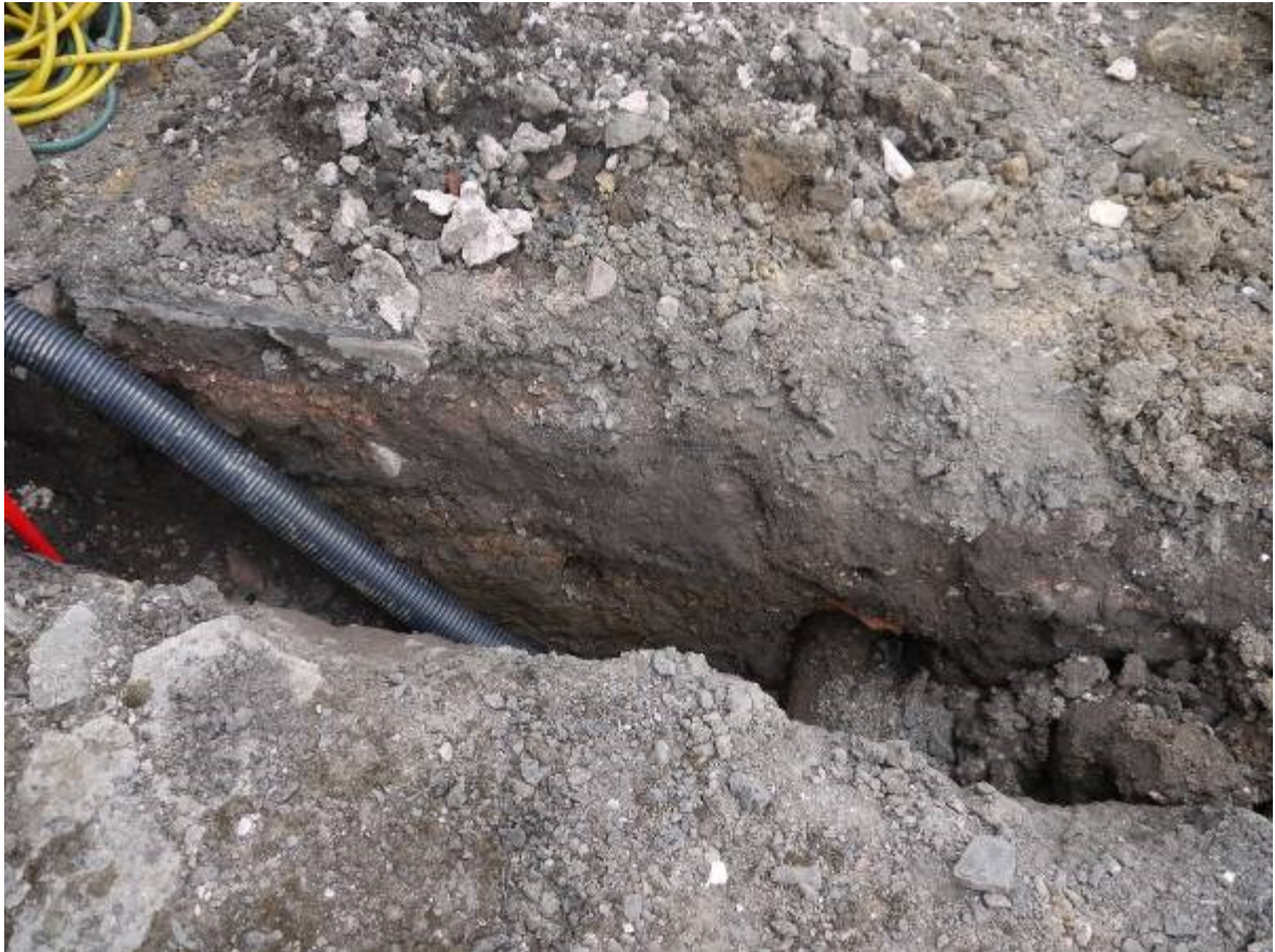
Illustration 5 West facing section of cable trench in vicinity of farm steadings, broken tile and brick visible in section
