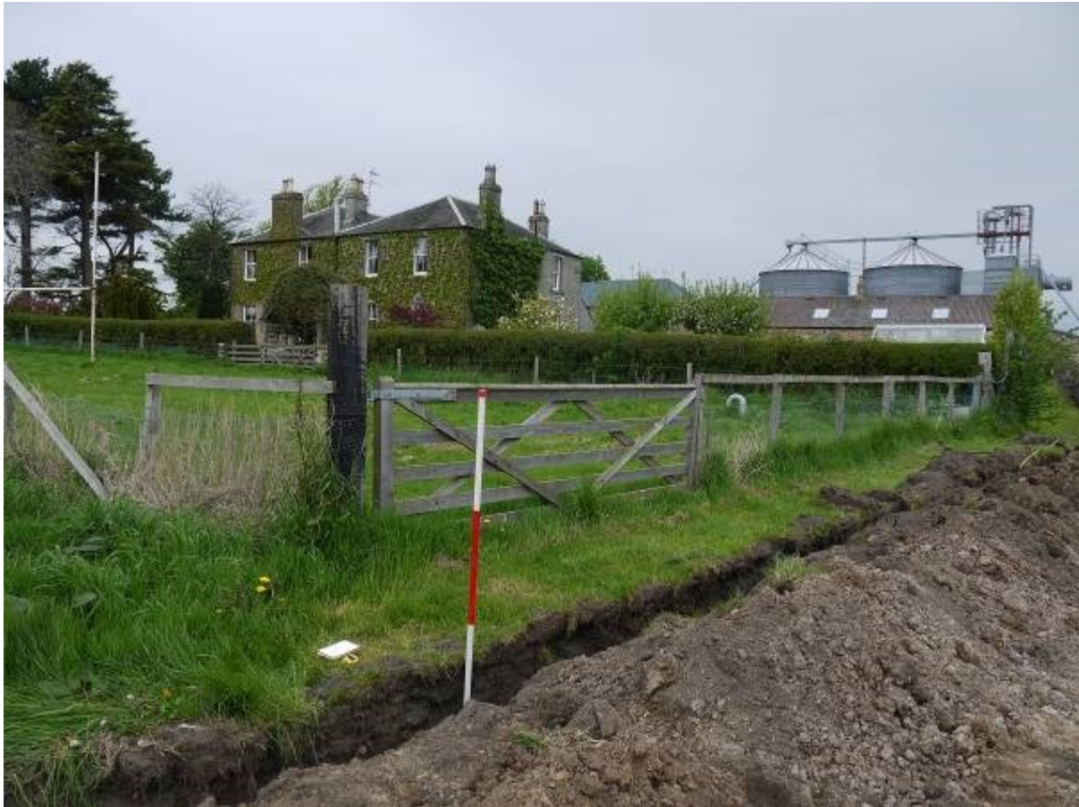
Illustration 10 General view of cable trench looking north west at entrance to field at point E on illustration 3
