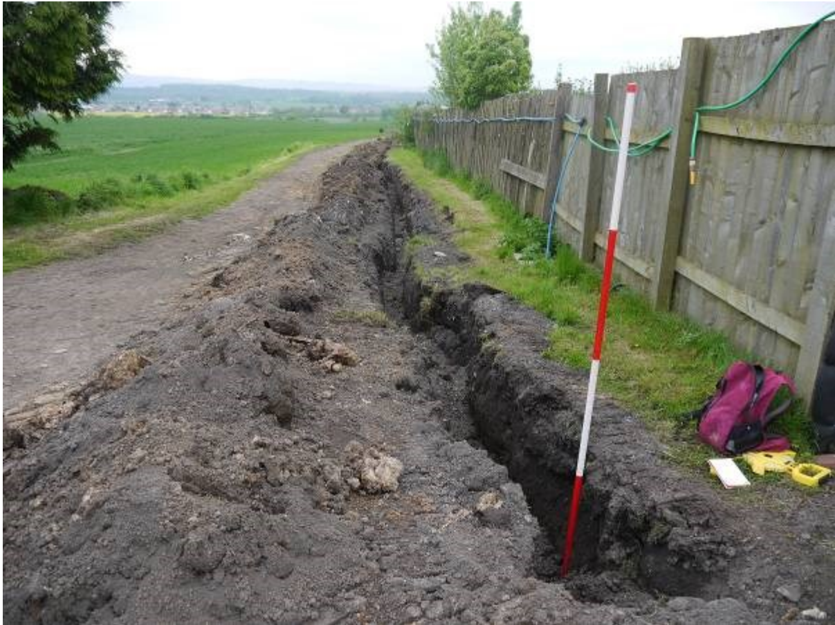
Illustration 6 Cable trench looking south towards site of turbine plinth, eastern boundary fence around farm on right
