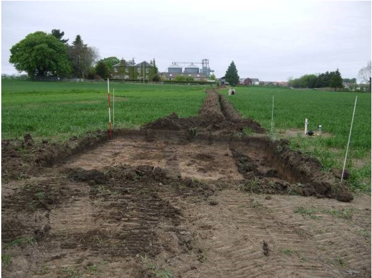
Illustration 14 General view of excavated turbine plinth and cable trench looking north showing natural clay
