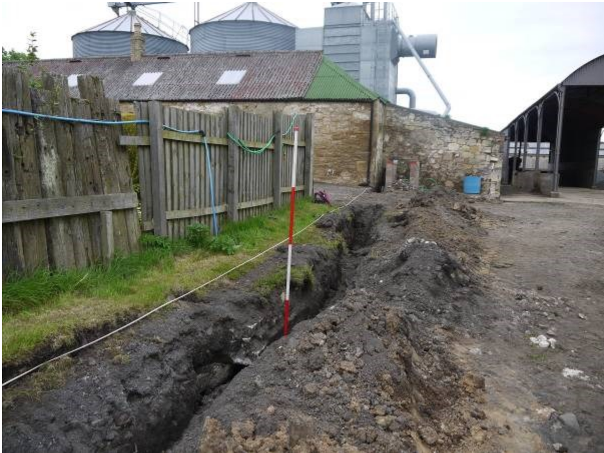
Illustration 8 Former septic tank in East facing section of cable trench at point c on illustration 3 looking north
