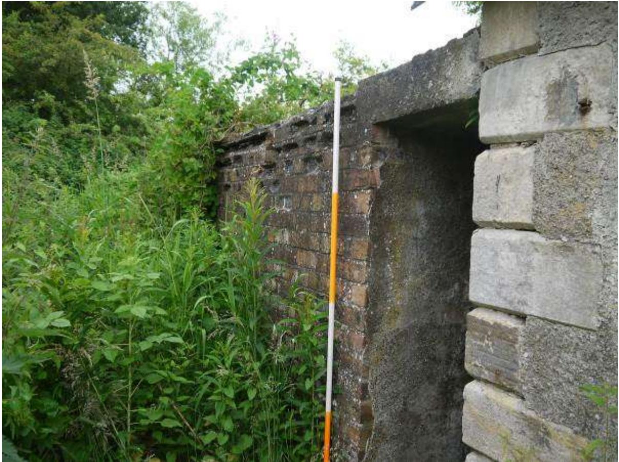
Illustration 11 south western end of eastern elevation of Building 1 showing brick extension and shaped sandstone quoins in corner of Building 1
