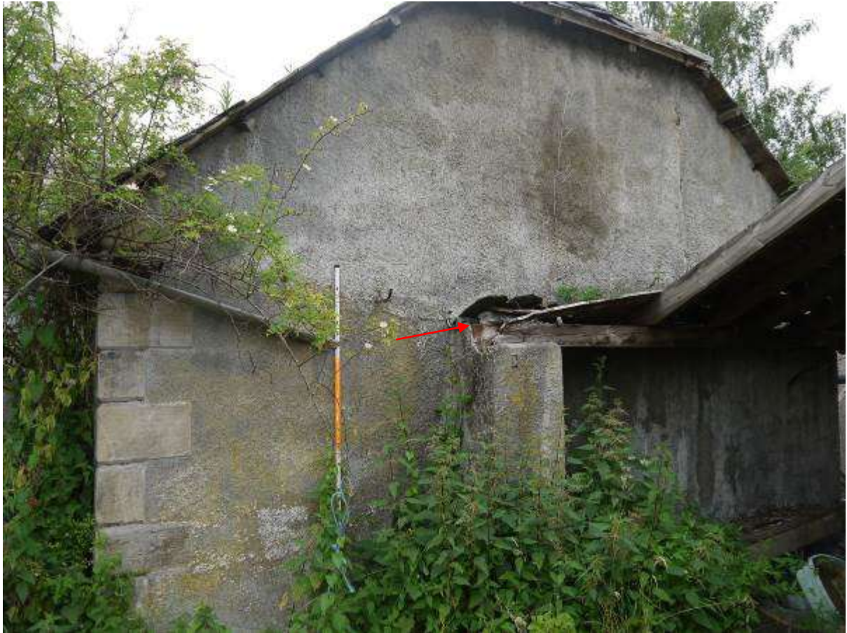
Illustration 12 north western end of south eastern elevation of Building 1 showing shaped sandstone quoins in front corner
