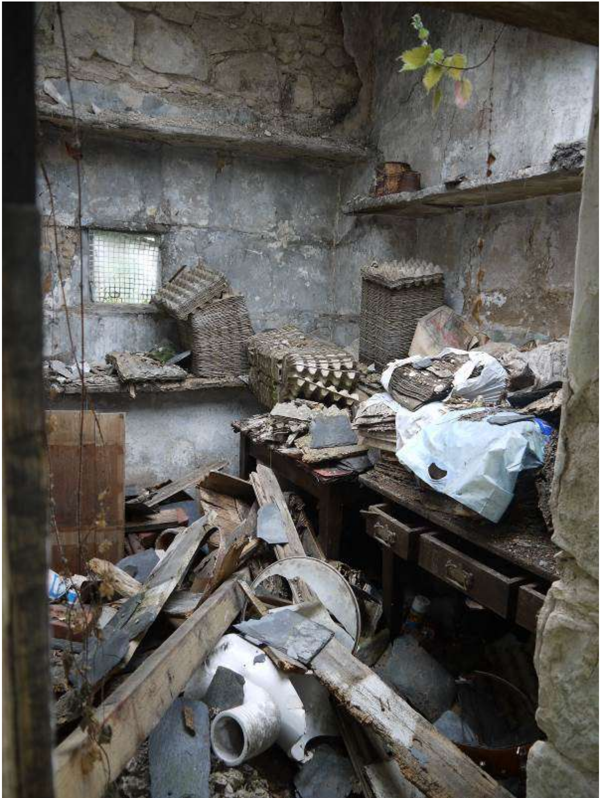
Illustration 22 Internal view of Room A in Building 3 showing window in boundary wall H, wooden furniture and egg boxes
