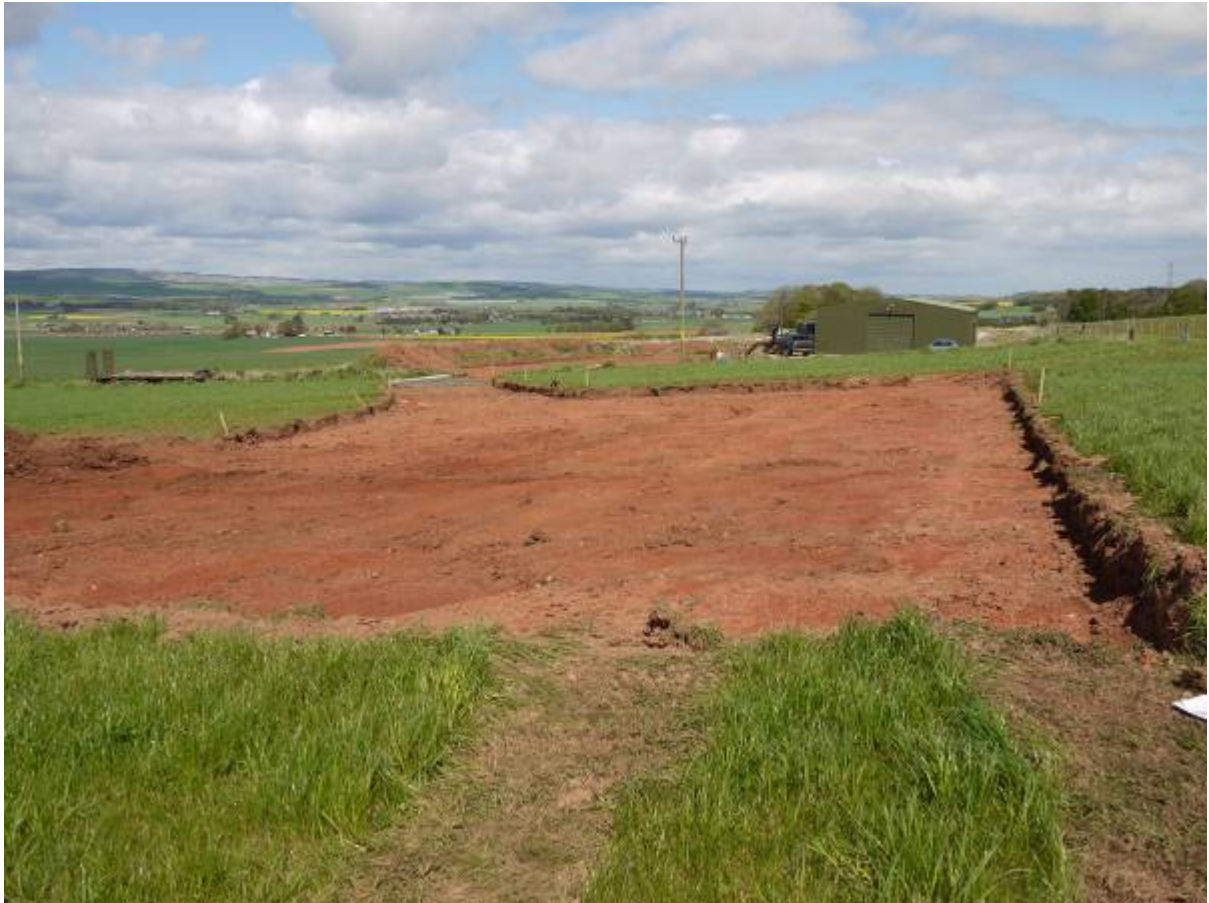
Illustration 12 Site B (house) southern side of plot and access road completely stripped of ploughsoil
