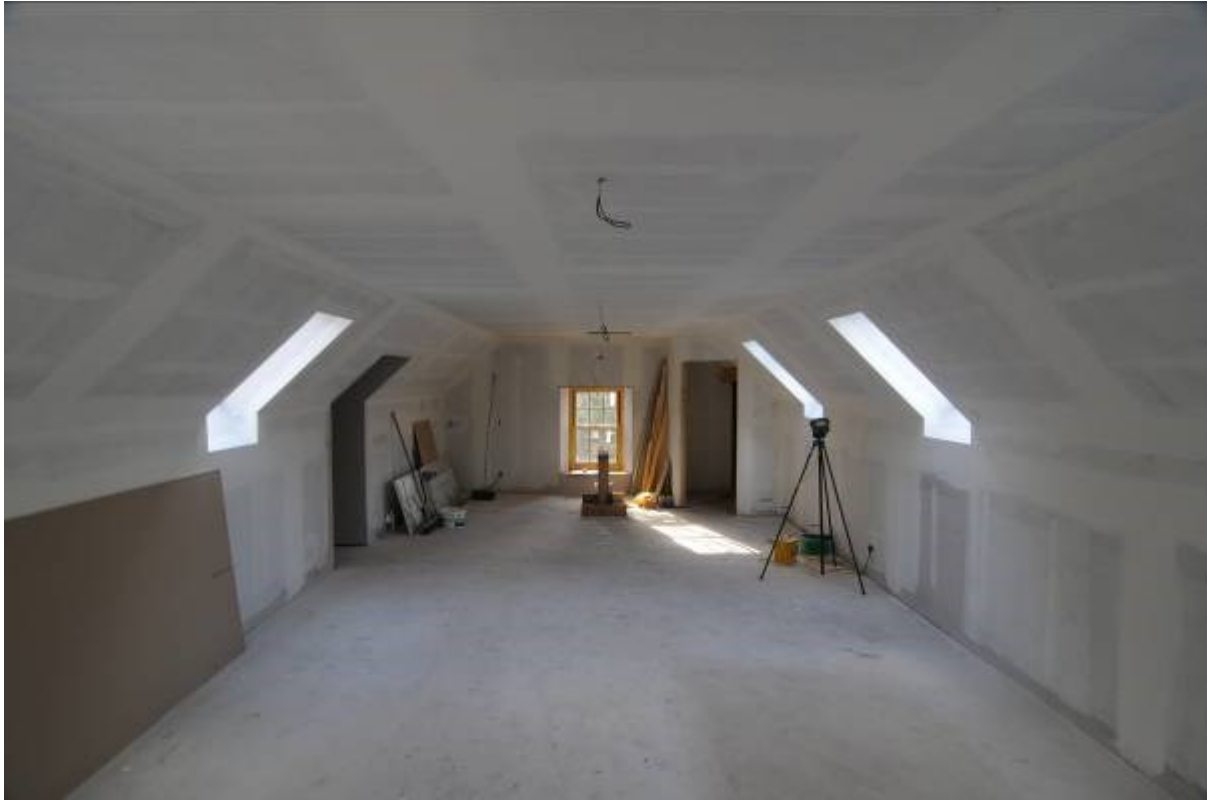
Illustration 11 General view of upper floor of former stables looking south, stair tower access to right
