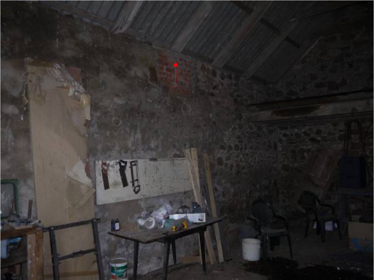
Illustration 20 Interior of southern end of Structure 1 showing blocked window at roof line (red arrow)
