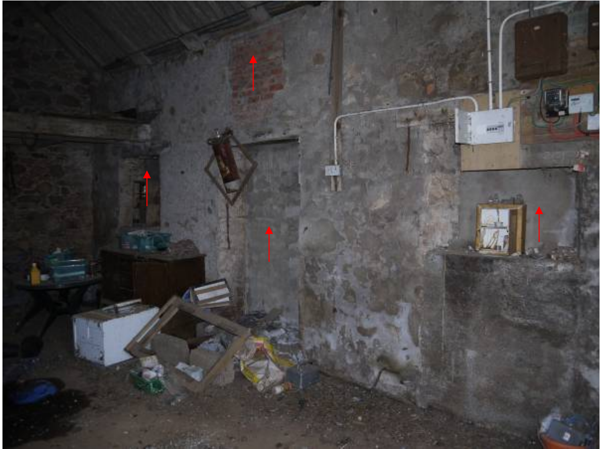
Illustration 19 View of interior of Southern end of Structure 1 showing blocked doorway and windows (red arrows) in Eastern wall
