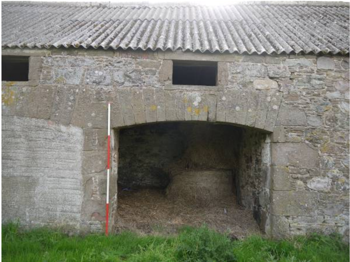
Illustration 7 Detail of West facing elevation showing arched doorways and small windows at roof line looking East
