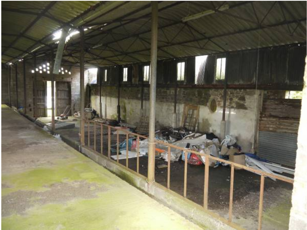
Illustration 17 Interior of Structure 3 from walkway looking South West, Eastern wall of Structure 1 in background
