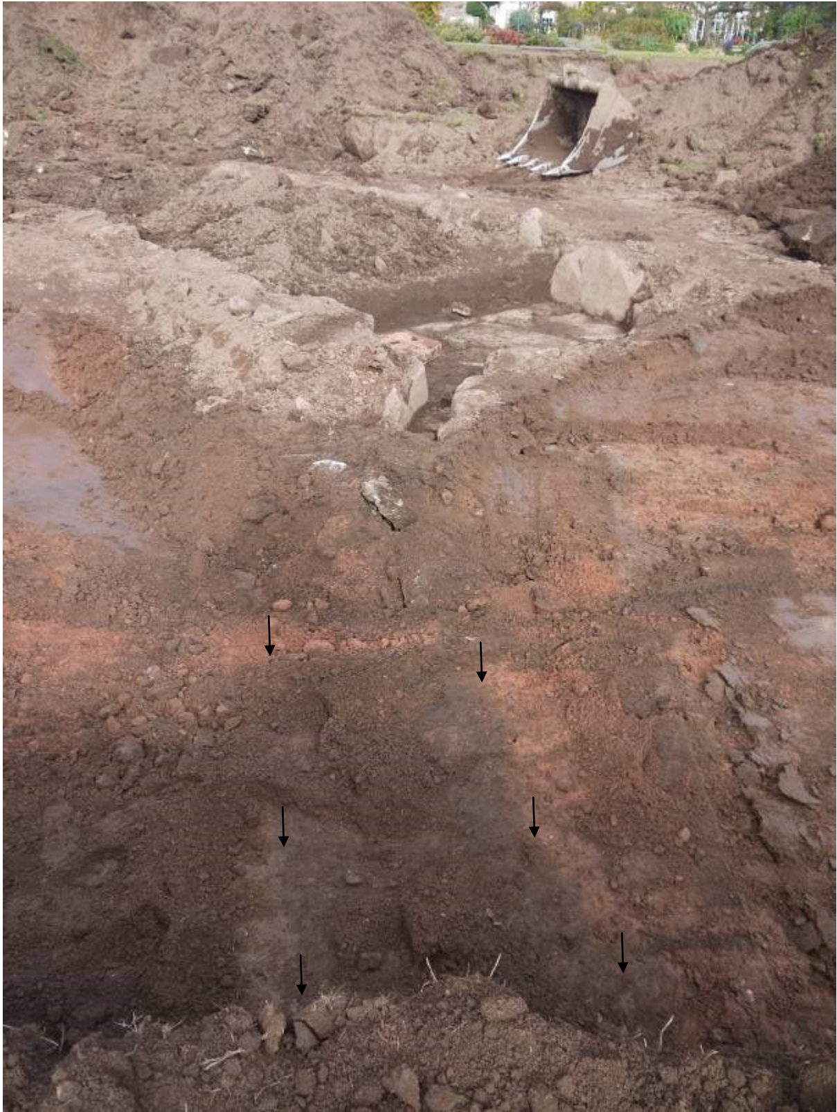
Illustration 11 - Line of drain 1006 from enclosed paved area visible in base of site strip (lines of arrows)
