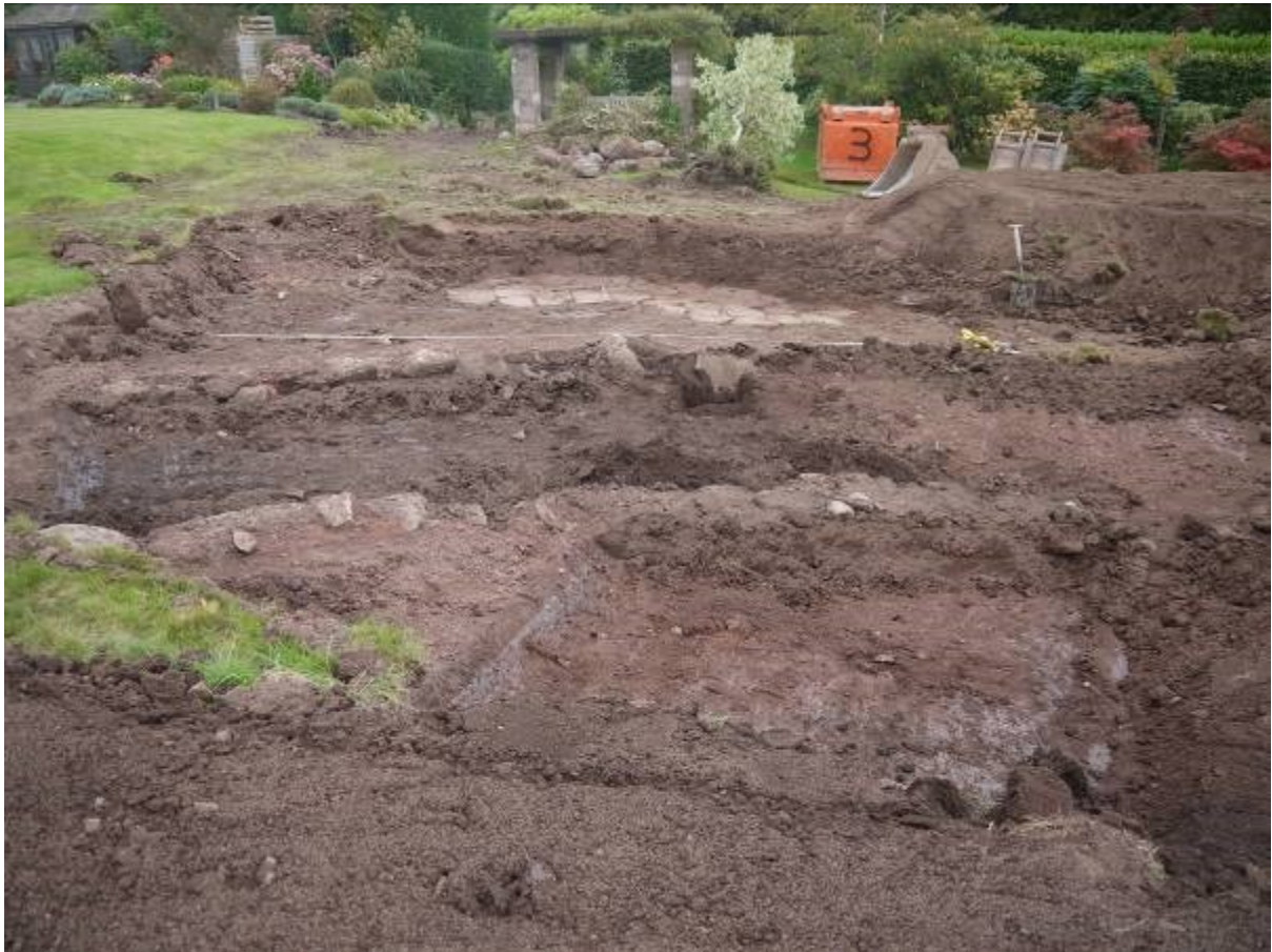
Illustration 7 General view of larger evaluation area looking East showing paving 1001 and walls 1003 and 1004 beginning to appear
