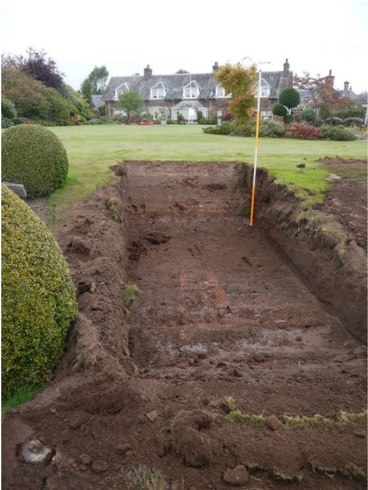
Illustration 13 – Trial trench E looking north towards ‘The Cottage’, line of sewer visible in foreground.
