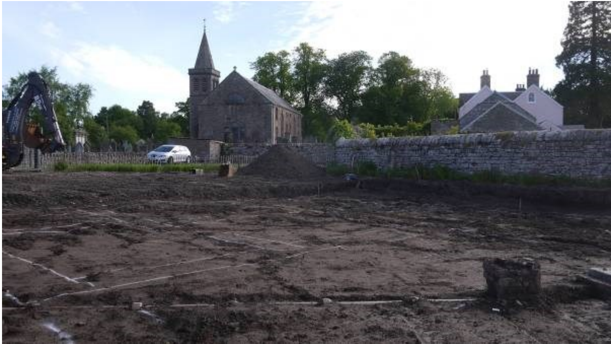
Illustration 5 Development site before commencement of foundation works looking East (Kettins Church and Manse visible in background)
