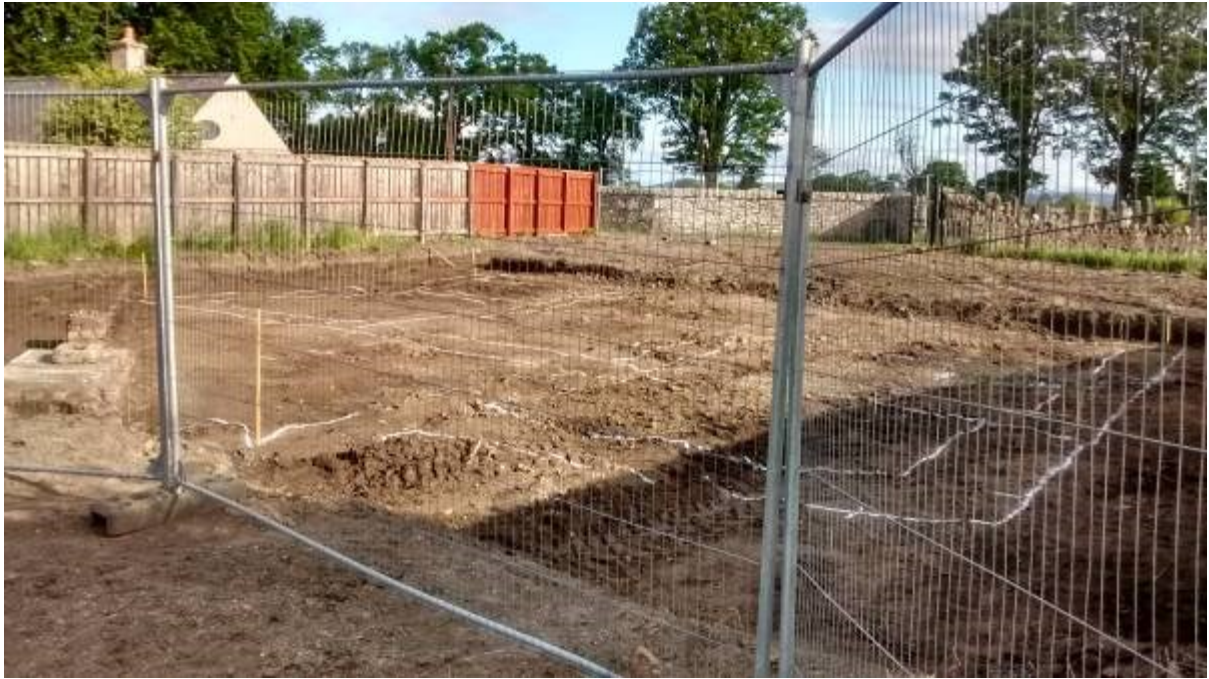
Illustration 4 Site after stripping of topsoil and marking out of proposed foundation lines looking North
