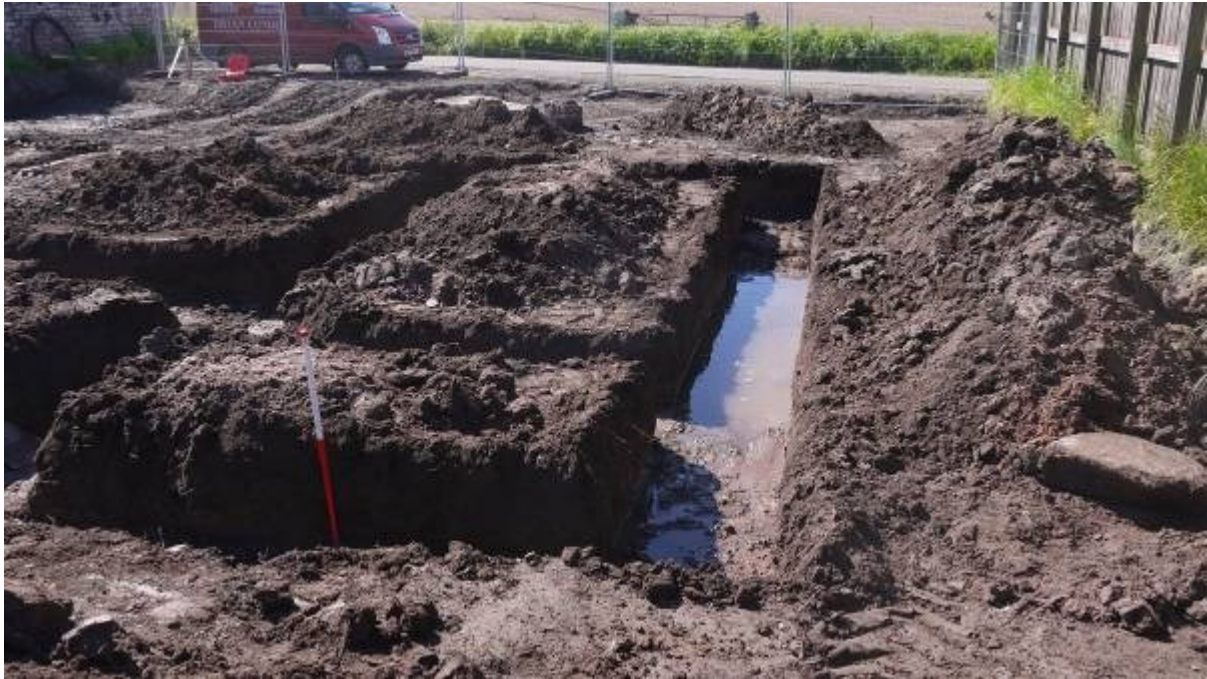
Illustration 6 Excavated foundation trenches at western end of site (top of water table is visible)
