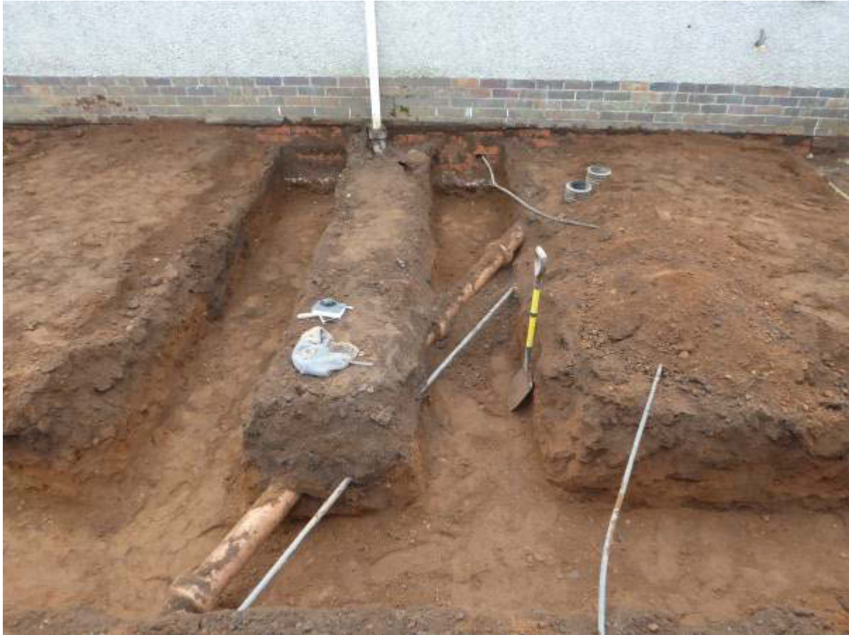
Illustration 9 General view of excavated line of western internal wall (C) looking South showing line of existing services.
