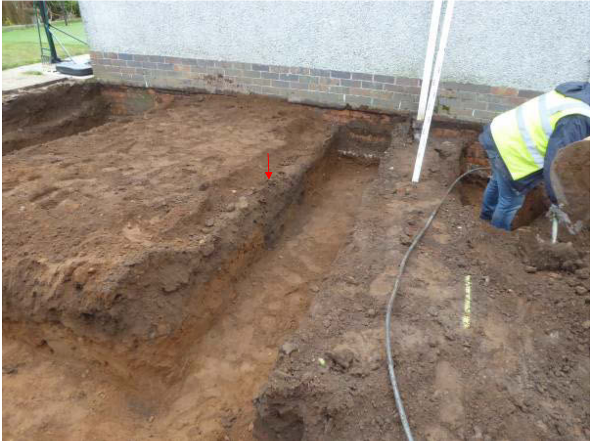
Illustration 7 Excavated trench for eastern internal wall division (B) looking South East, red arrow indicates location of cut feature 103.
