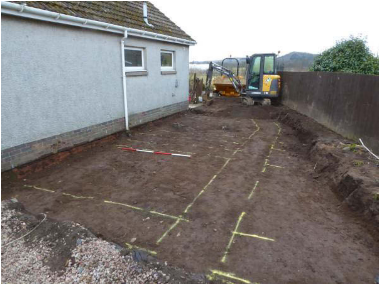
Illustration 5 General view of site of new extension looking West, wall lines marked out in yellow
