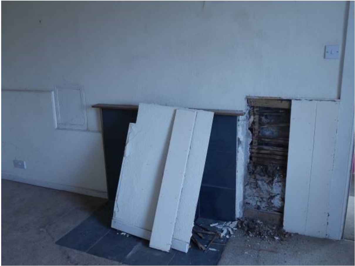
Illustration 14 Fireplace in lounge (3) with wooden lath and plaster exposed in wall
