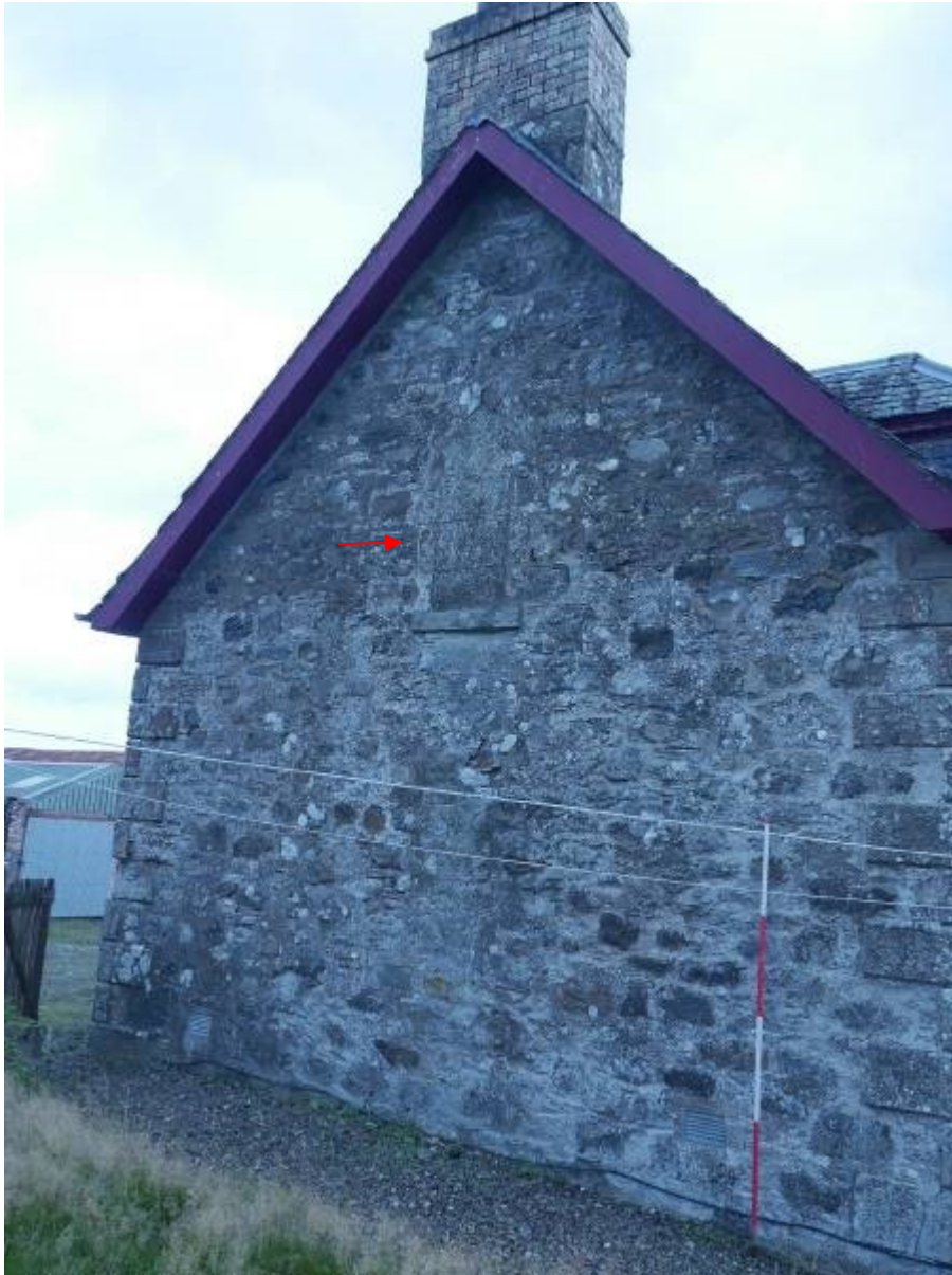
Illustration 9-Western elevation of farmhouse looking North East showing blocked arched window at first floor level (red arrow).
