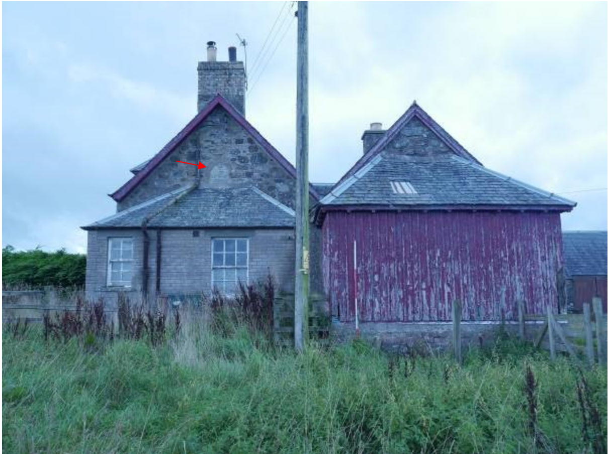
Illustration 11-Eastern elevation of farmhouse looking West, blocked window with round headed arch visible behind later toilet/bathroom block (red arrow).
