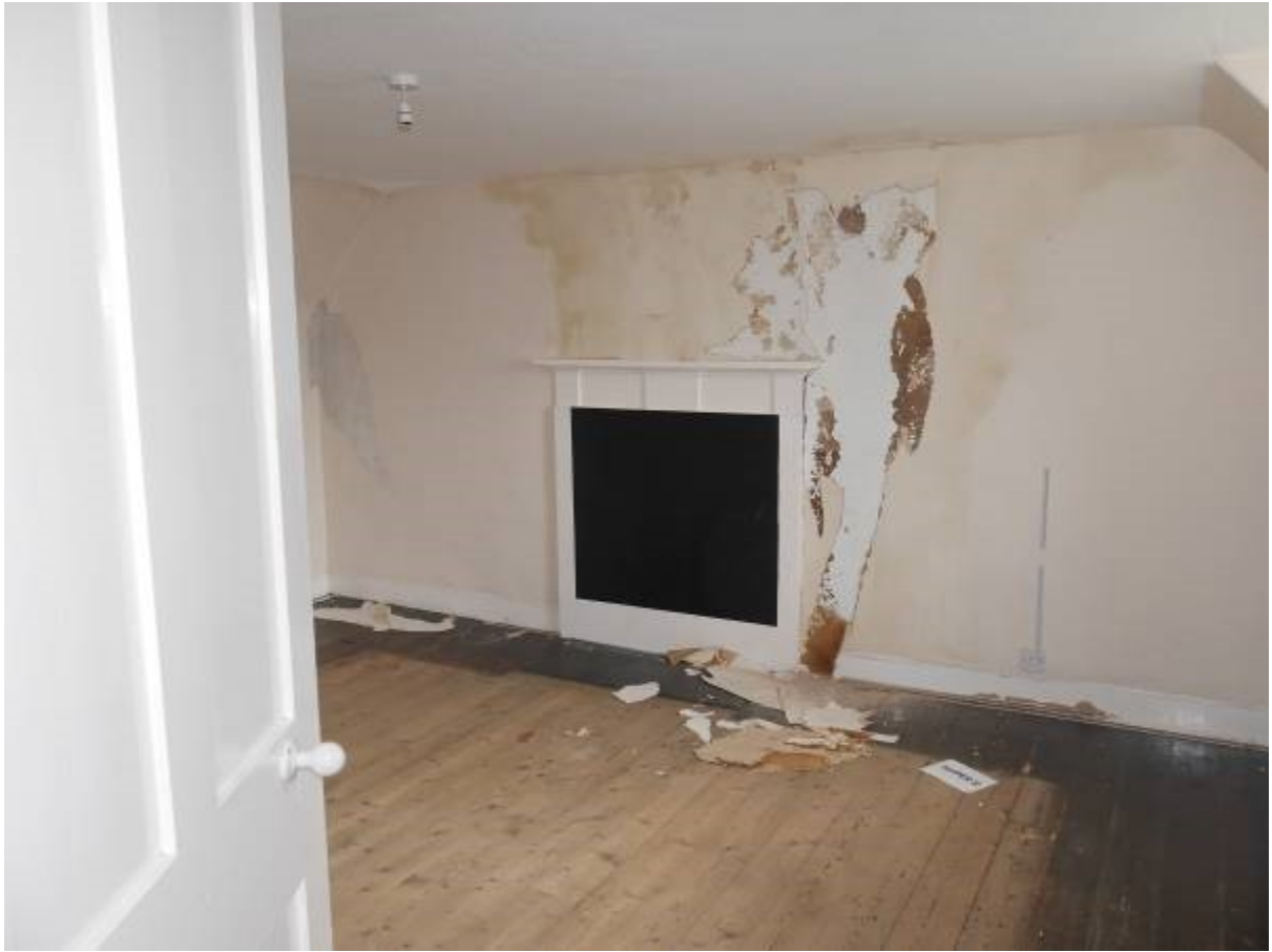
Illustration 25- Blocked fireplace in upstairs bedroom (10) looking North East
