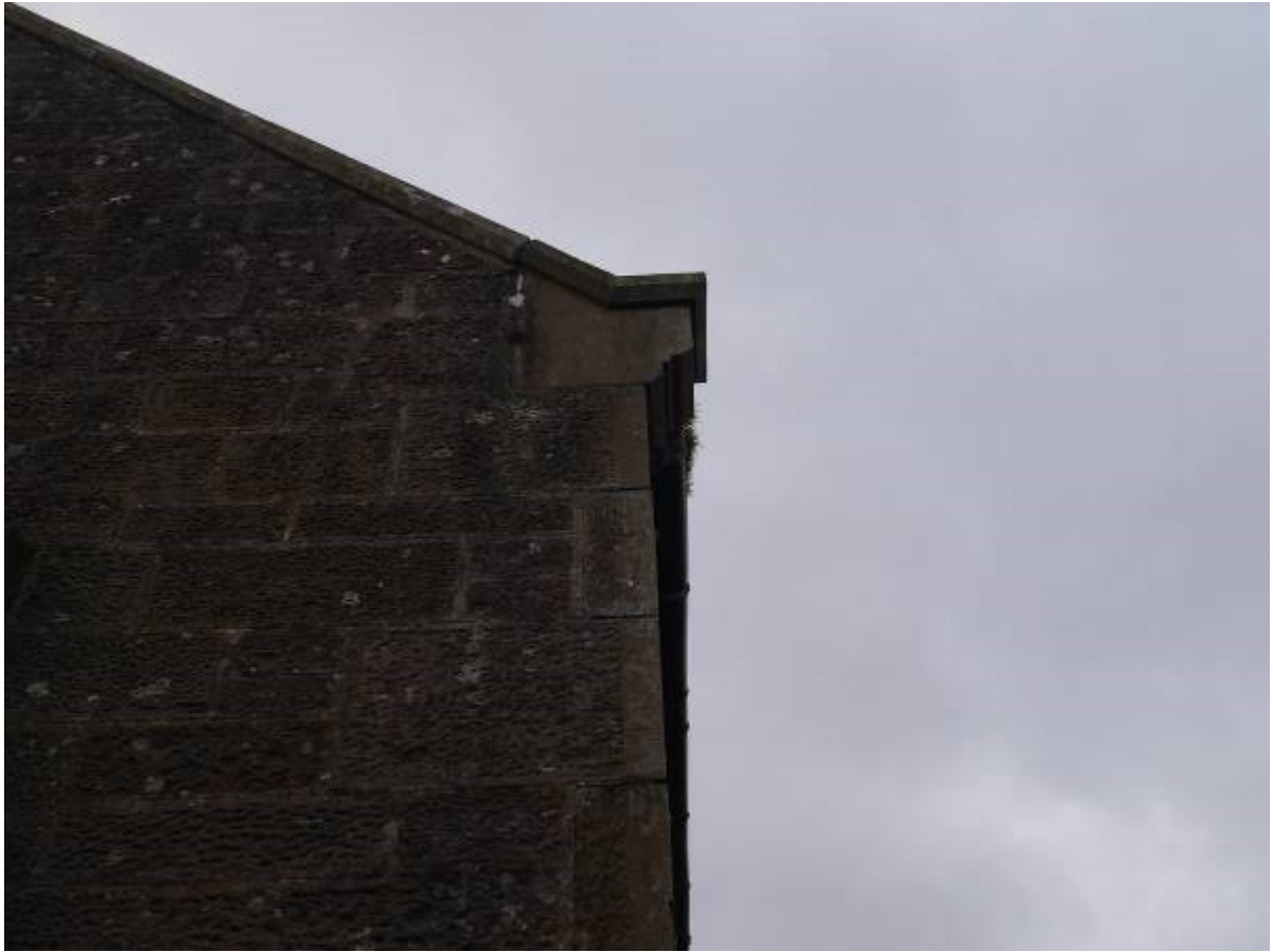
Illustration 41- Sculpted stone at wall head at Eastern end of Northern elevation of Building B
