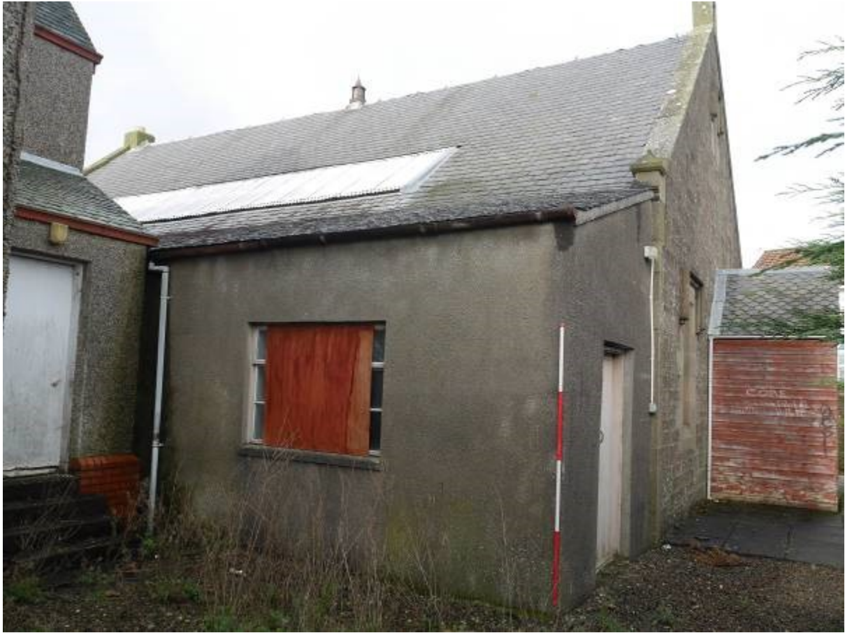
Illustration 44- Southern elevation (Eastern section) of Building B showing modern storeroom built against it and inserted skylights in slated roof
