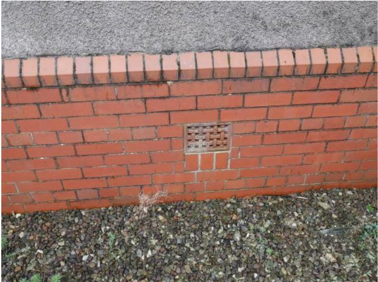
Illustration 18- Detail of decorative brick panel in brickwork at foot of Northern elevation of Eastern Transept
