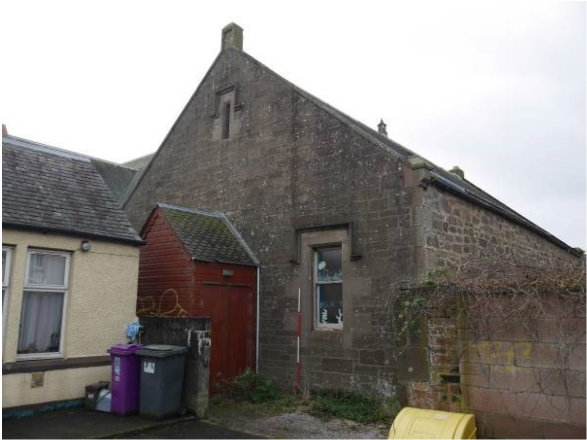
Illustration 42- Eastern elevation of Building B showing windows with decorative cornices, more recent wooden entrance hall also visible
