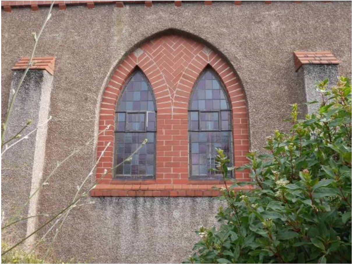
Illustration 8 - Detail of one of the windows in the Western elevation of the Nave (Building A)
