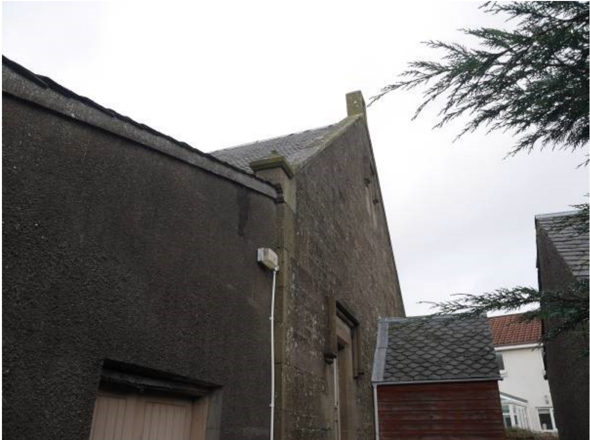
Illustration 43- Southern section of Eastern elevation of Building B showing junction with more recent storeroom, sculpted stone at wall head and window with decorative cornice
