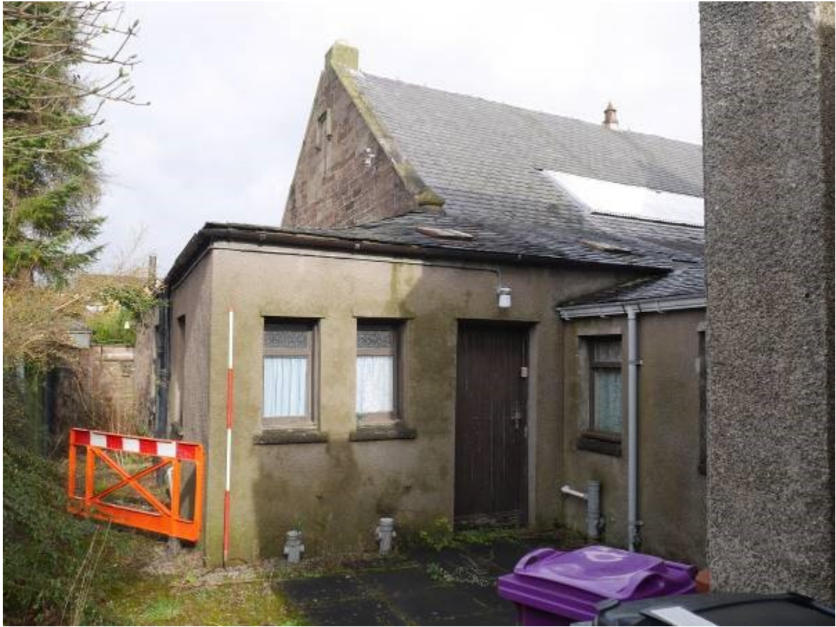
Illustration 45- Southern Elevation of Building B (Western section) showing toilet, kitchen and classroom built against it, surviving visible section of Western elevation also visible
