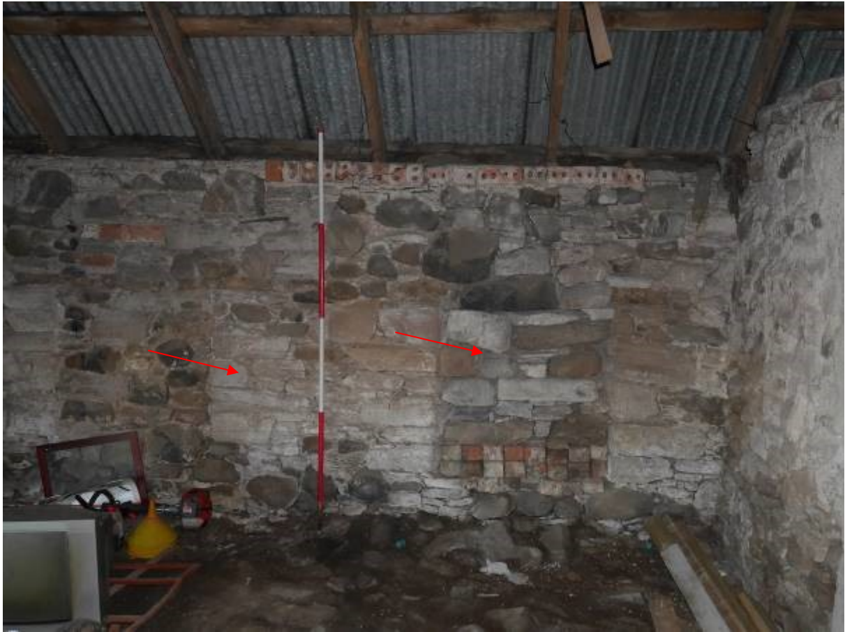
Illustration 21- Eastern elevation of Steading 2 showing two blocked windows (marked with red arrows)
