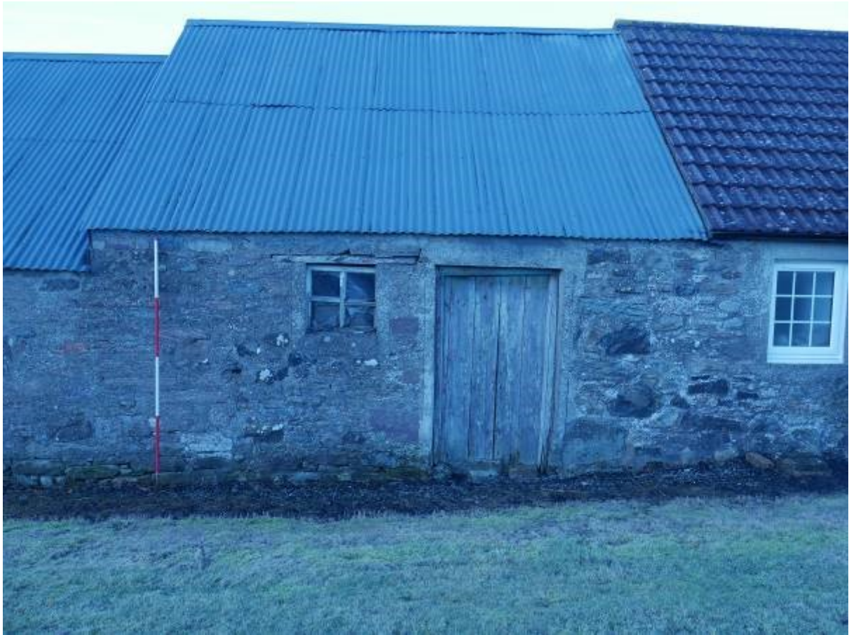
Illustration 15- Detail of Eastern elevation showing entrance into Steading 1 and slightly higher roof line
