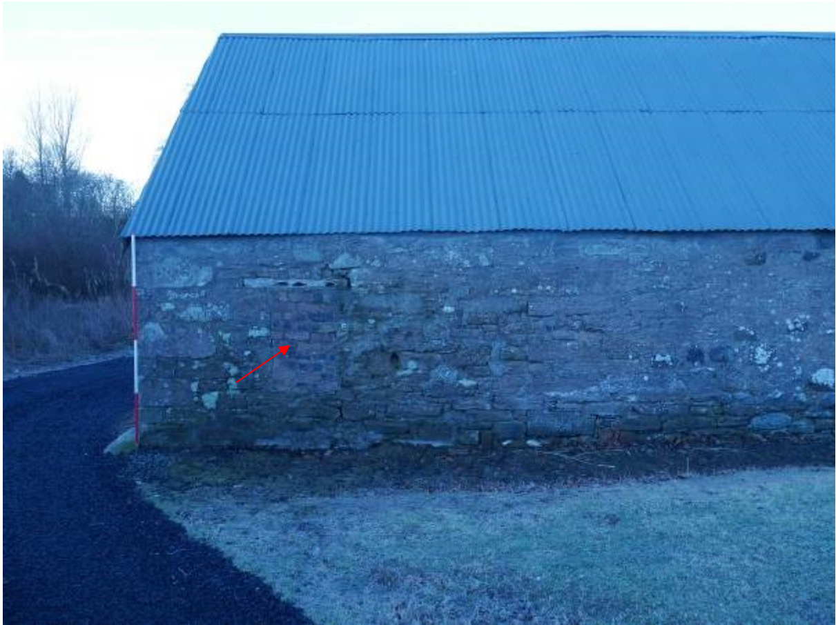
Illustration 13- Southern end of Eastern elevation showing blocked window (red arrow)
