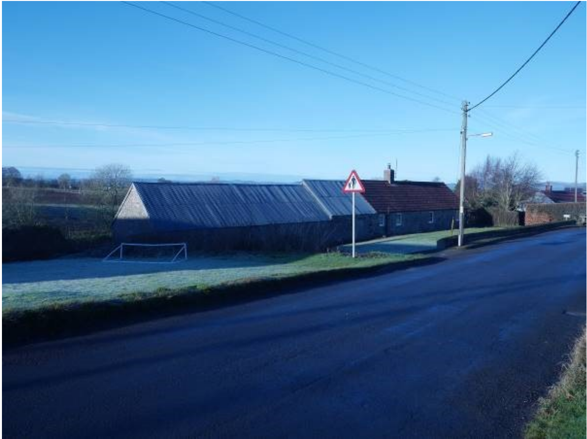
Illustration 6- The Cottage, Collace from the South East building surveyed has tin roof
