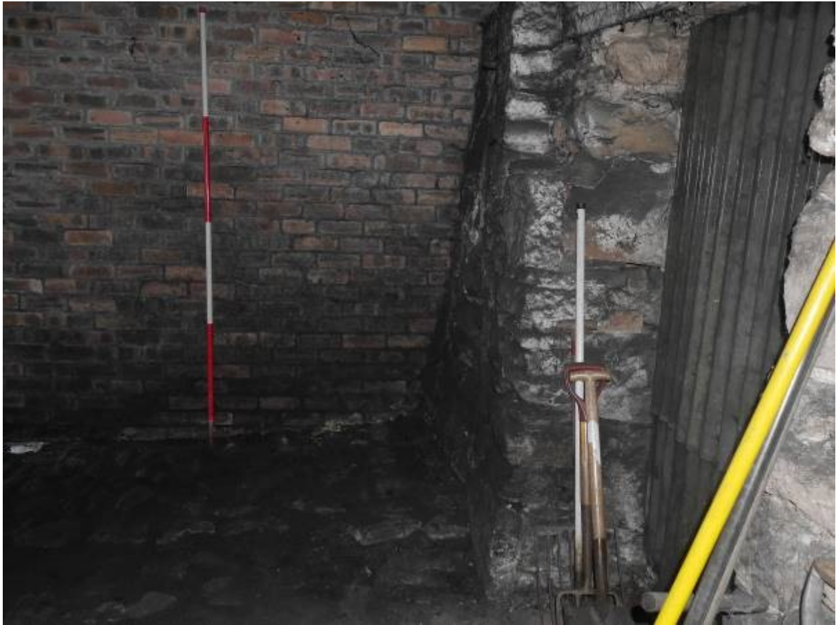
Illustration 16- Northern internal elevation to Steading 1 showing brick wall, sloping face on wall of Eastern elevation also visible
