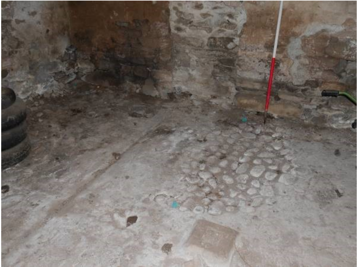
Illustration 29- Internal floor of Steading 3 showing cobbling, drain and one of the socketed stones in the floor
