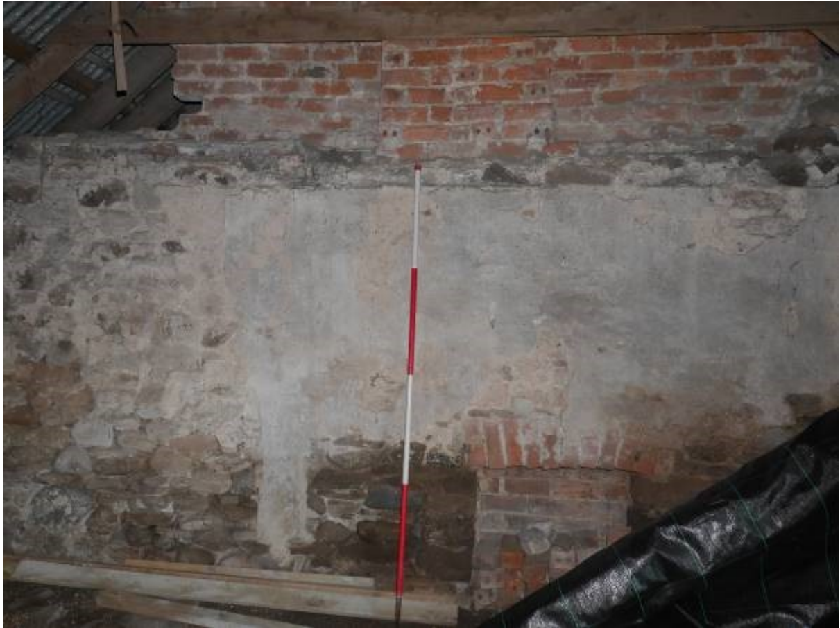
Illustration 23- Southern internal elevation for Steading 2 showing fireplace with brick arch and brick support for roof
