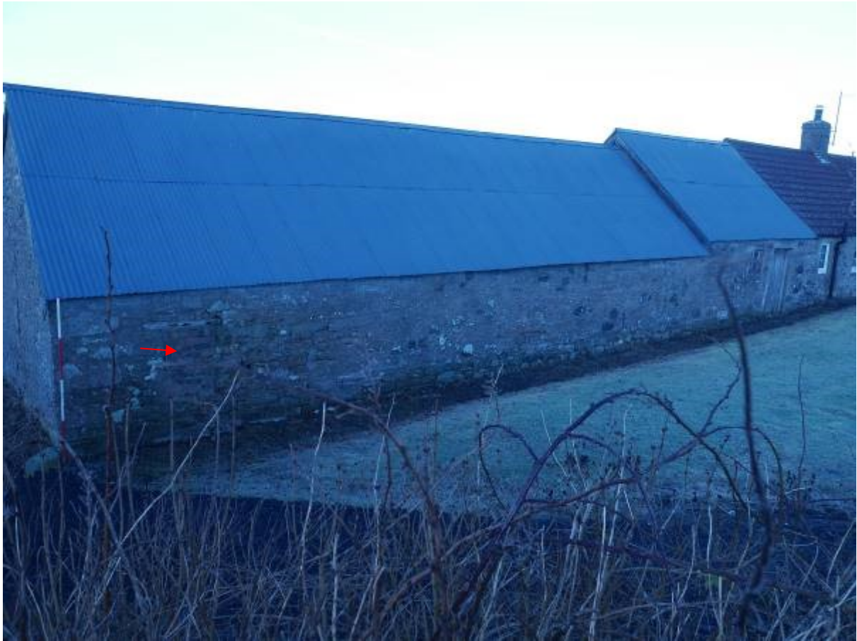
Illustration 12- Eastern elevation looking North West (blocked window marked with red arrows)
