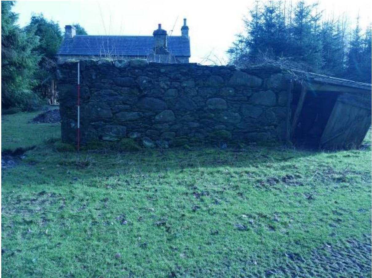
Illustration 22 - Western elevation to Building 3, collapsing Building 4 visible on right
