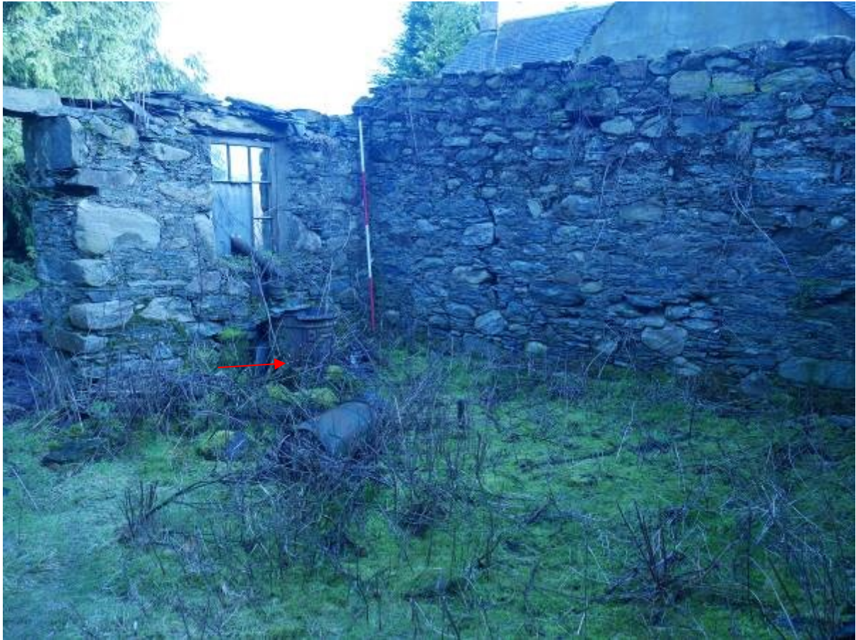
Illustration 28 – Internal Western and Southern elevations of Room 3b in Building 3 showing cast iron stove or boiler (red arrow)
