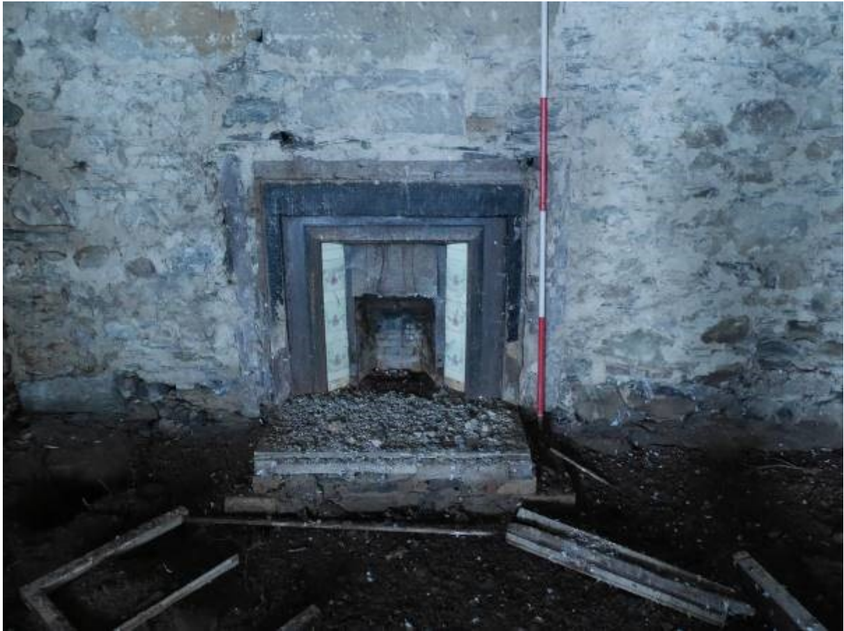
Illustration 13- Fireplace at ground floor level in Northern elevation of Building 1 with decorated tiles
