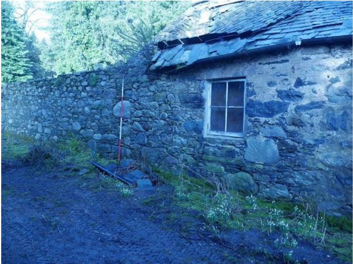
Illustration 20 – Butt joint between Buildings 2 and 3 visible in Southern elevation (to the right of the scale)
