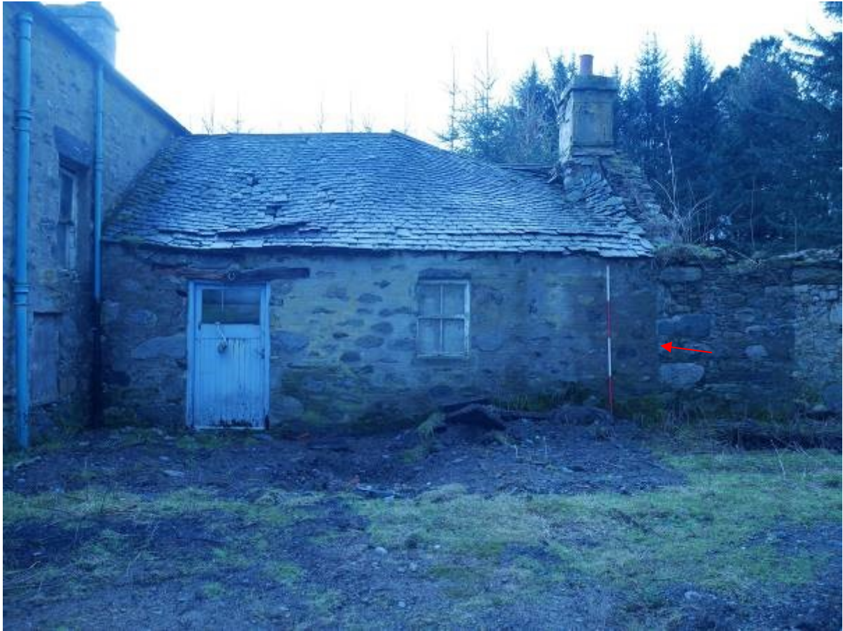
Illustration 17 - Northern elevation of Building 2, note straight joint between the Western end of Building 2 and the Eastern end of Building 3 (red arrow)
