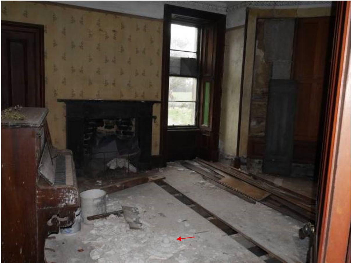
Illustration 21 - Building A Room 4 (Eastern living room) looking East showing collapsed ceiling moulding on floor (red arrow)
