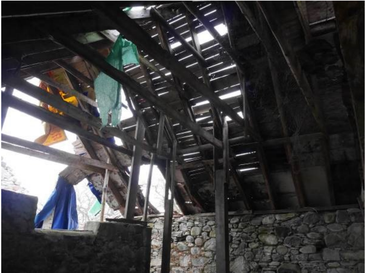
Illustration 41 - Building B internal view of surviving section of wooden roof supports for slate roof
