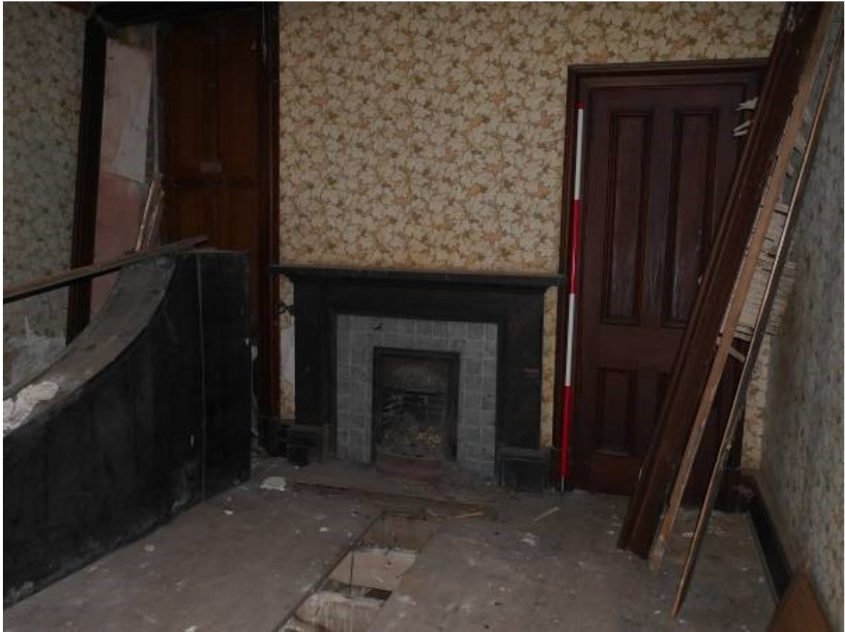
Illustration 24 - Building A Room 5 (Western living room) showing fireplace and cupboard in Western wall
