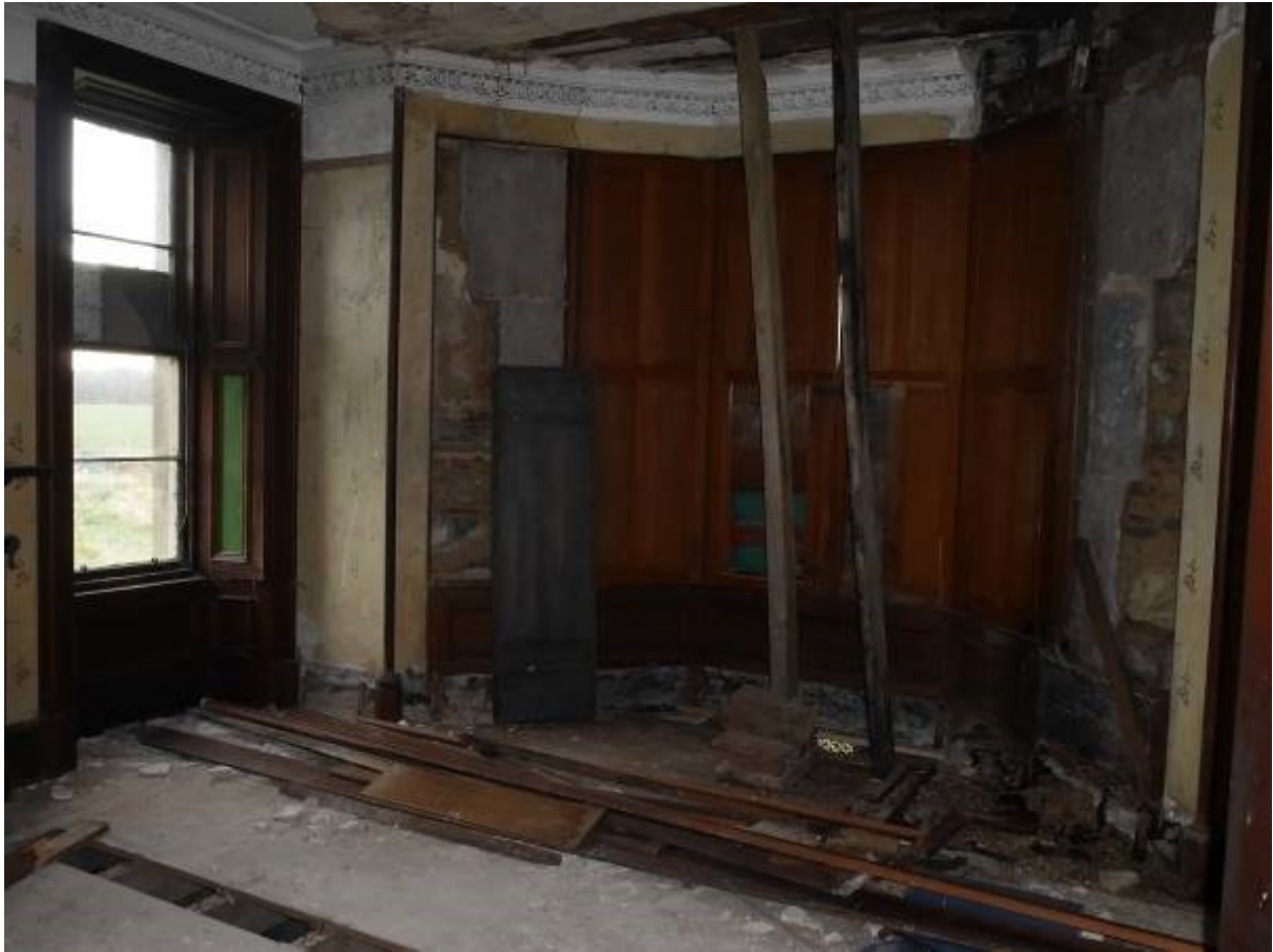
Illustration 22 - Building A Room 4 looking South showing interior of bay window and decorative moulding around ceiling
