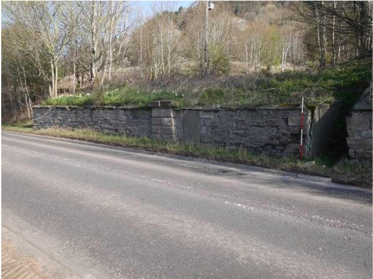
Illustration 24 - General view of raised revetted garden directly across the road from the tollhouse, flight of steps to right of scale, pillar and blocked alcove also visible in wall.
