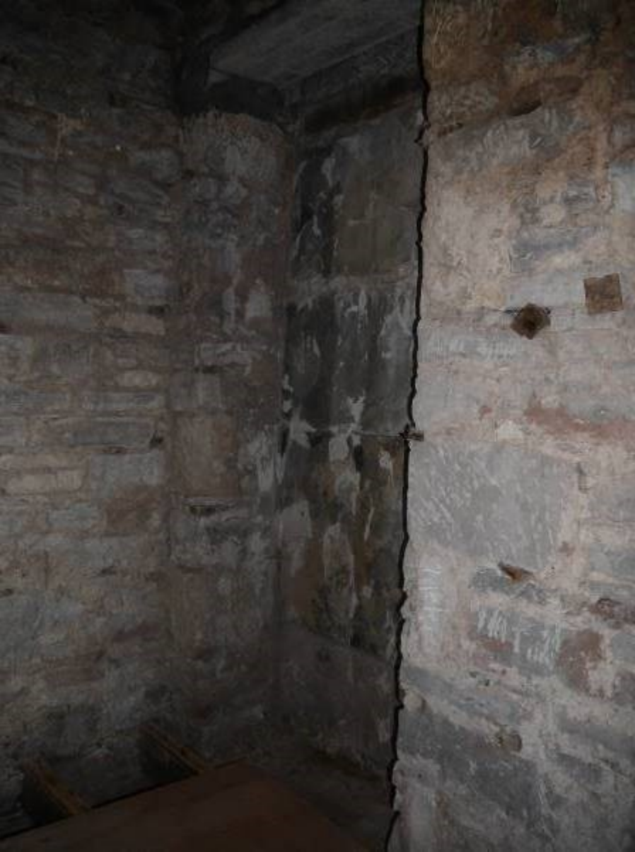
Illustration 19 – Wall recess behind front alcove for table of dues in North Eastern internal elevation of tollhouse
