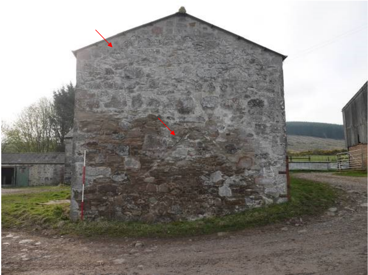
Illustration 36 – North Western elevation of Building 6, roof raggle and slight raising of gable marked with red arrows
