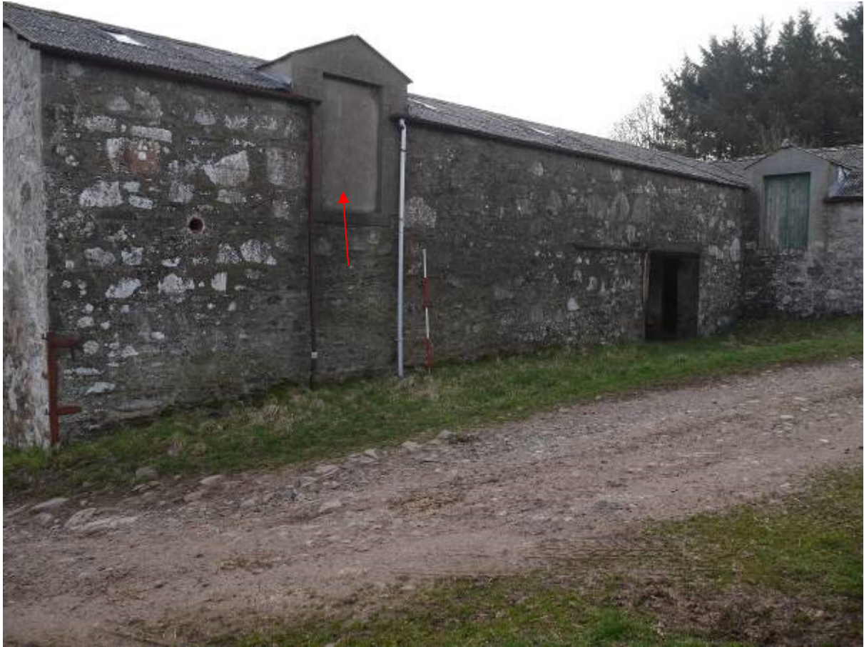
Illustration 37 – South Western elevation of Building 6 with blocked door at first floor level marked with red arrow
