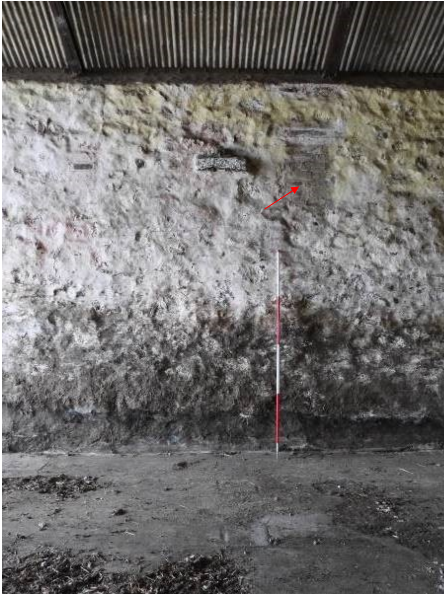
Illustration 29 - Internal support for pulley? And blocked hole for drive shaft for water wheel (marked with red arrow) in internal South Eastern elevation of Building 4
