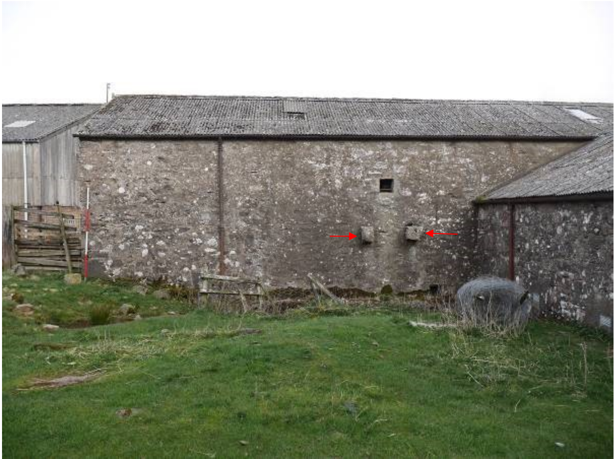
Illustration 26 – South Western elevation to Building 4 water wheel supports marked with red arrows, hole for drive shaft visible above
