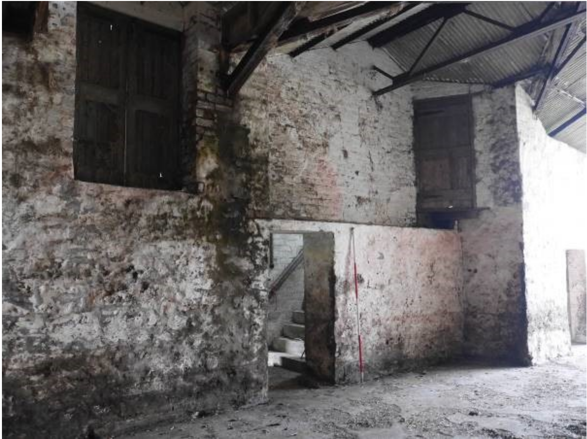
Illustration 30 – Doorway providing access to stairs to upper floor of Building 5 in internal North Western elevation of Building 4
