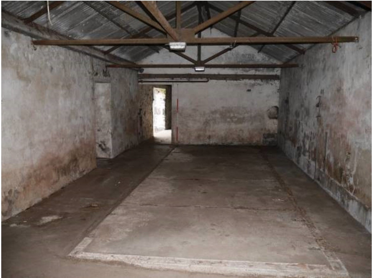
Illustration 17 – Room b in Building 2 looking North East showing animal pen foundations in floor
