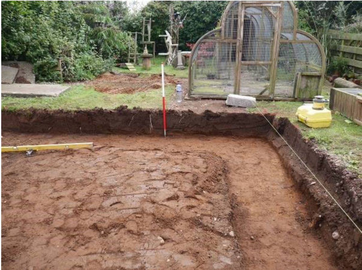
Illustration 8- Eastern foundation trench totally excavated showing Context 200 lying above natural sand 201 looking South East.
