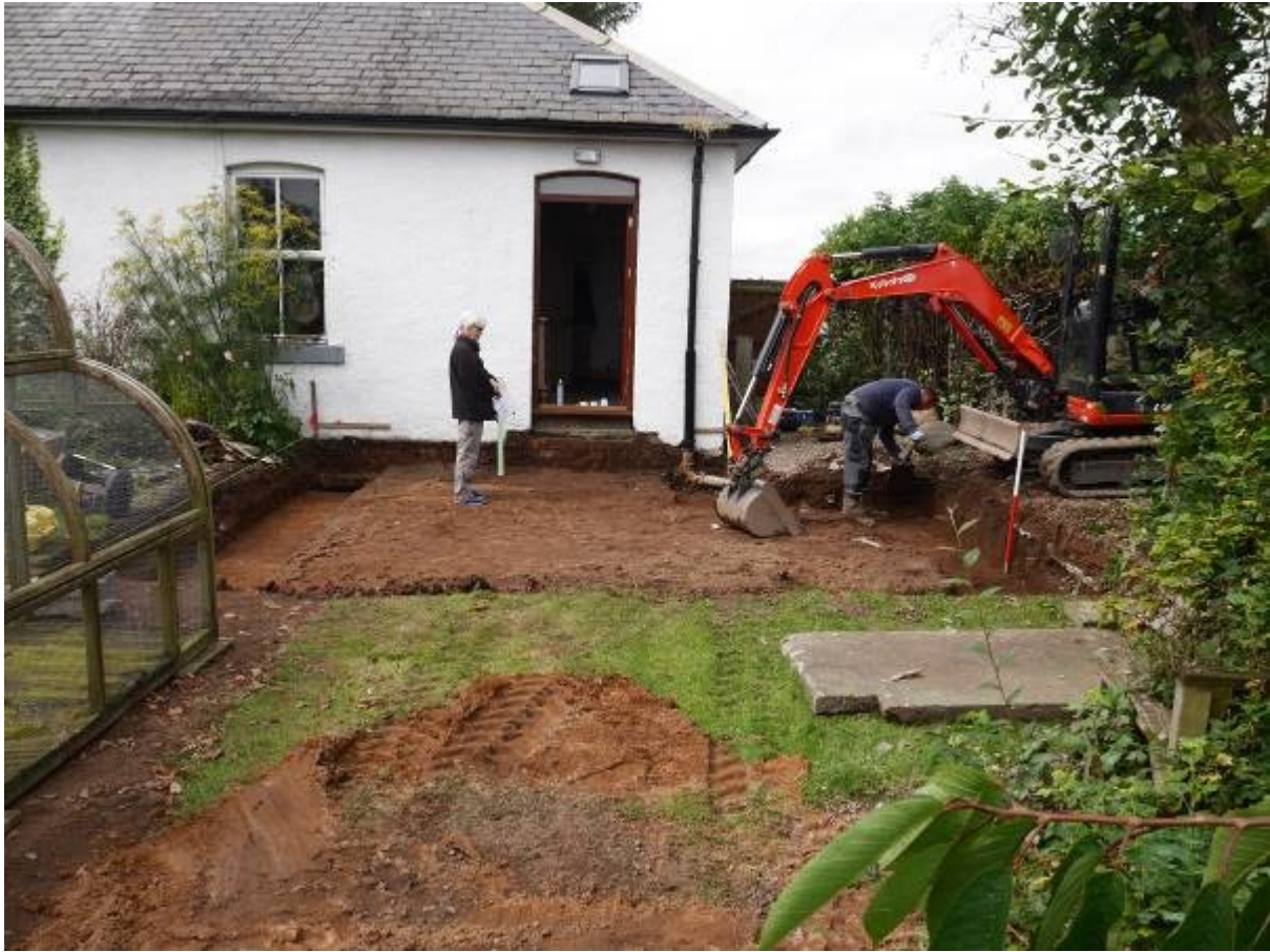
Illustration 10- General view of totally excavated footprint and foundation trenches for new extension.
