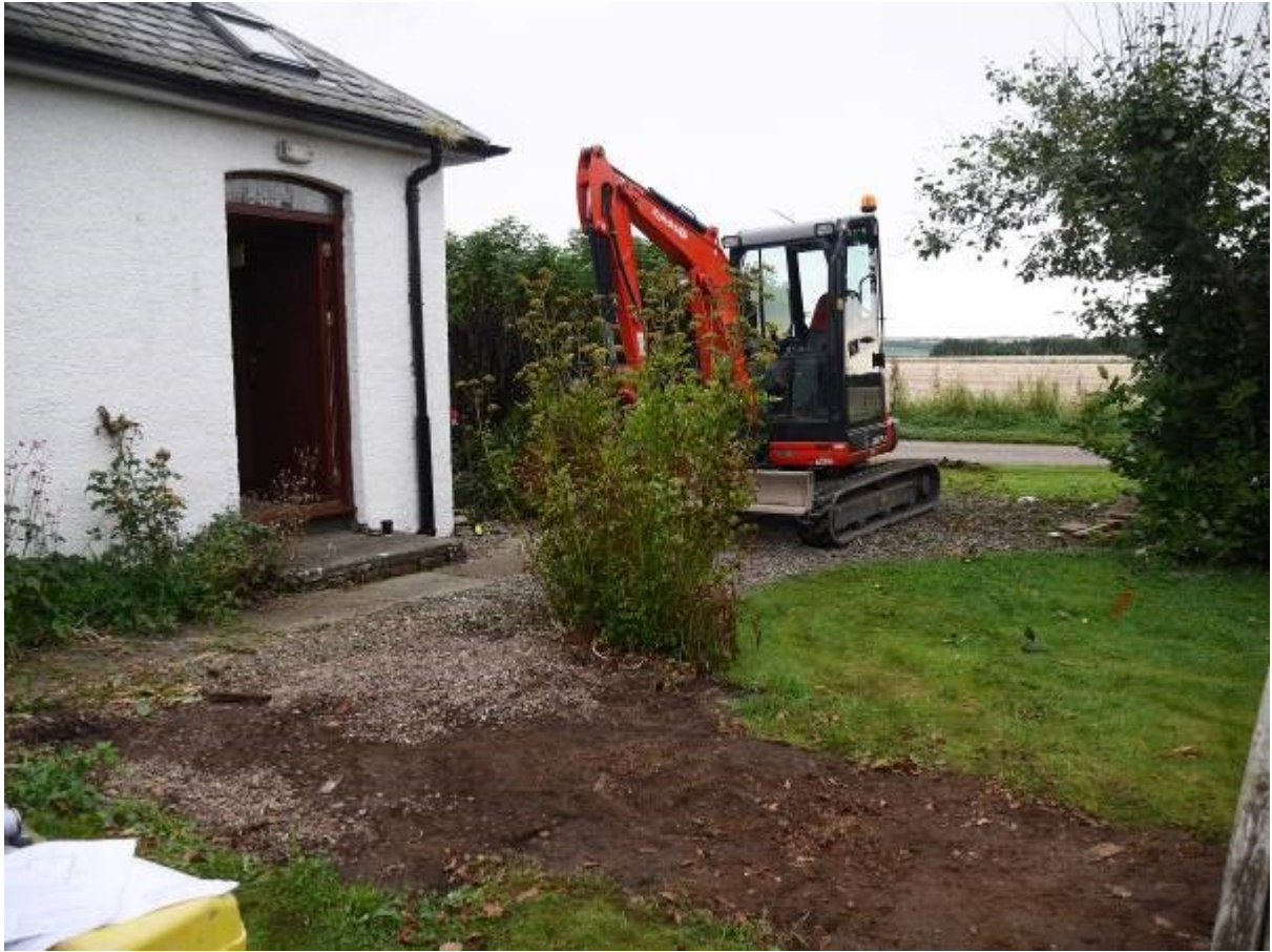
Illustration 5- General view of site of new extension prior to excavation looking North.
