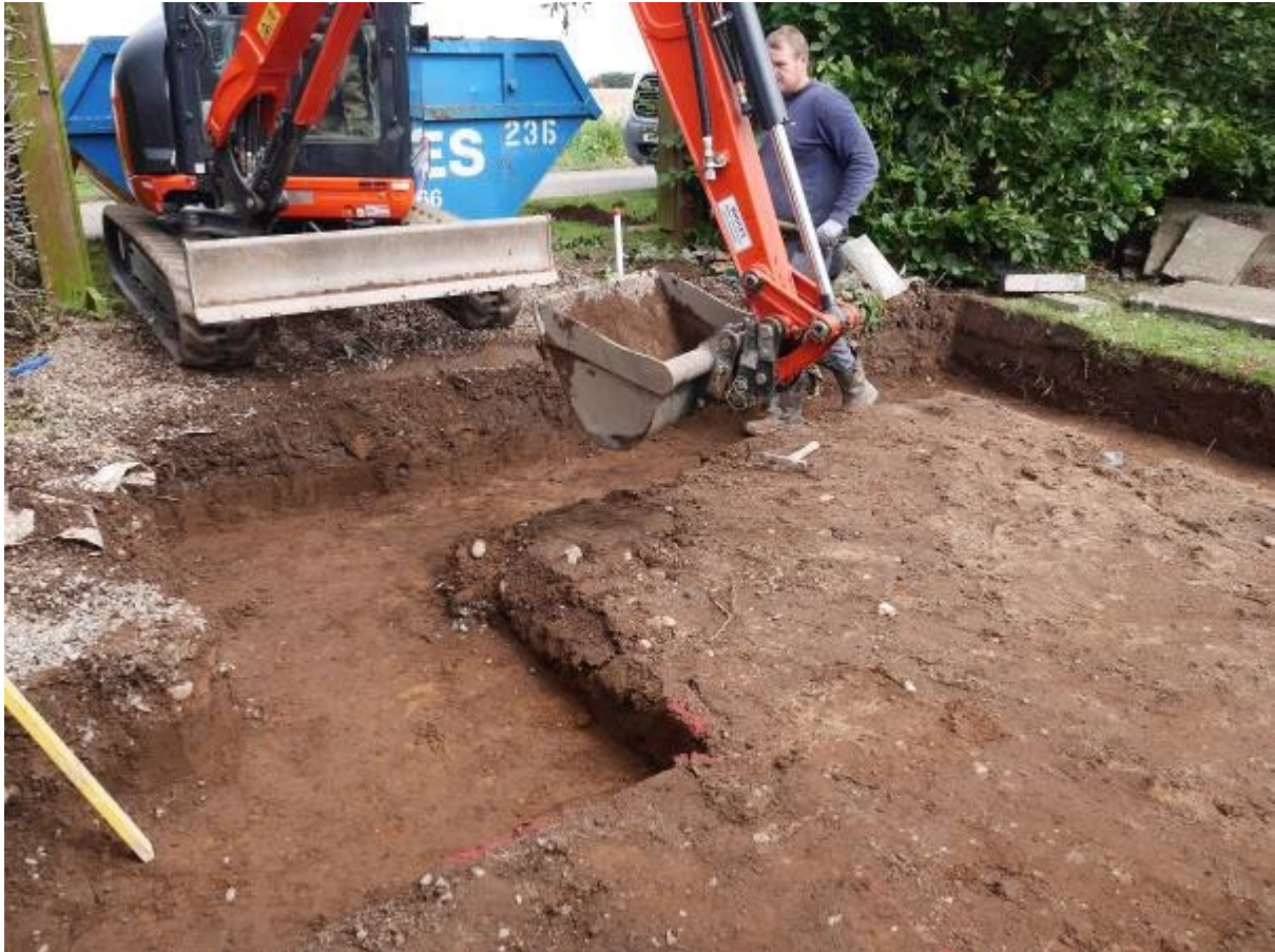
Illustration 9- Northern foundation trench totally excavated showing Context 200 lying above natural sand 201, gravel and plastic 204 visible in section.
