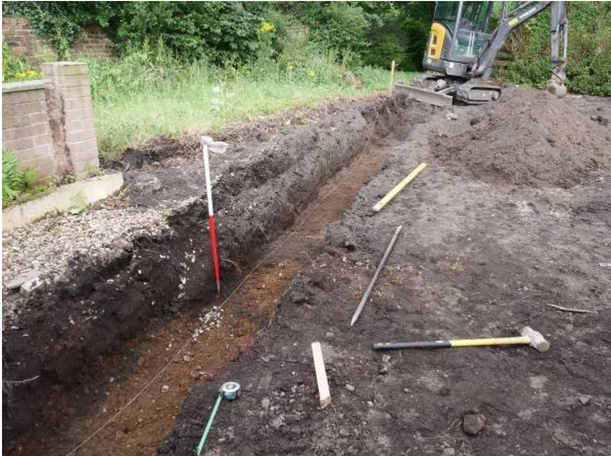
Illustration 7 Trench A looking West showing appearance of soil 103, junction of natural gravel 102 and beginning of soil 103 visible just above scale
