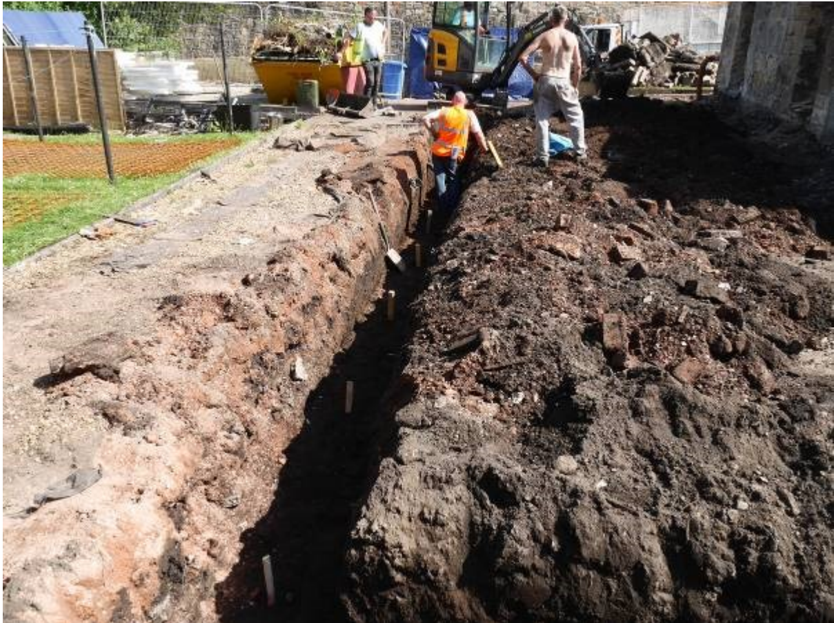
Illustration 10 view along trench E looking South East showing made up ground 100 overlying Context 103 to formation level.
