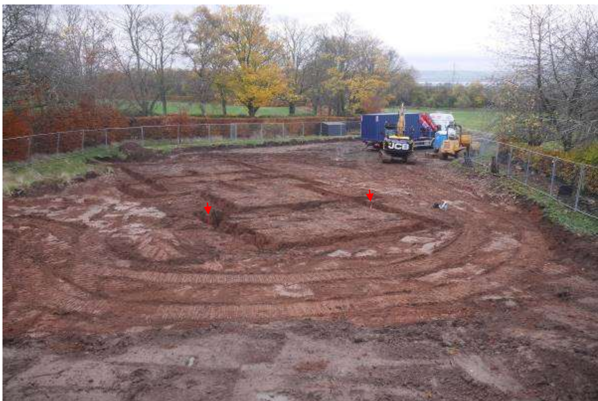
Illustration 11- General view of excavated foundation trenches for new house looking South (River Tay just visible at top of photograph), line of cut feature 102 is marked with ranging rods (red arrows).
