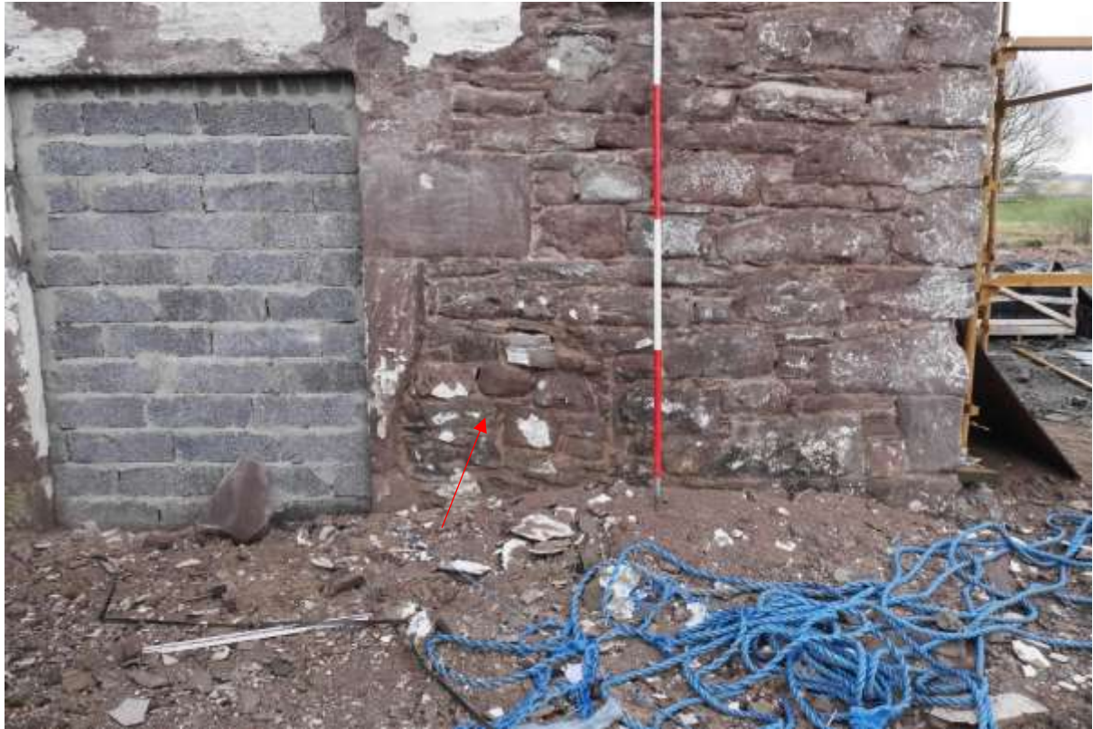
Illustration 15- Detail view of blocked circular hole in North Eastern elevation (red arrow).
