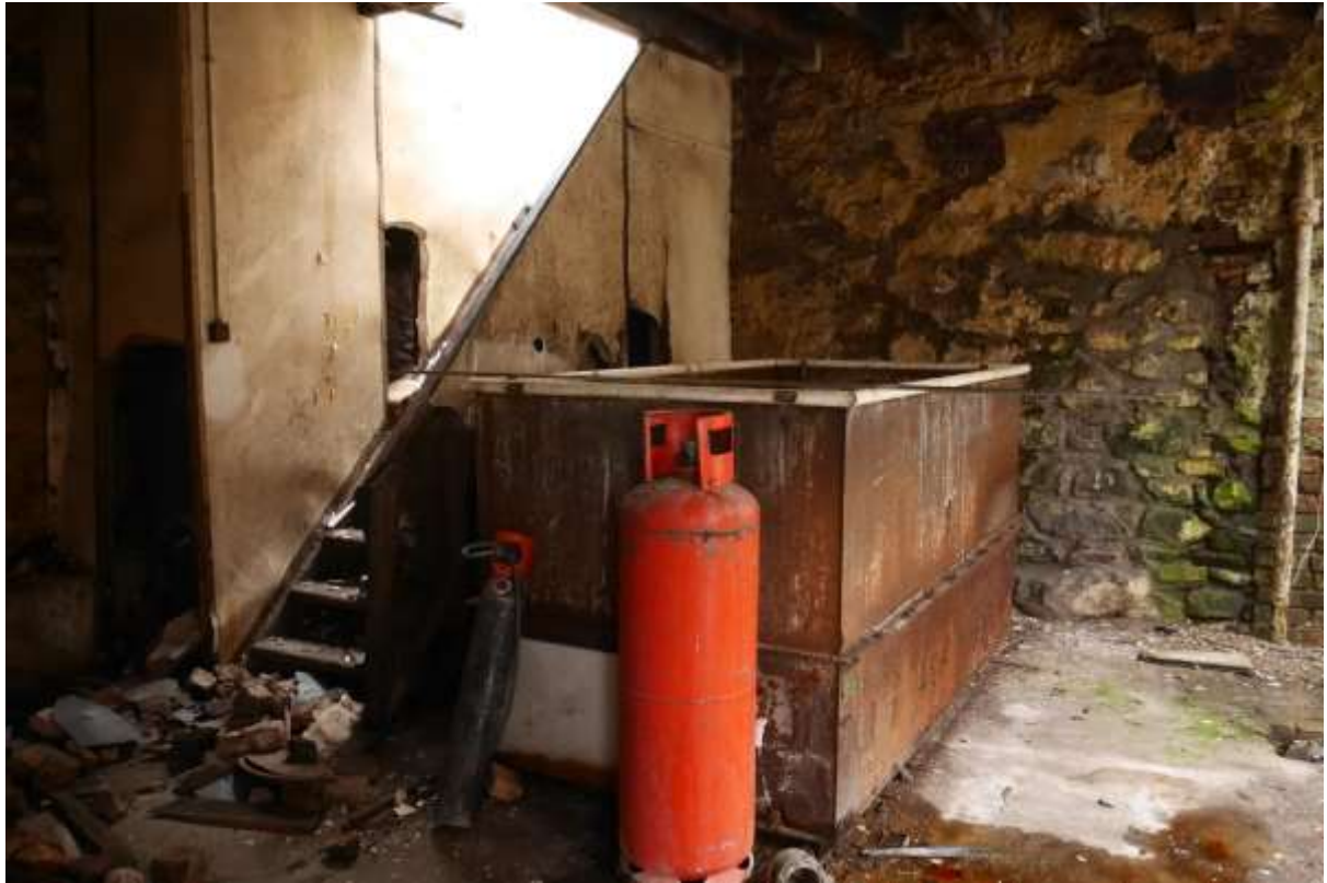
Illustration 23- Interior of small building showing cast iron tank and flight of stairs to door access from road.
