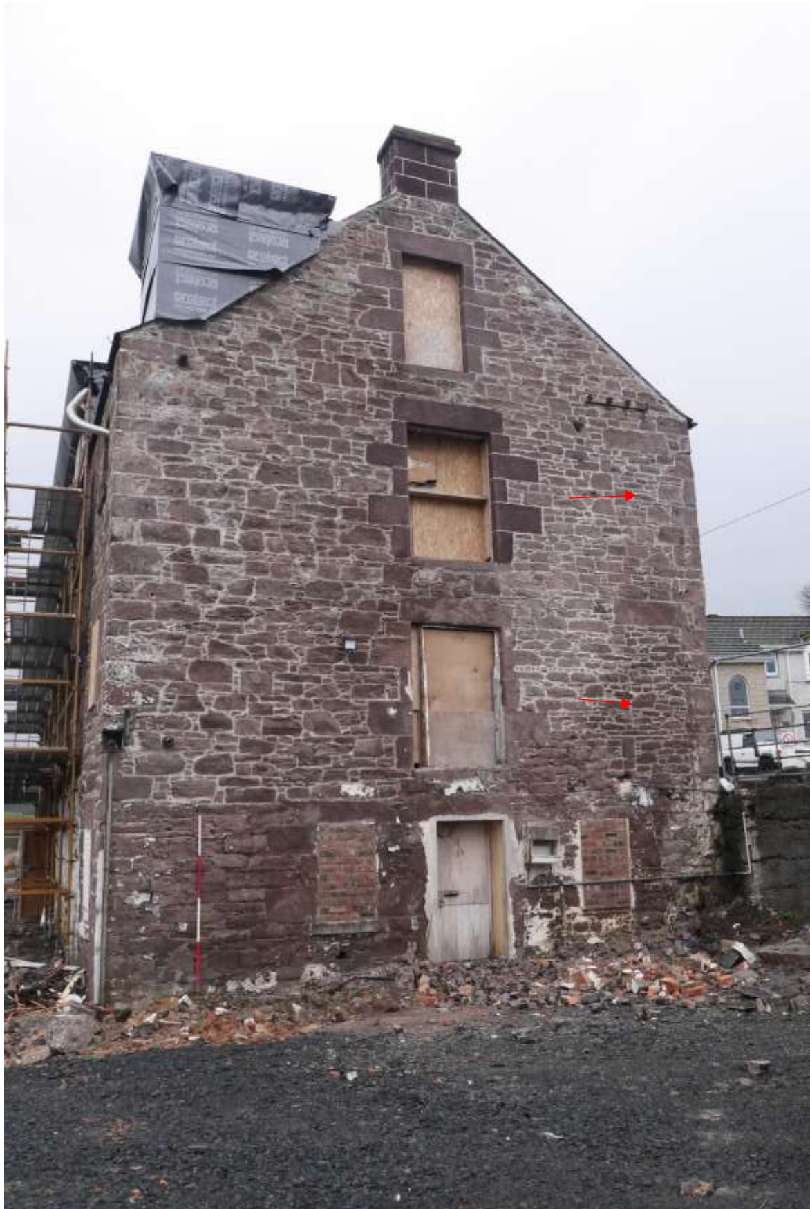
Illustration 12- South Eastern external elevation of building (red arrows show dummy windows)
