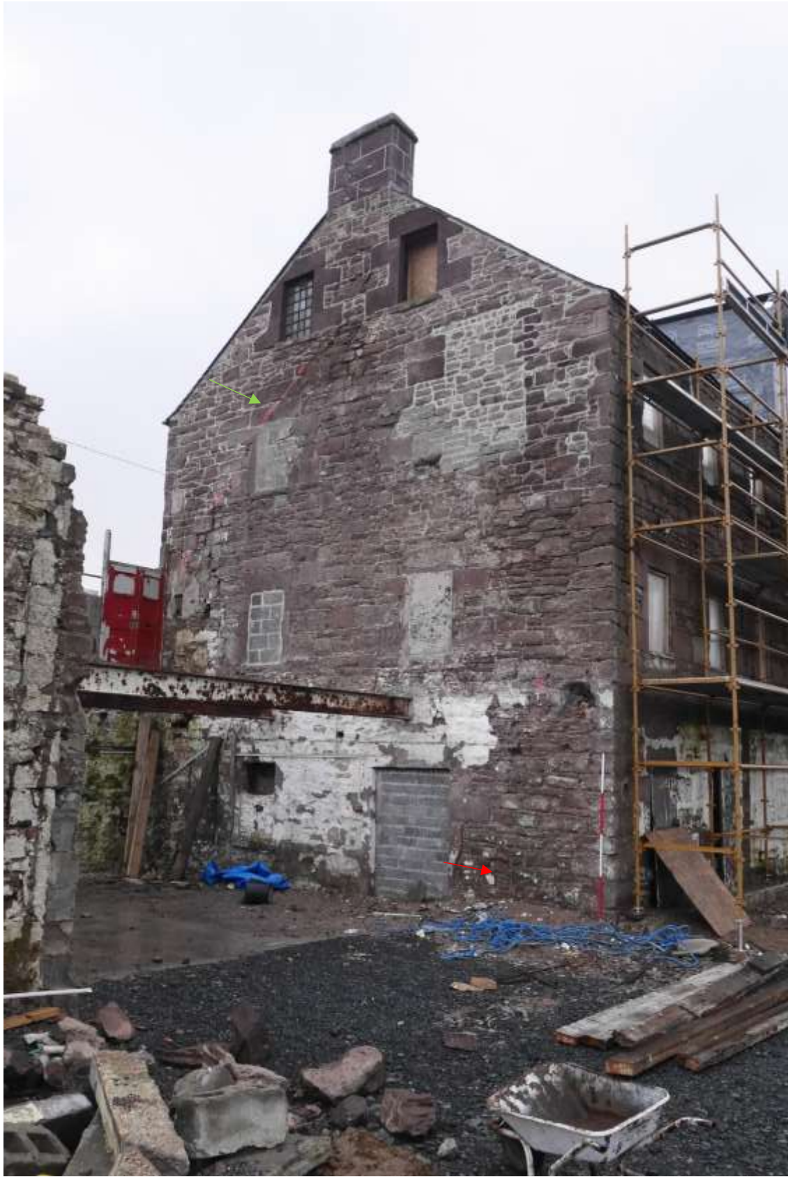
Illustration 14- North Eastern elevation of mill building, red arrow shows position of blocked circular hole, green arrow shows former roof line of adjoining building.
