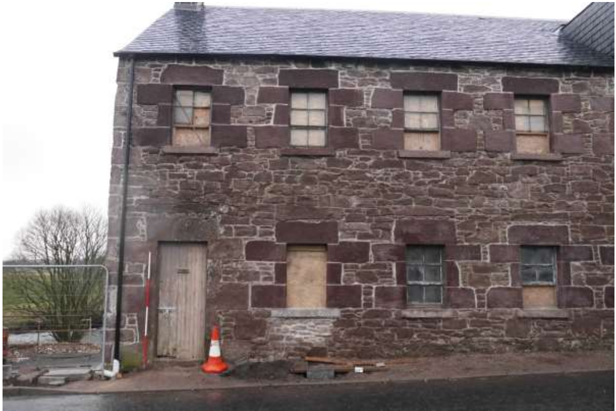
Illustration 17- Southern end of North Eastern elevation showing windows defined by sandstone blocks.
