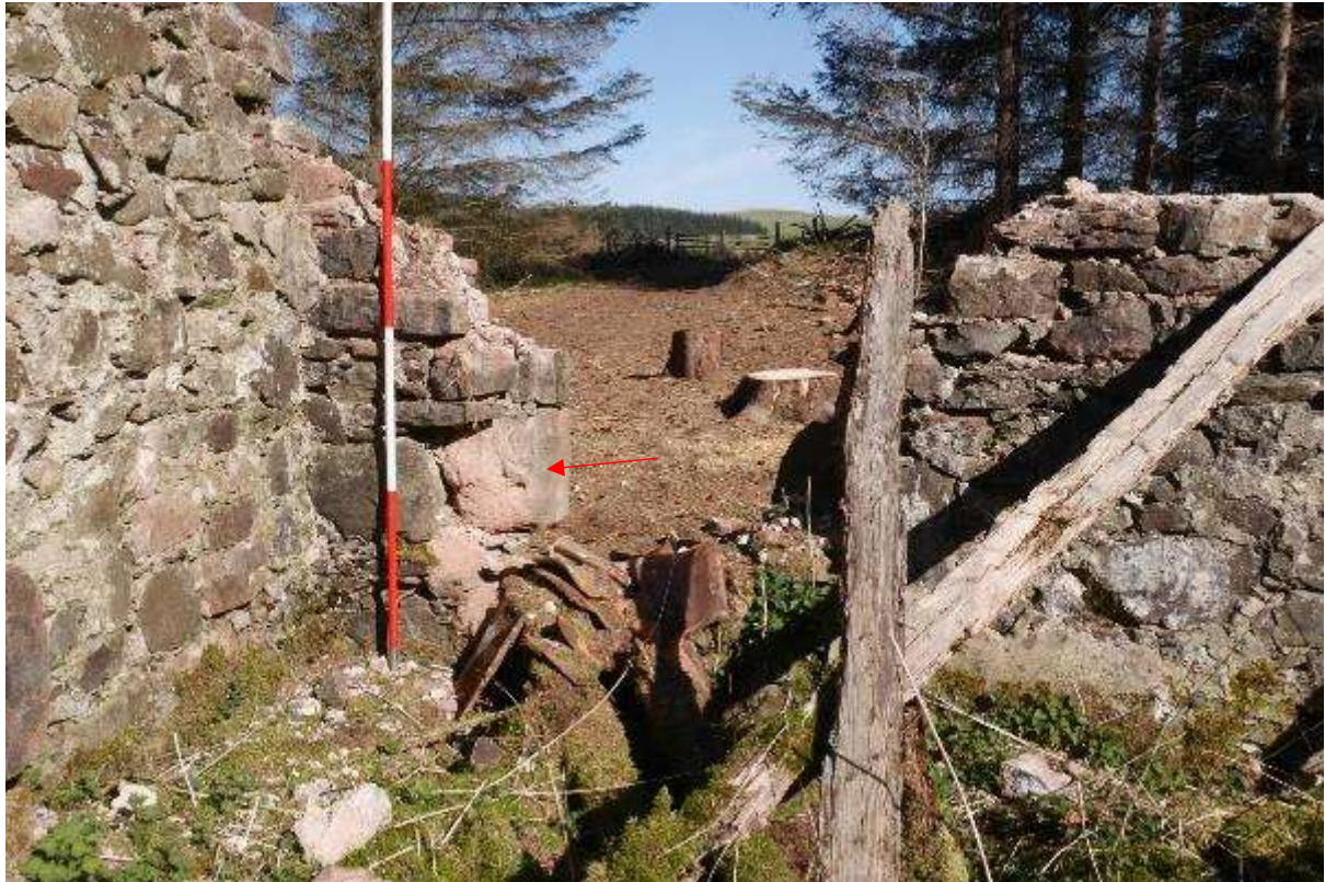
Illustration 34- Window at Western end of internal Southern elevation of Room A, red arrow shows other side of reused architectural fragment (no 8), collapsed ceramic roof tiles also visible.
