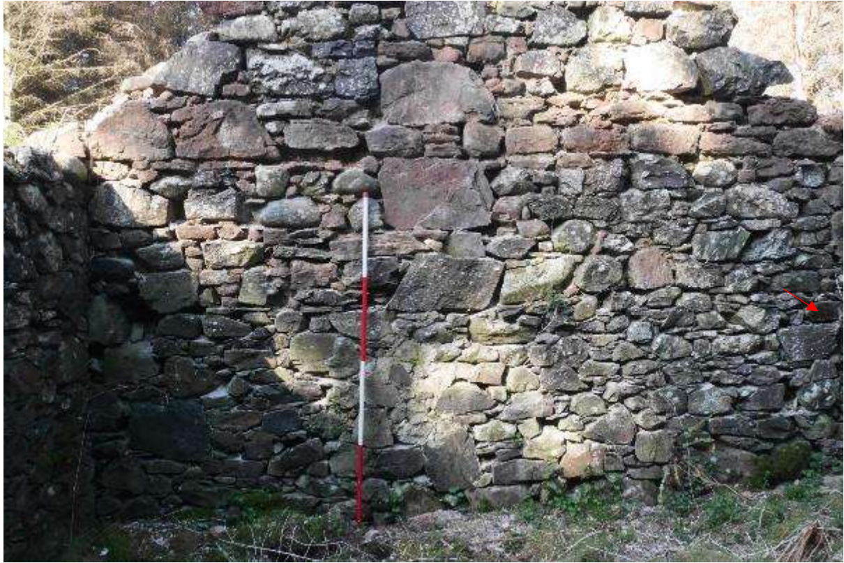
Illustration 39- Western internal elevation of Room B showing flat stones marking line of chimney for fireplace in Room A, red arrow indicates stone with incised lines from sharpening of metal object (no 9).
