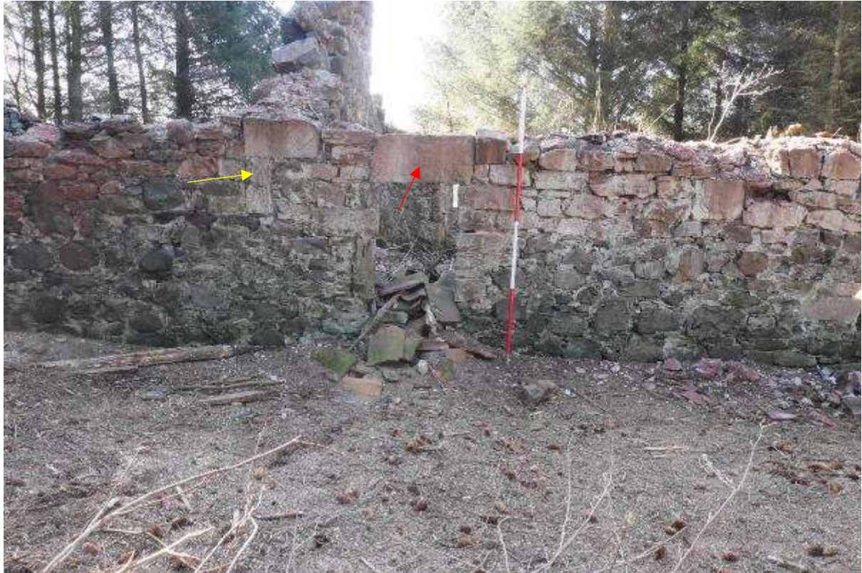
Illustration 25- Window in Room A in Northern elevation of building with collapsed ceramic roof tiles visible, yellow arrow shows straight joint between rooms A and B with tool marked stones (no 6), red arrow indicates window lintel with pecked toolmarks (no 7).
