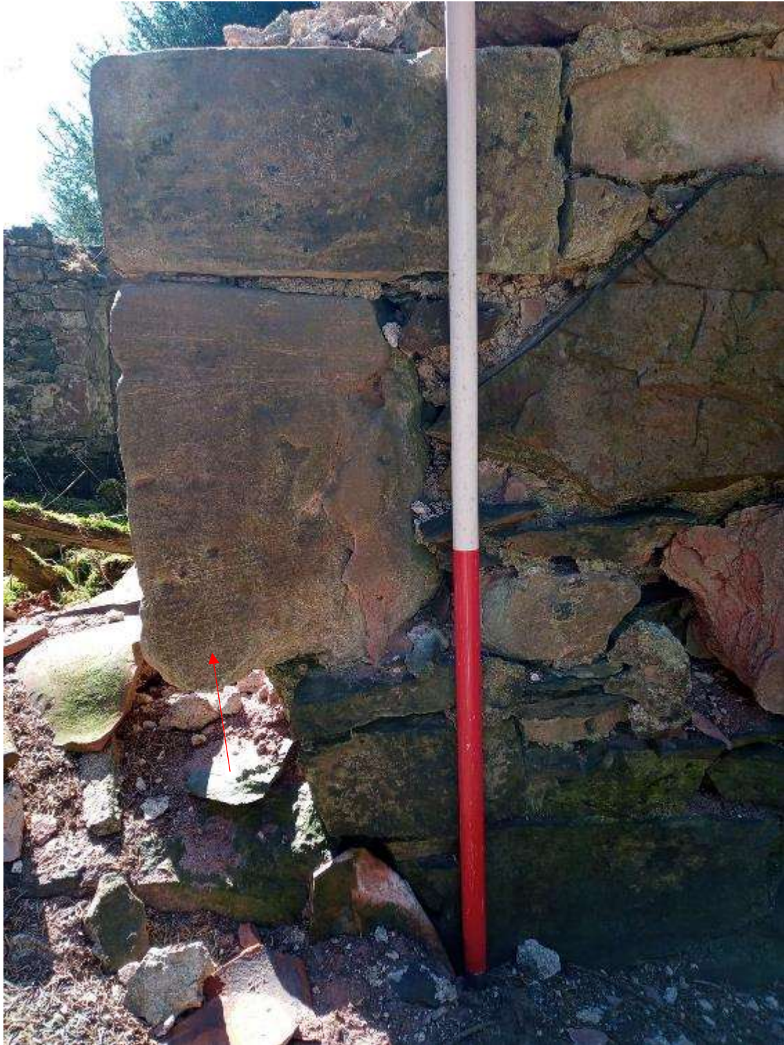
Illustration 30- Detail view of reused architectural fragment in red sandstone (no 8) in window in Room A in Northern elevation of building.
