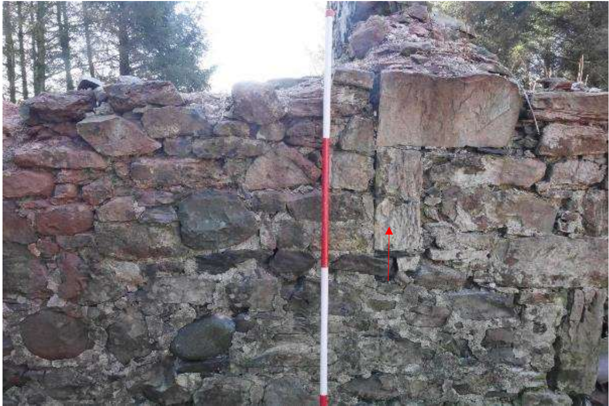
Illustration 26- Straight joint between Rooms A and B visible in Northern elevation, red arrow shows tool marked pieces of yellow sandstone (no 6).
