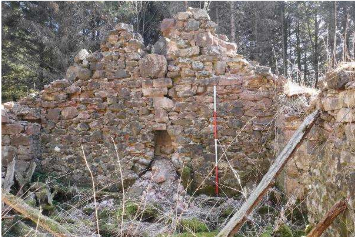
Illustration 37- Internal Eastern elevation of Room A showing central fireplace with angled access to chimney.
