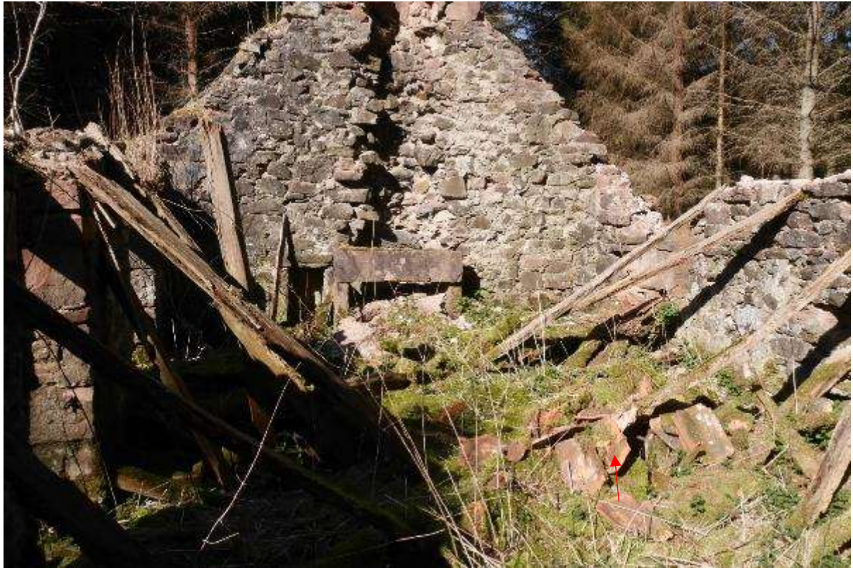
Illustration 32- General view of interior of Room A looking West showing collapsed roof timbers and ceramic roof tiles (red arrow).
