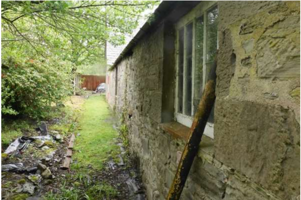
Illustration 21- Southern end of Western external elevation of Building 1 showing window of similar design to those in its external Eastern elevation.
