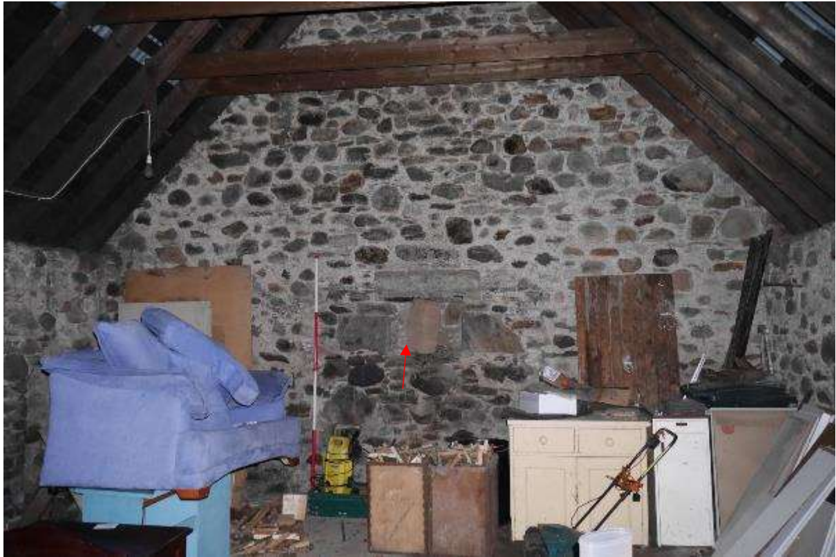
Illustration 11- North facing internal elevation of Building 1 showing hearth/fireplace in wall (red arrow).
