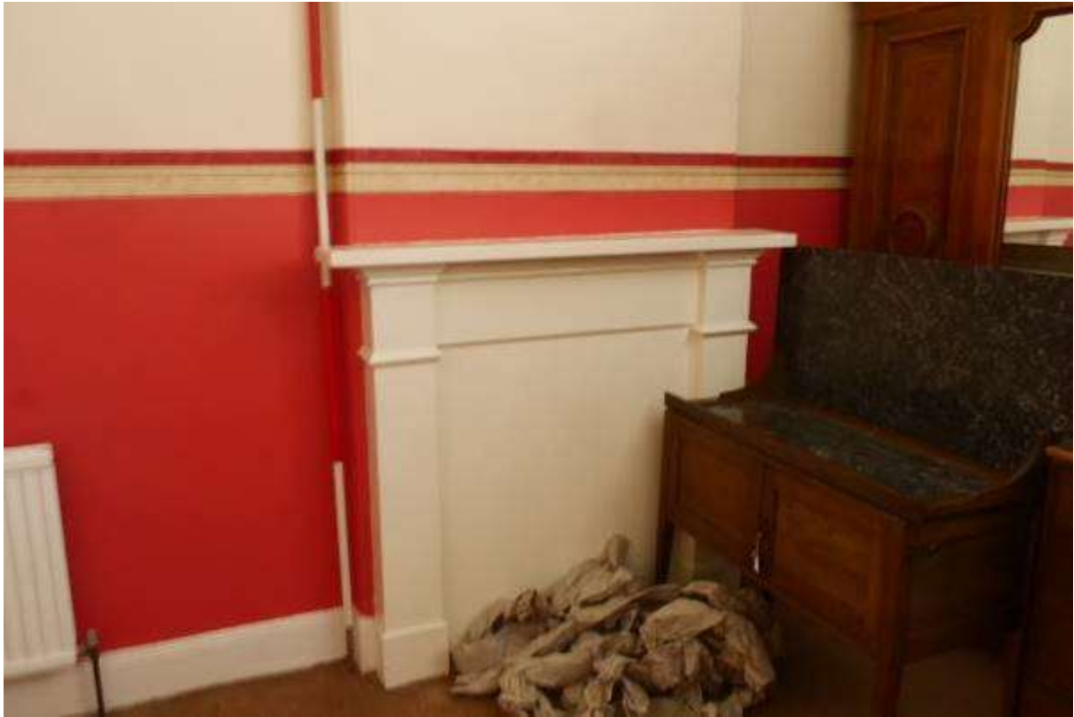
Illustration 64- Internal North Western elevation of Room 7 showing blocked fireplace. It is proposed to remove part of this wall.
