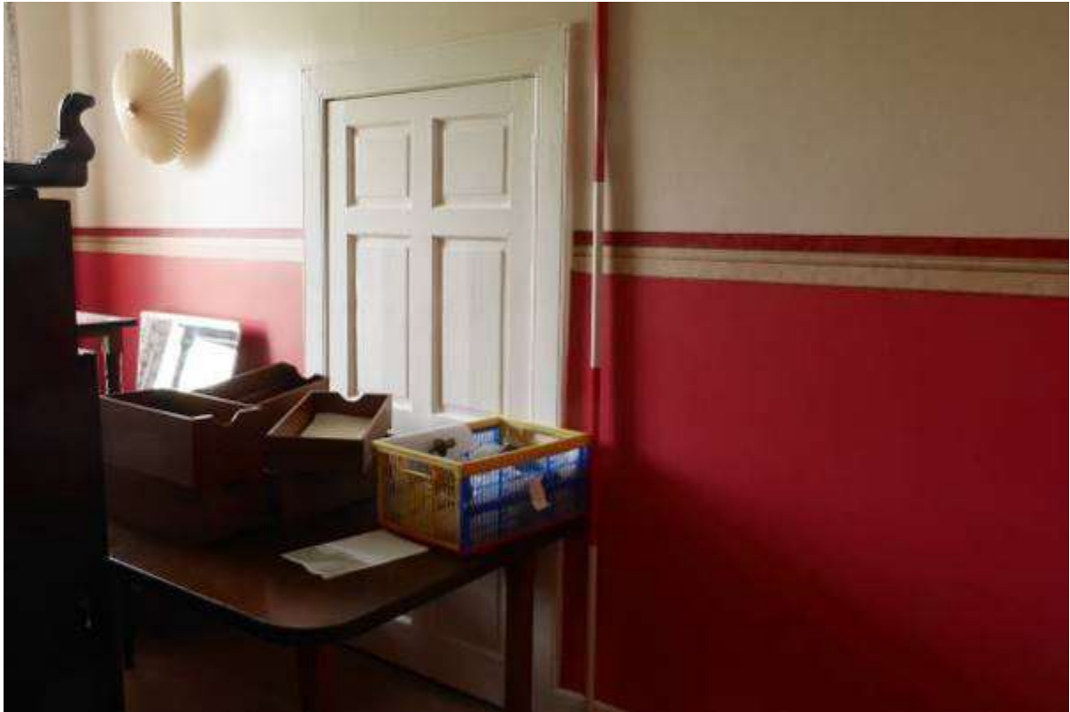
Illustration 62- Internal South Eastern elevation of Room 7 showing cupboard. It is proposed to make alterations to this elevation.
