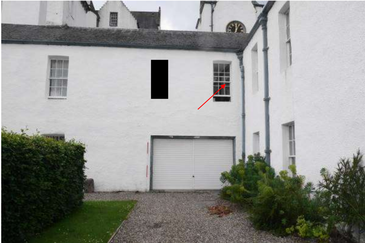
Illustration 96- Garage door (19) in external South Western facing elevation of South East Wing. It is proposed to remove the door. A new window will be inserted (black rectangle) and the window arrowed will have its sill lowered for a doorway access into a new turret, a new doorway will also be formed in the right-hand wall between the last window and the corner. The garage door is to be reduced in width and new glazed doors inserted.
