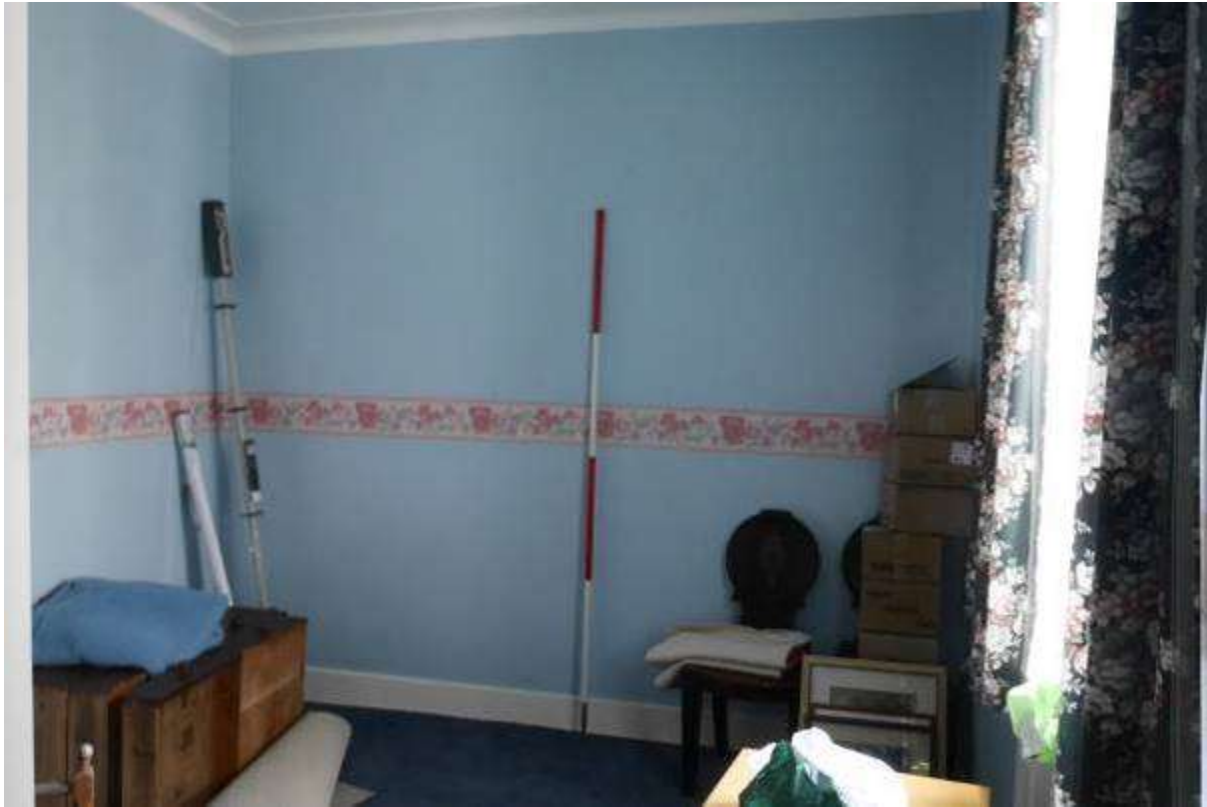
Illustration 66- Internal South Eastern elevation of Room 8. It is proposed to make alterations to this elevation and to open a new doorway into Sitting Room G18 (see Illustrations 33 and 67), through a pre-existing opening, blocked in the 1960s.
