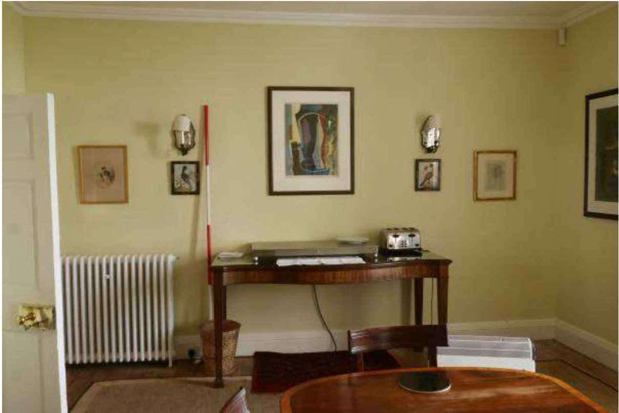
Illustration 83- North Western facing internal elevation of Room 13 (Dining Room). This wall is be removed and the door and wall to the left will also be removed.
