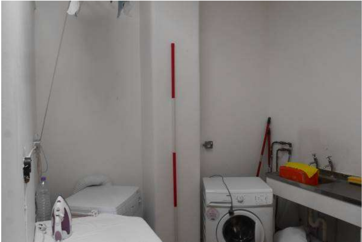
Illustration 90- General view of Utility Room (16) looking West. It is proposed to remove the drying room (to the left).
