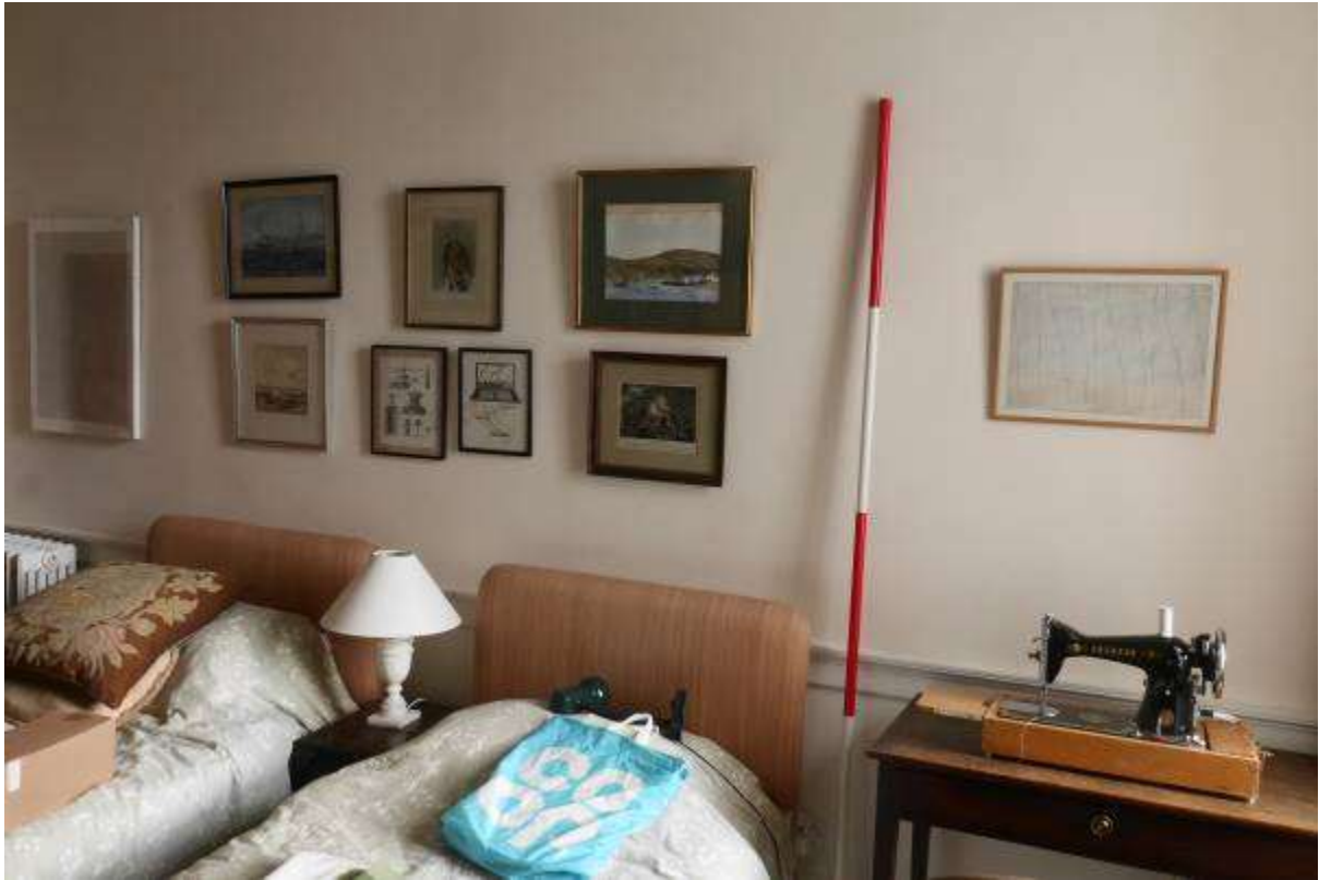
Illustration 116- Bedroom 25 North Western facing internal elevation, it is proposed to open a new doorway in this wall.
