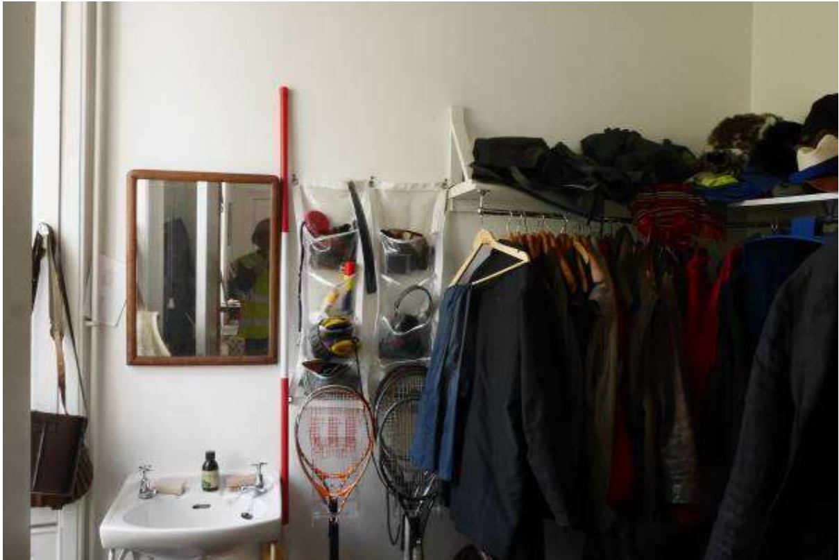
Illustration 77- South Eastern facing internal elevation of Room 11 (Cloak room). It is proposed to remove this wall and the one on the right, shared with the lavatory behind it.
