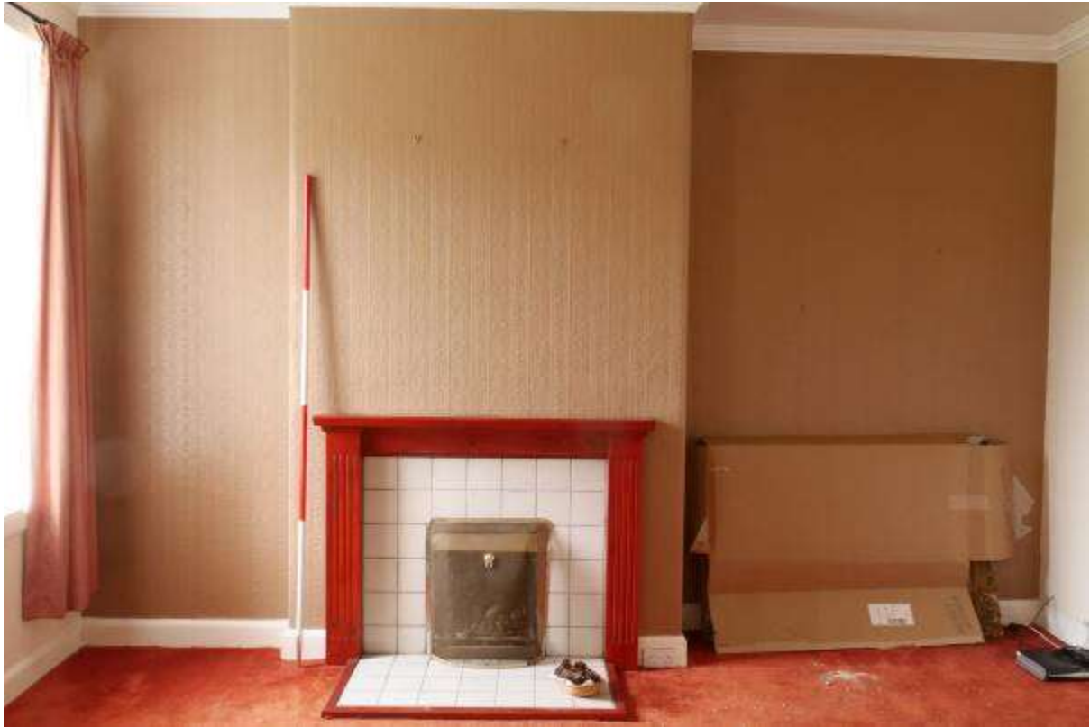
Illustration 50- South Eastern facing internal elevation of Room 4 showing fireplace. It is proposed to make alterations to the fireplace.
