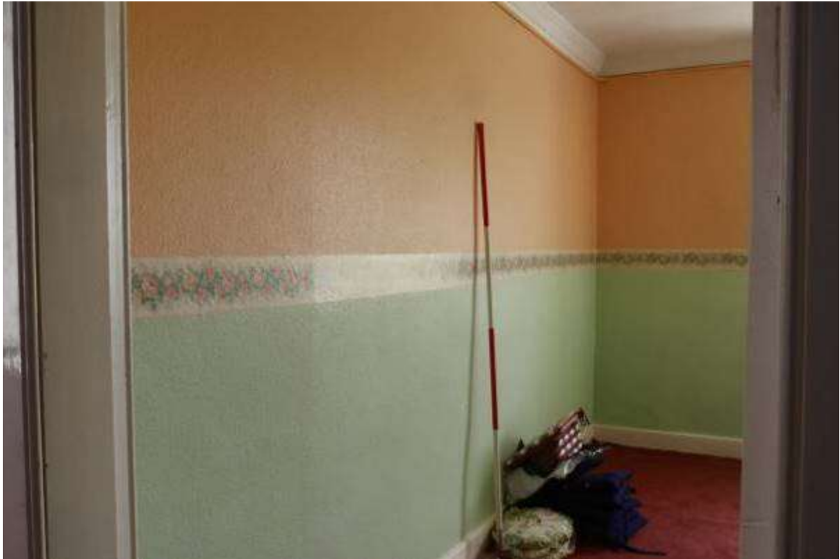
Illustration 60- Internal North Western elevation of Room 6 (Bedroom). It is proposed to make alterations to this elevation.
