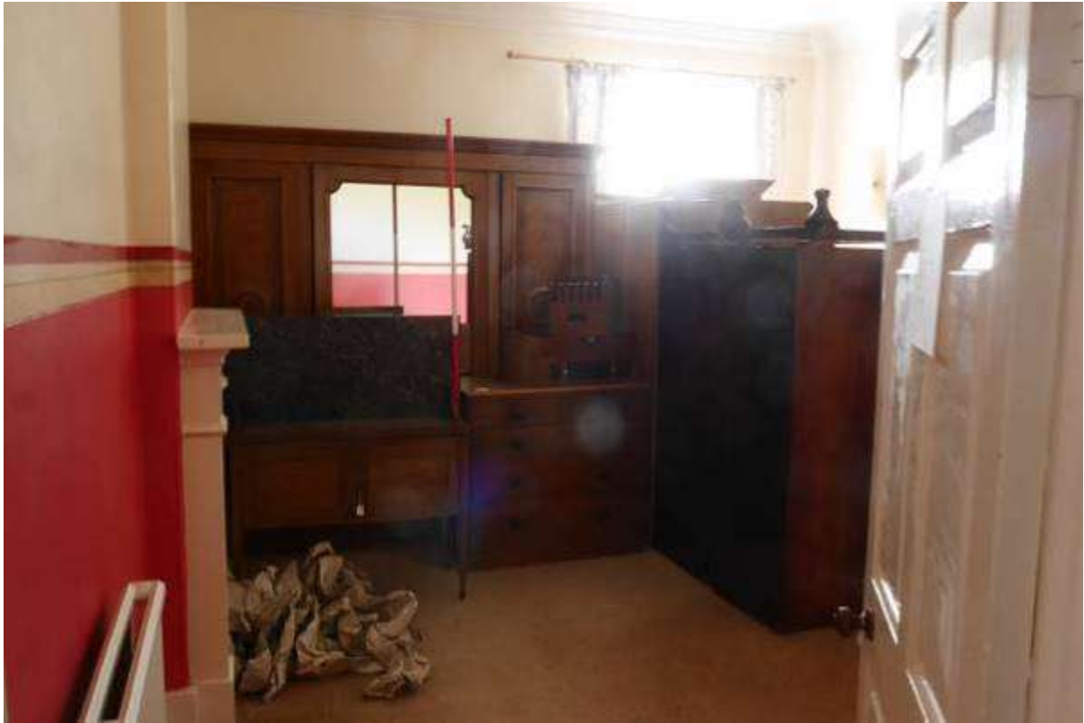
Illustration 61- Internal North Eastern elevation of Room 7 (Bedroom). It is proposed to make alterations to this elevation, to form a new opening out to the new west extension window.
