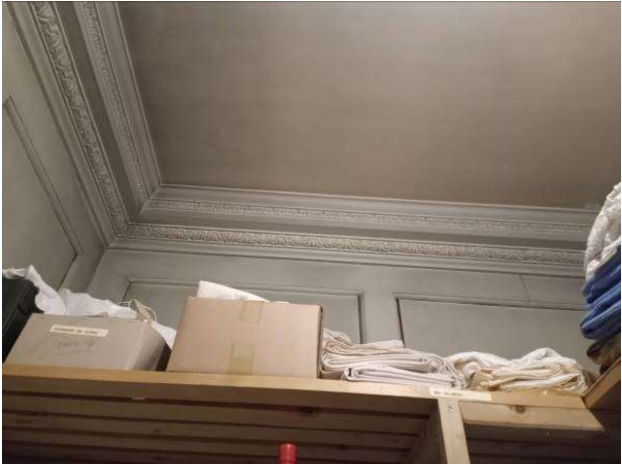
Illustration 112- Linen Cupboard 24 detail of mouldings along ceiling edge and wooden panelled walls on North Western facing internal elevation (wall to be removed).
