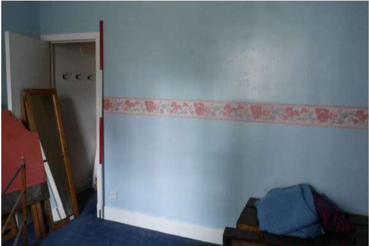
Illustration 68- Internal North Eastern elevation of Room 8 showing cupboard. It is proposed to remove this wall.
