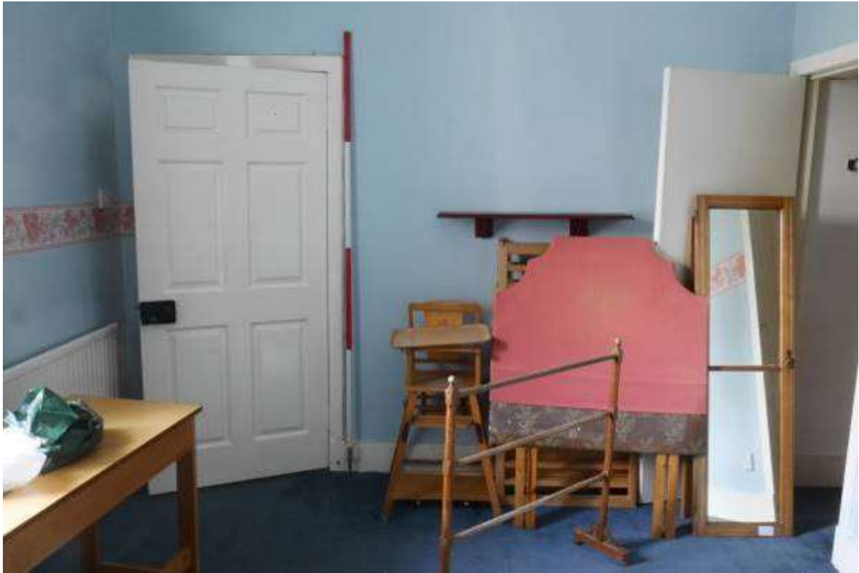
Illustration 69- Internal North Western elevation of Room 8 showing door into South Corridor (3). It is proposed to make alterations to this elevation, the wall and cupboard on the right are removed and the space re-combined with the Study beyond (West).
