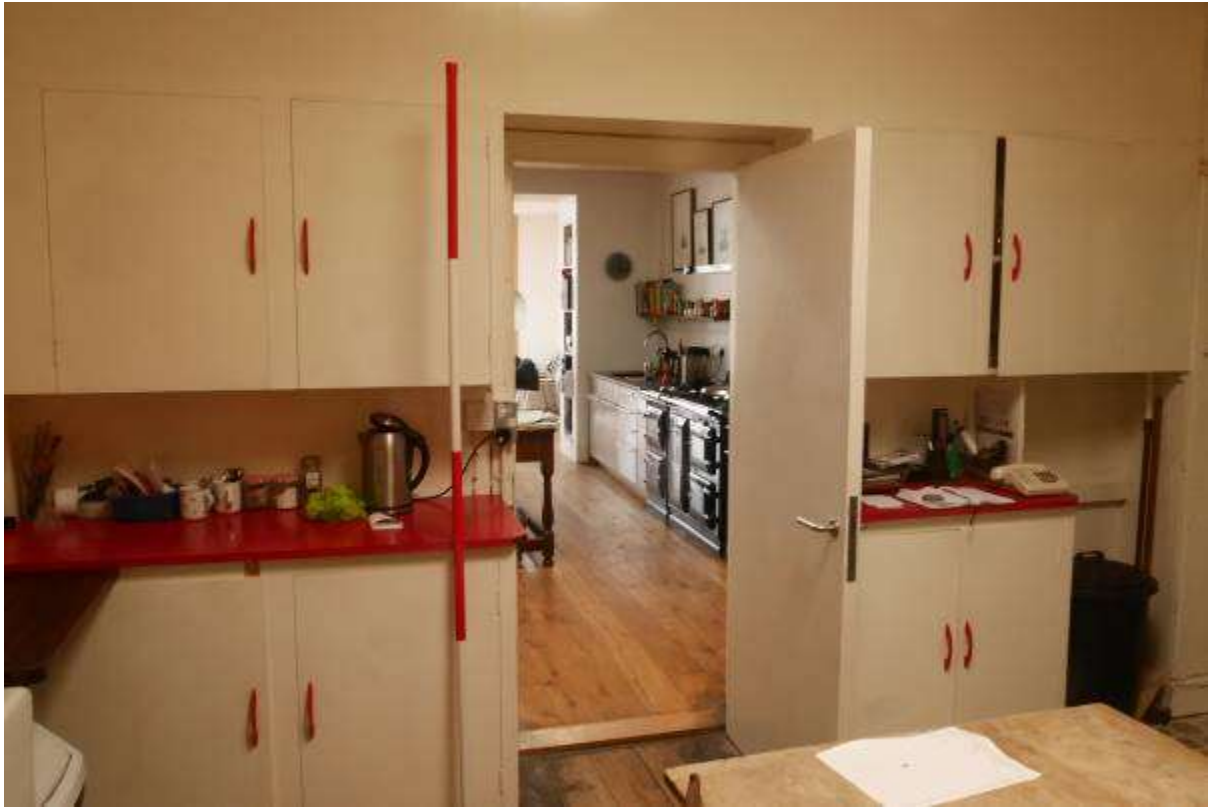
Illustration 89- North Western facing internal elevation of Room 15 (Pantry). It is proposed to remove all the furniture.
