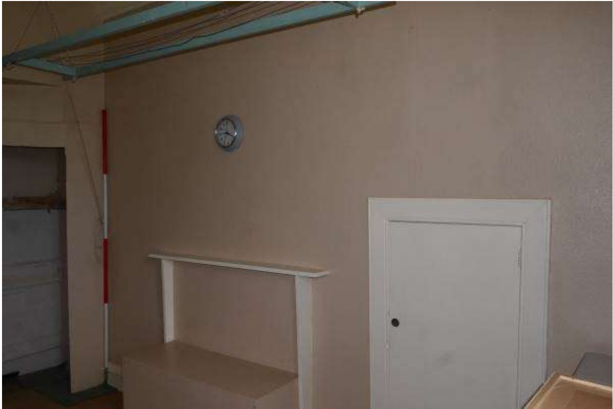
Illustration 56- Internal North Western facing elevation of Room 5 (Kitchen) showing blocked fireplace and cupboard. It is proposed to remove the fireplace.
