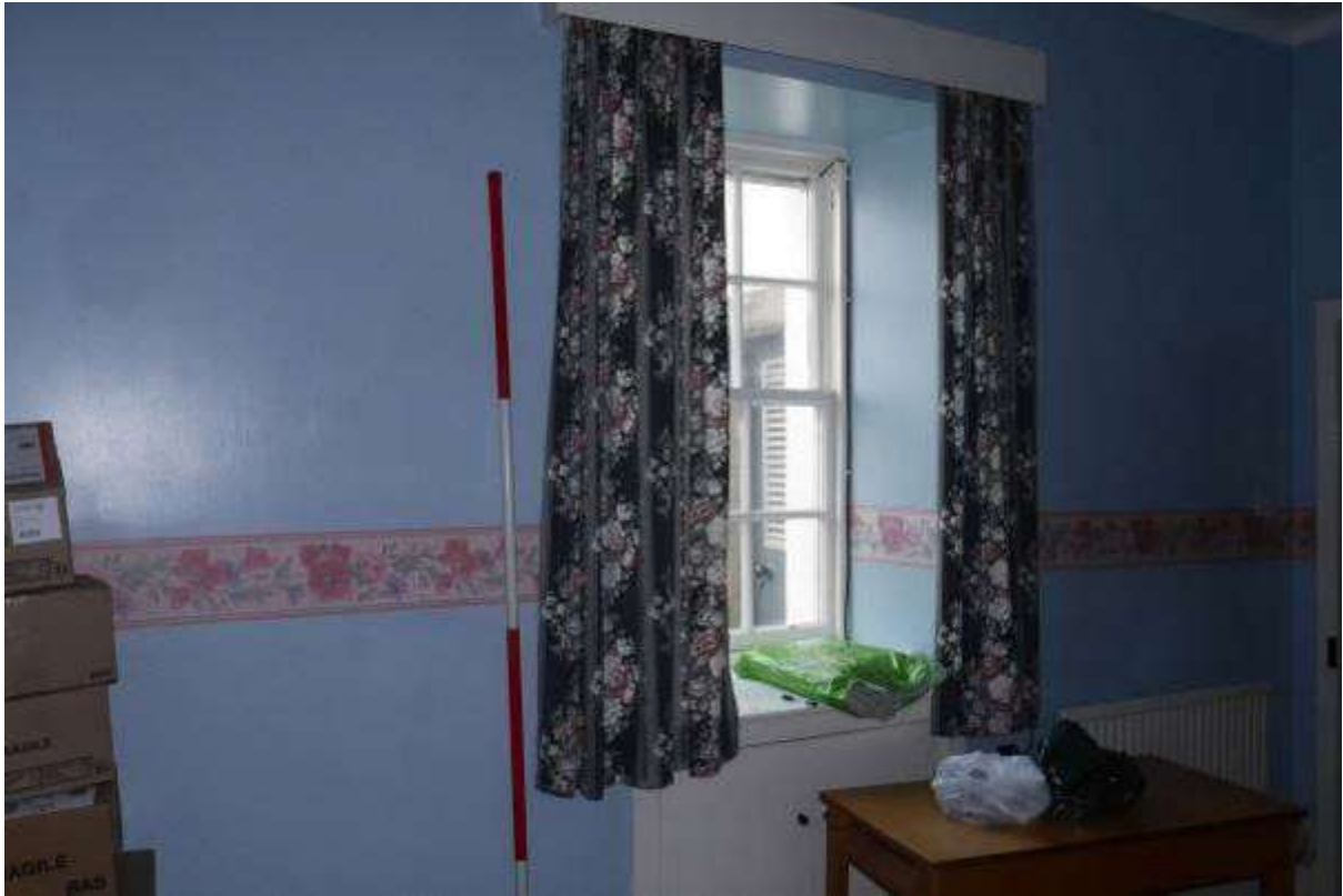
Illustration 65- Internal South Western facing elevation of Room 8. It is proposed to make alterations to this elevation, the sill of the window will be lowered to form a new window into the new corridor beyond.
