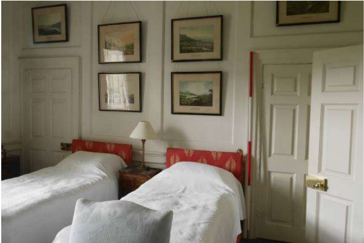
Illustration 101- Bedroom 21 South Eastern facing internal elevation showing wooden panelling and double doors. The door on left is to be blocked, and the one on the right will provide access to a new shower space.
