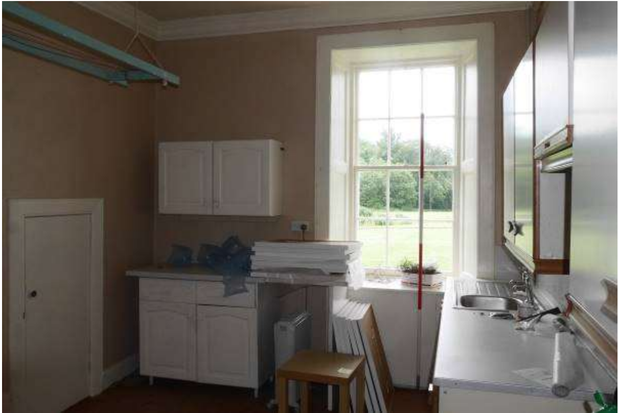
Illustration 53- Internal North Eastern facing elevation of Room 5 (Kitchen). It is proposed to make alterations to this elevation.
