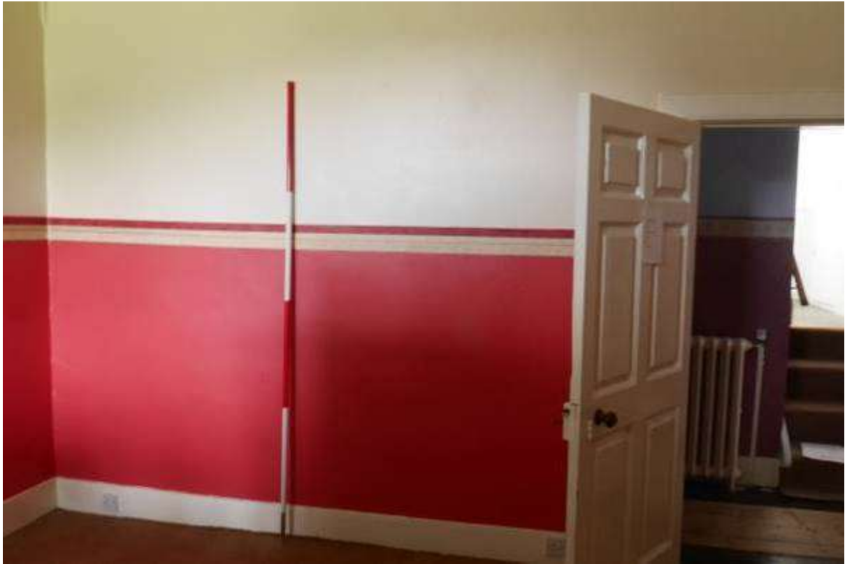
Illustration 63- Internal South Western elevation of Room 7. It is proposed to make alterations to this elevation, it is proposed to remove this wall and doorway below door head level.
