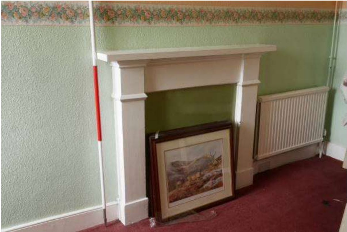
Illustration 58- Internal South eastern facing elevation of Room 6 (Bedroom) showing fireplace. It is proposed to remove part of this wall and the fireplace.
