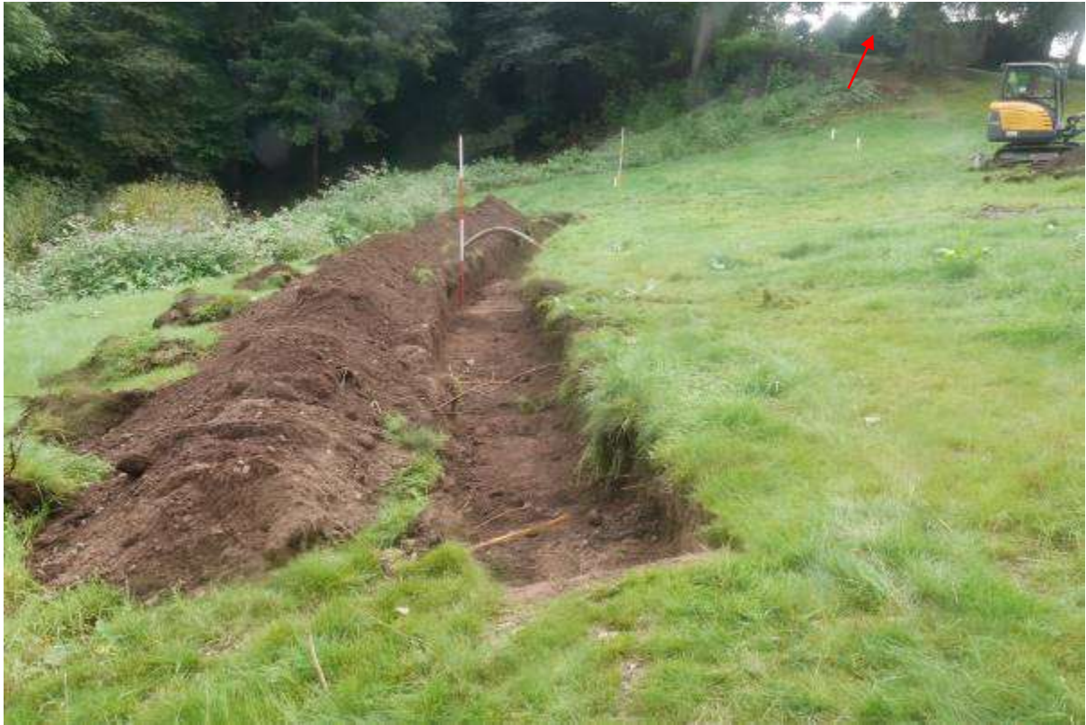
Illustration 6- Trench A in process of excavation looking South East, Forgandenny churchyard is just visible behind the trees at the top of the photograph (red arrow).
