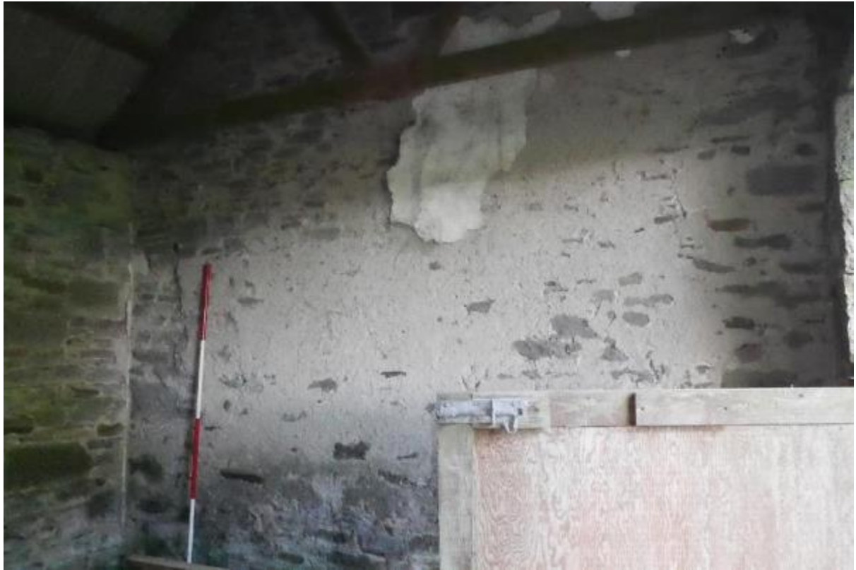
Illustration 16- Internal South Eastern facing elevation of North Western room of Building A.
