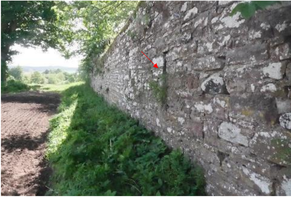
Illustration 56- External North Western facing elevation of Boundary wall C, red arrow shows location of slit window.
