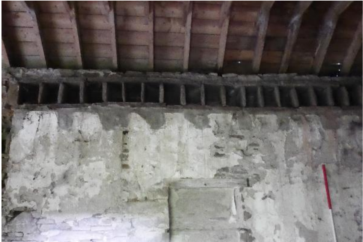
Illustration 40– Detail view of 21 bird boxes at roof line in internal South Eastern facing elevation of Building B. The interior of the wooden roof supporting the slates is also visible.
