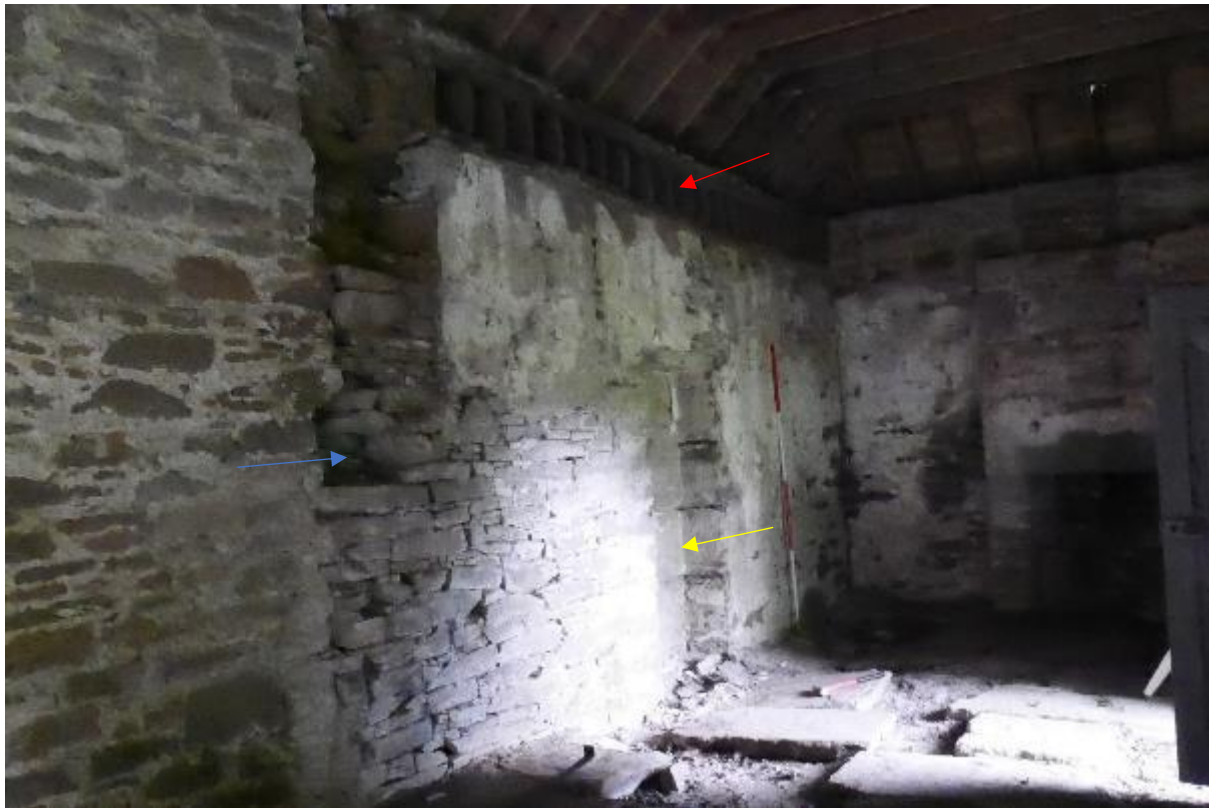
Illustration 38 – Northern half of internal South Eastern facing elevation of Building B, bird boxes shown at the red arrow, former wall line of earlier building at blue arrow. Blocked doorway at yellow arrow.
